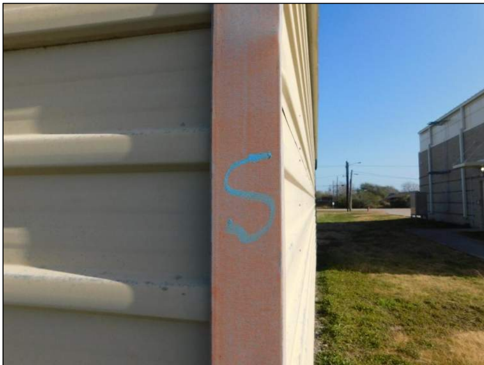
Photo 93: No hail spatters on south wall.
