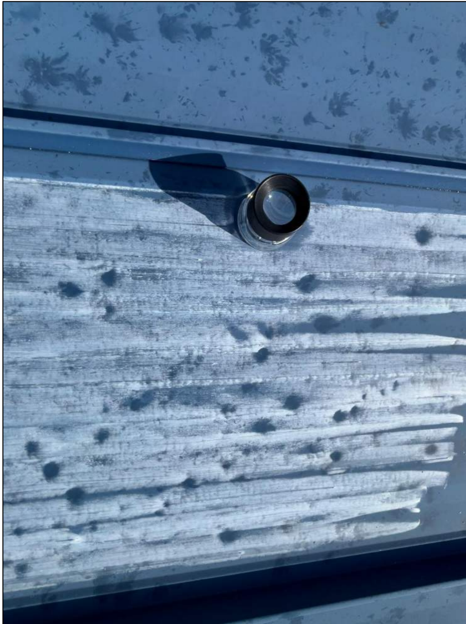
Photo 15: Magnifier inspection was conducted on the largest hail spatters.
