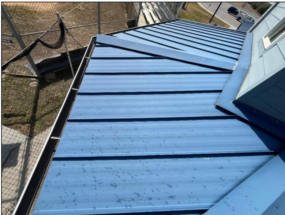
Photo 26: Significantly less hail spatters on east-facing apron slopes.
