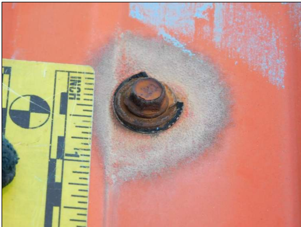
Photo 45: Close-up of fastener corrosion and gasket deterioration due to aging.
