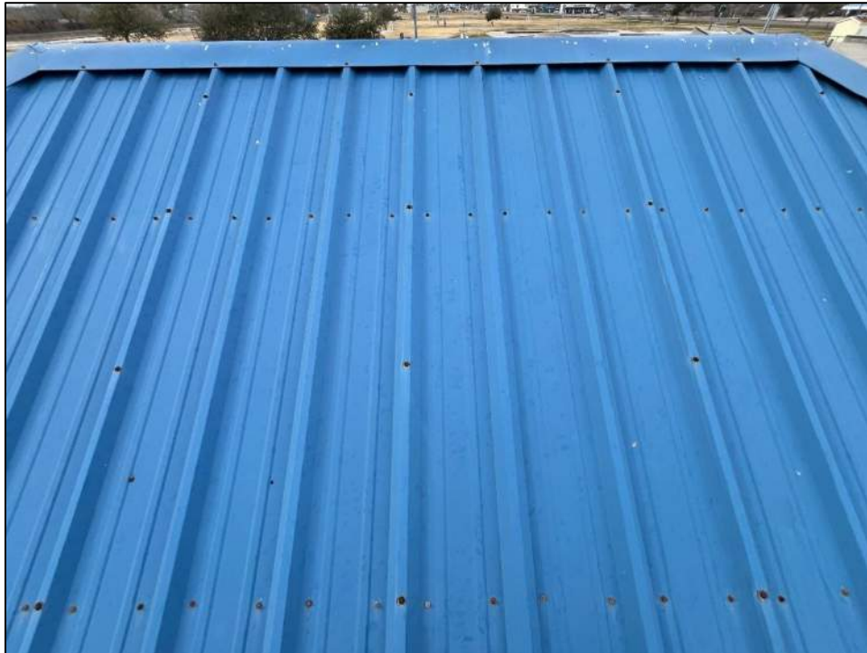
Photo 66: East slope overview. Note corroded fasteners throughout the slope.
