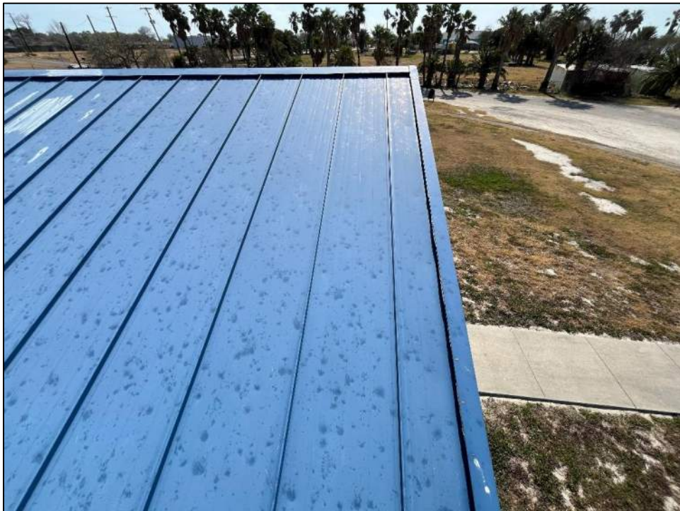
Photo 10: Widespread hail spatters on north slope.
