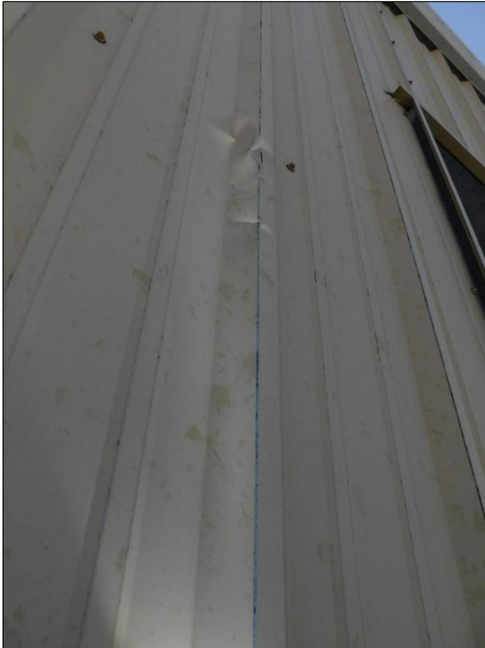
Photo 9: Crumpled wall ribs at the upper portion of west wall that were inconsistent with hail impact.
