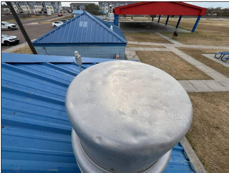
Photo 69: Dented vent hood consistent with hail impact.
