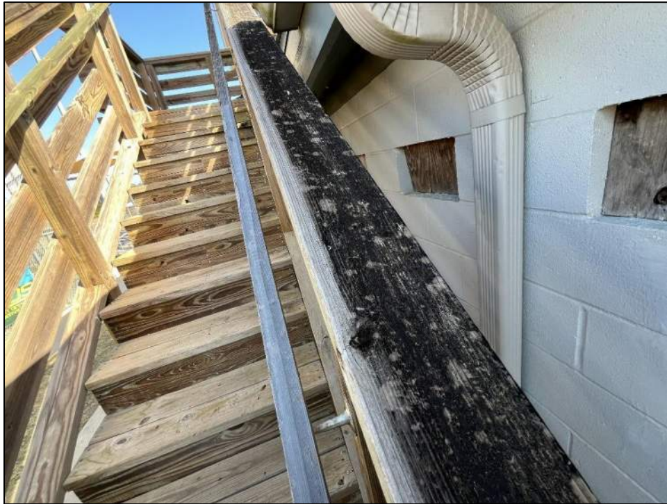
Photo 9: Close-up of hail spatters on algae covered wooden hand rails.
