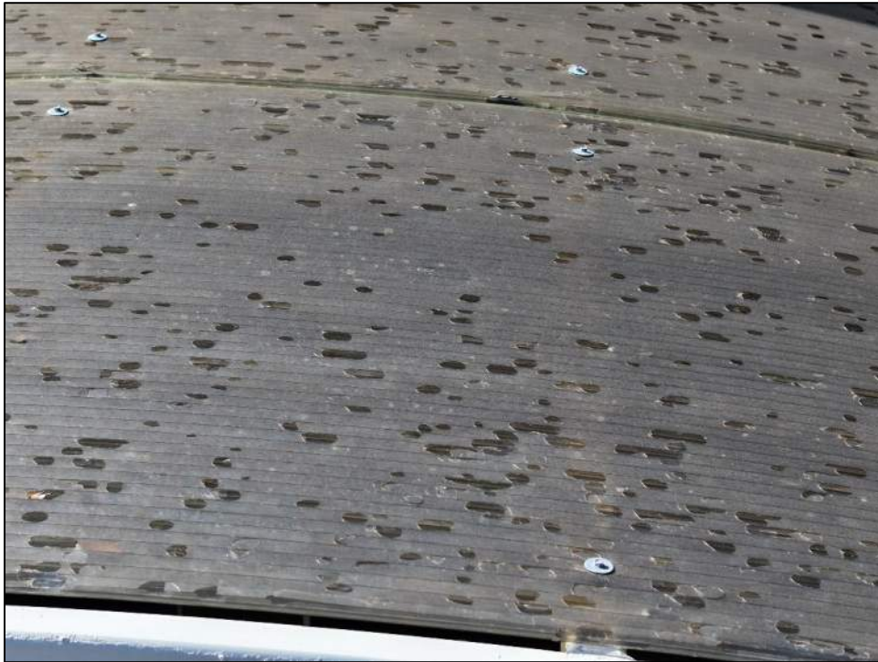
Photo 47: Close-up of the hail punctures to the polycarbonate canopy above the police station front entry.
