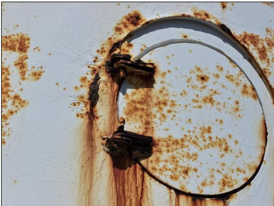
Photo 26: Close-up of the severely corroded side door and hinges.
