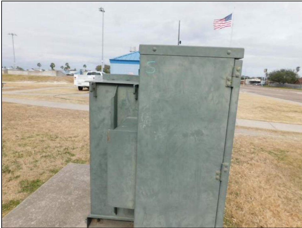
Photo 25: No hail spatter on south-facing surface of nearby electrical cabinets.
