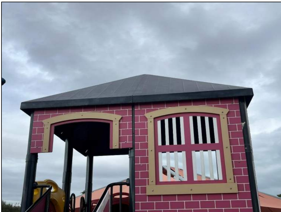
Photo 114: Side view of the playset with a steel plate roof.
