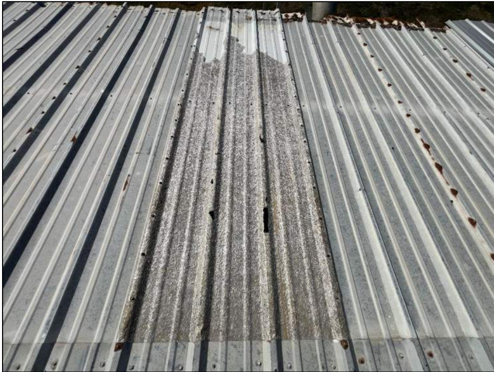
Photo 29: Additional view of the deteriorated skylight panels with large rib fractures that were both consistent and inconsistent with hail impact.
