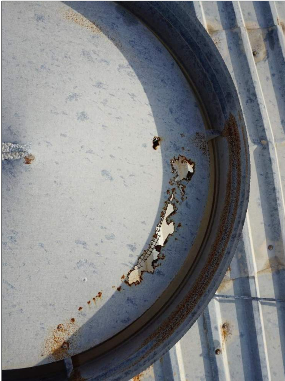
Photo 54: Rusting through of other remaining ridge vent covers.
