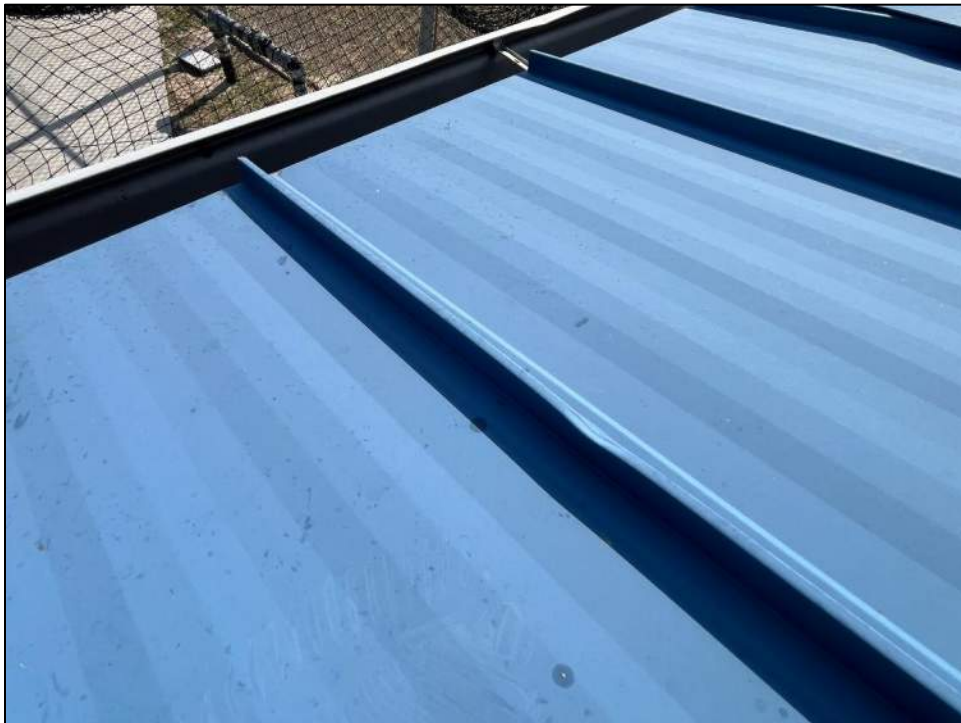
Photo 28: Deformed seam absent of hail impact.
