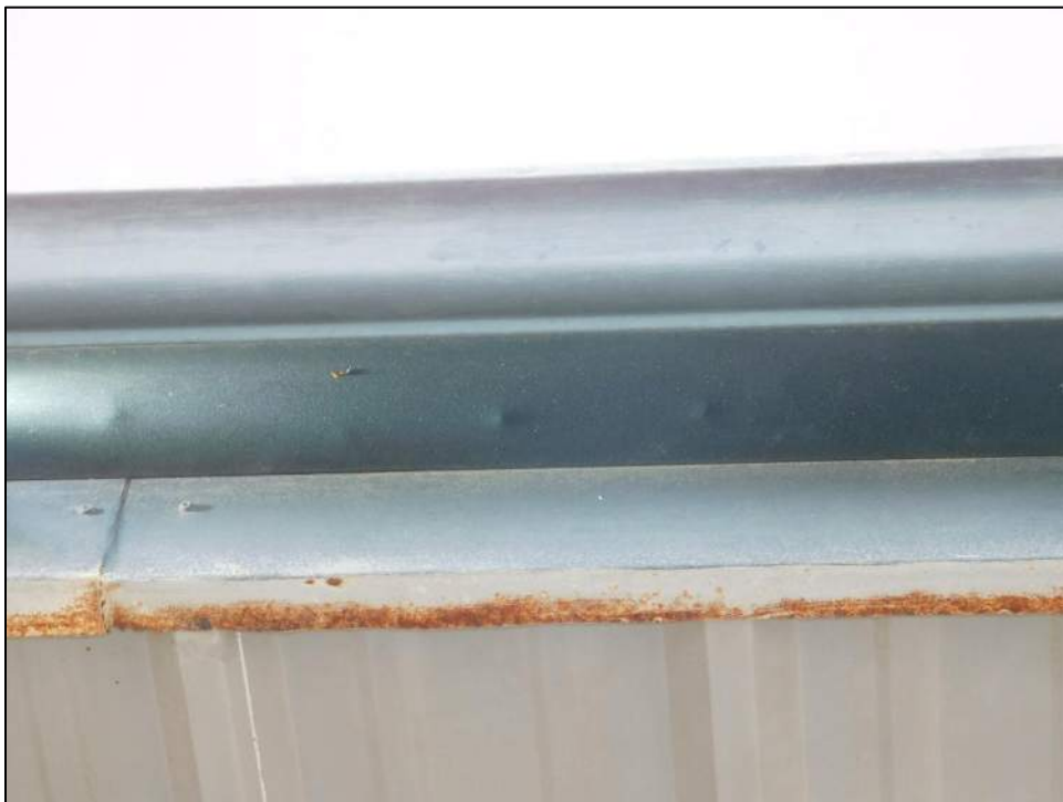
Photo 22: Dented gutter bottom (front elevation) consistent with hail impact.
