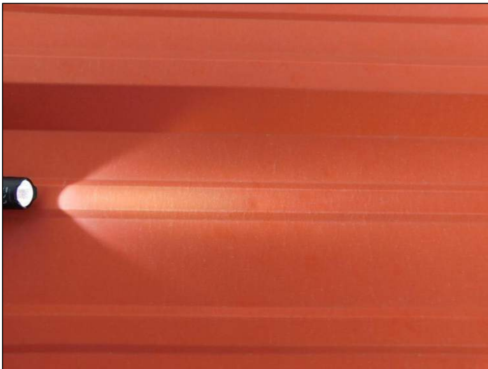
Photo 35: Slight denting on west slope consistent with hail impact.
