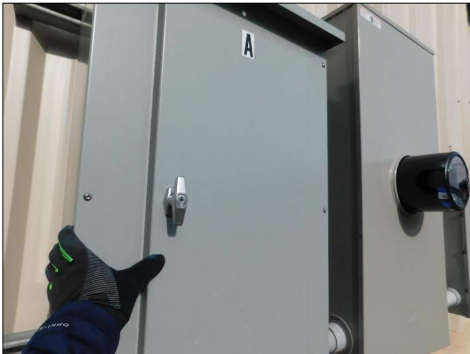
Photo 6: No hail spatters were observed on the electrical panels.
