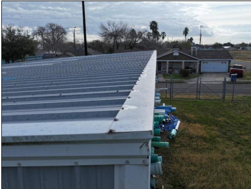
Photo 11: Front closure metal remained securely fastened.
