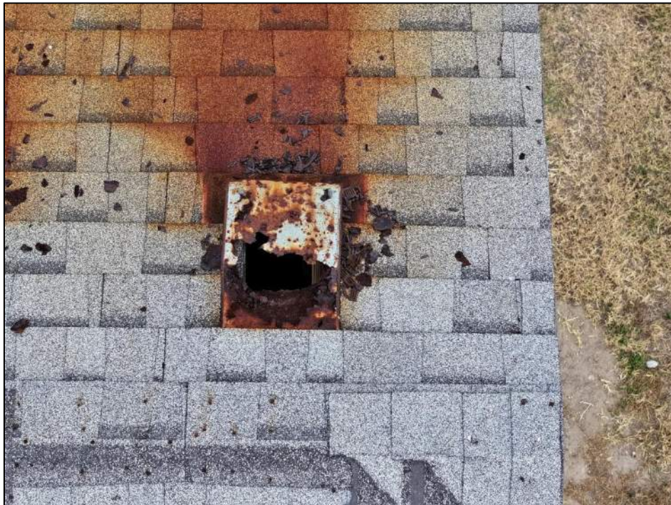
Photo 8: Deteriorated ridge vents.
