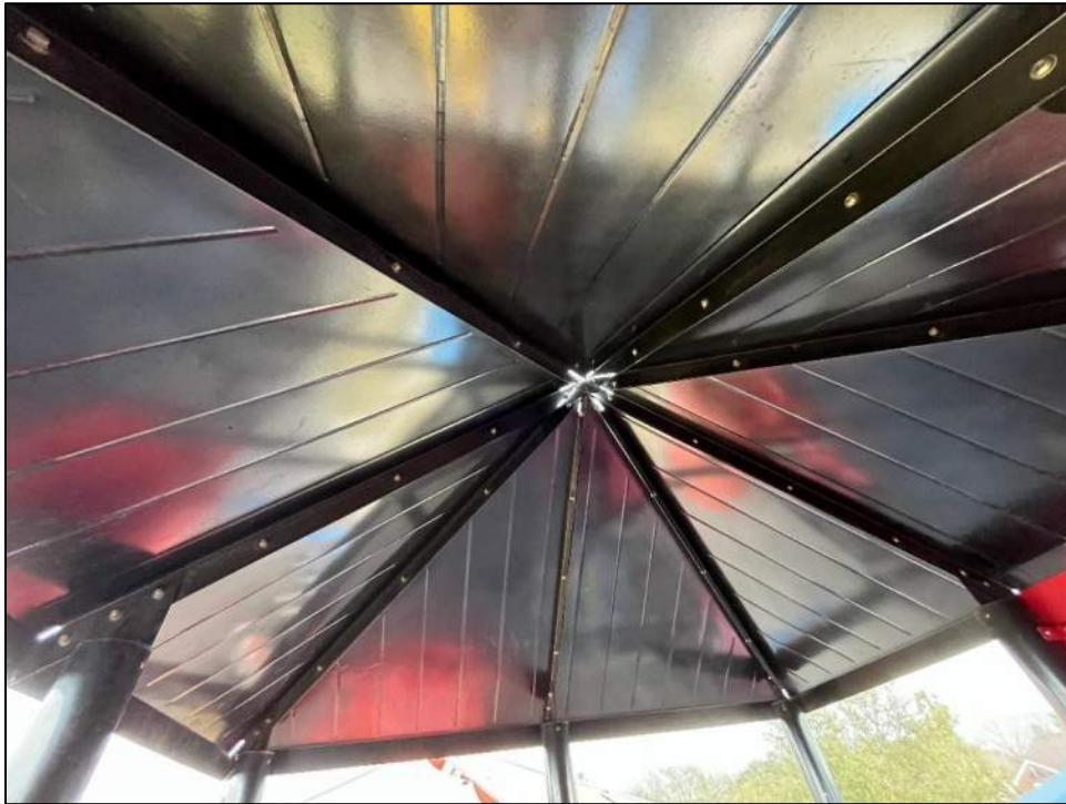
Photo 115: Underside of the metal plate roof were absent of any hail impact indentations.
