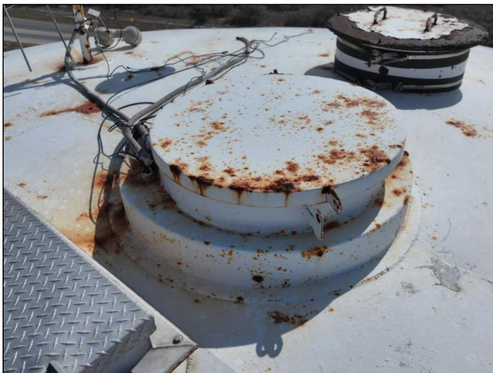
Photo 24: Steel plate vent coverings remained structurally intact. Wiring remained undisturbed.
