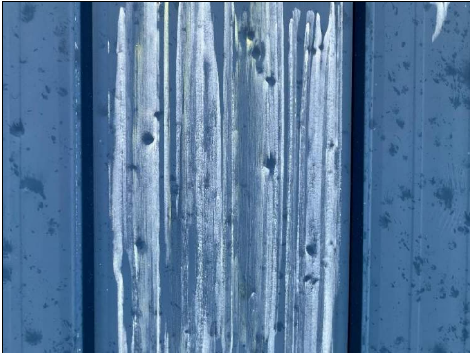
Photo 13: Hail denting on north slope had inner diameter of up to 5/8 inch.
