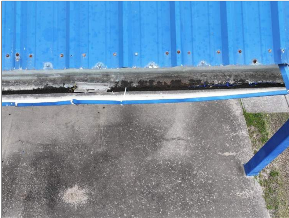
Photo 52: Mechanical damage to gutter along north slope eave.
