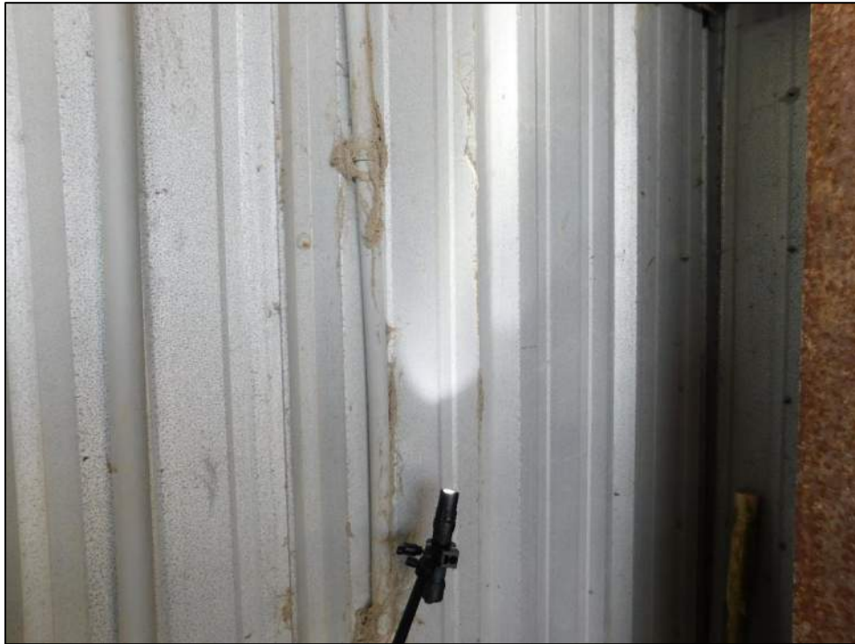
Photo 87: No denting observed on the north or west wall (interior surfaces).
