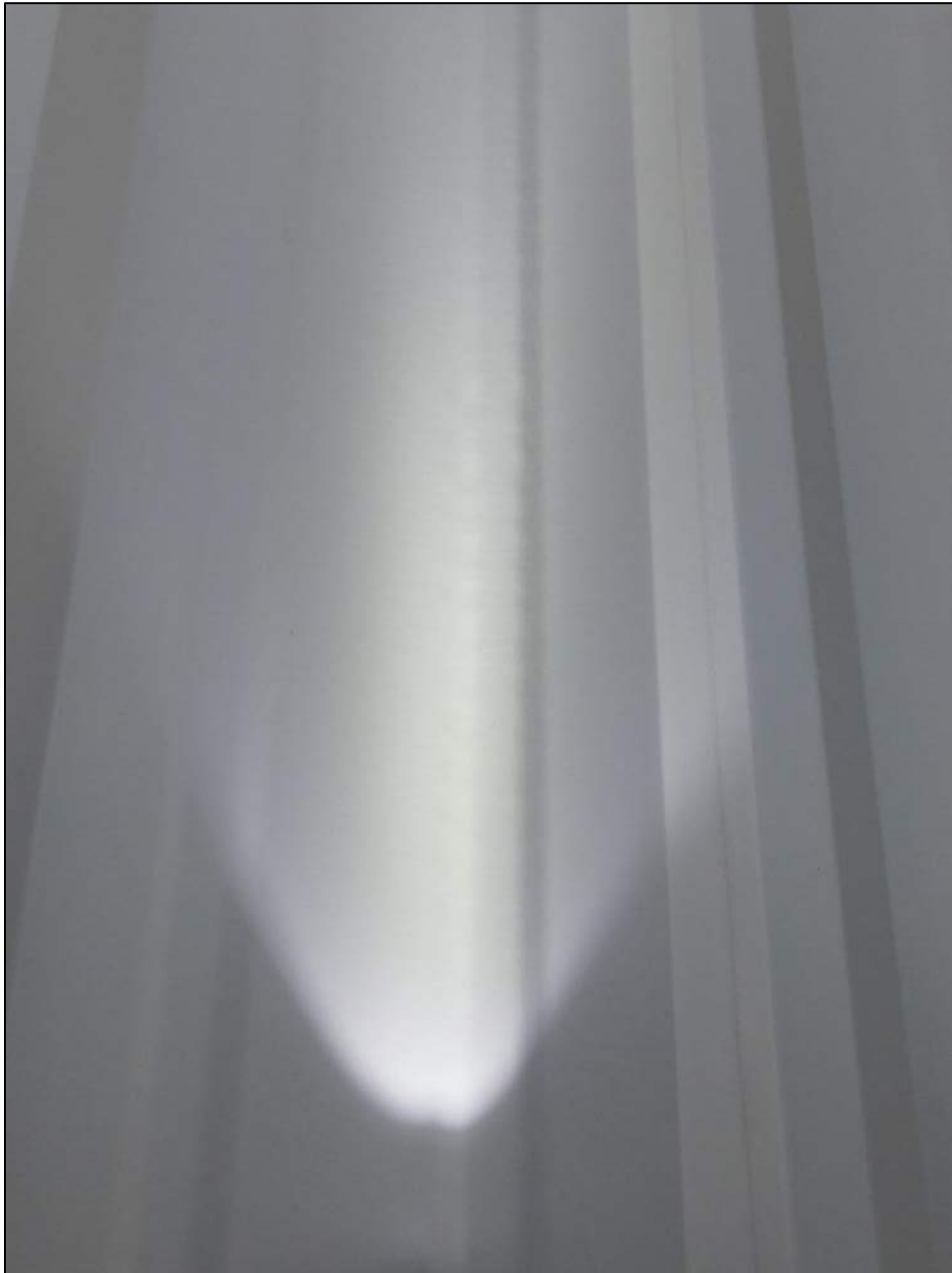
Photo 11: Isolated slight denting was observed on the west wall panels under directional lighting.
