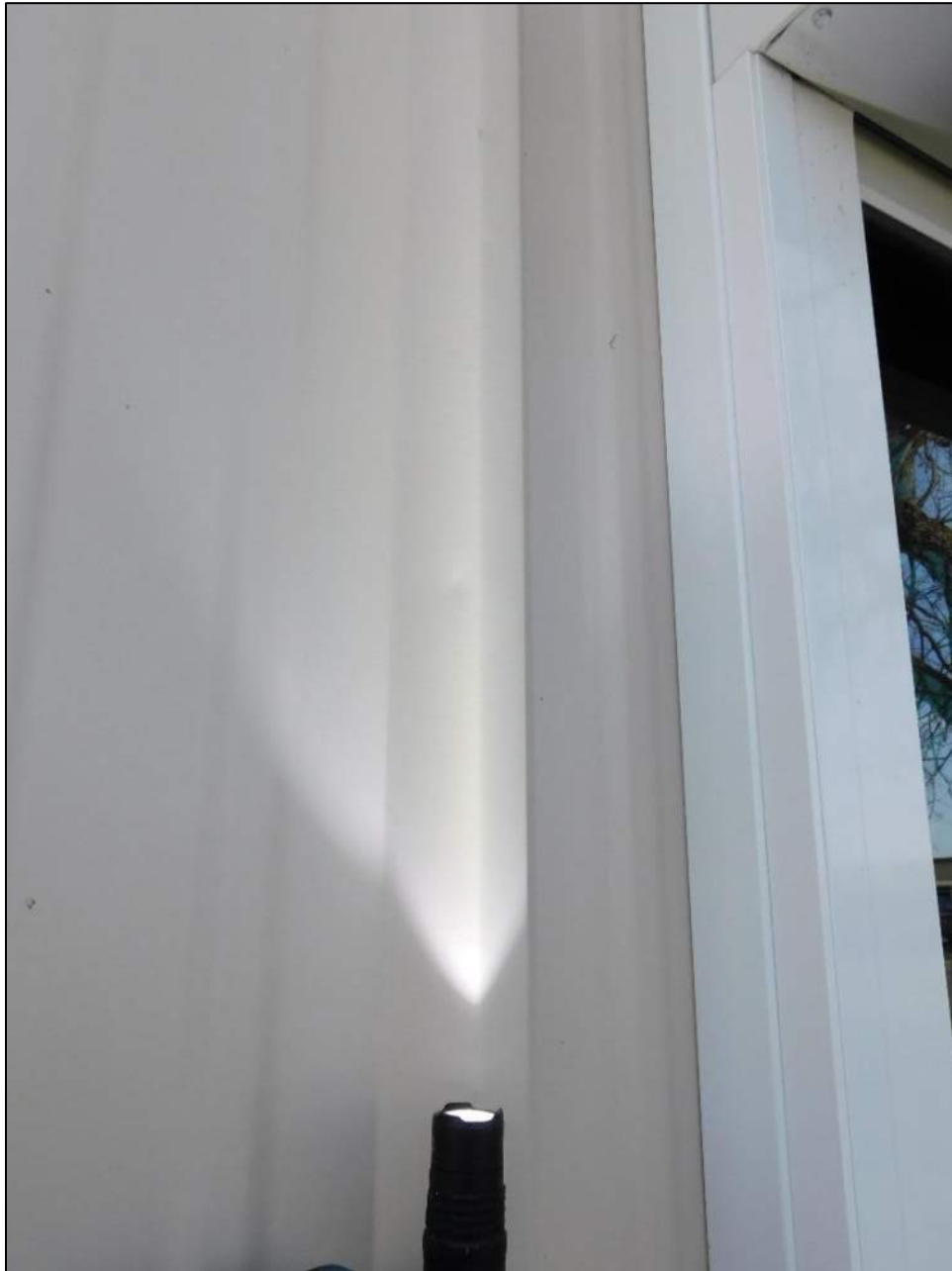
Photo 12: Isolated slight denting was observed on the west wall panels under directional lighting.
