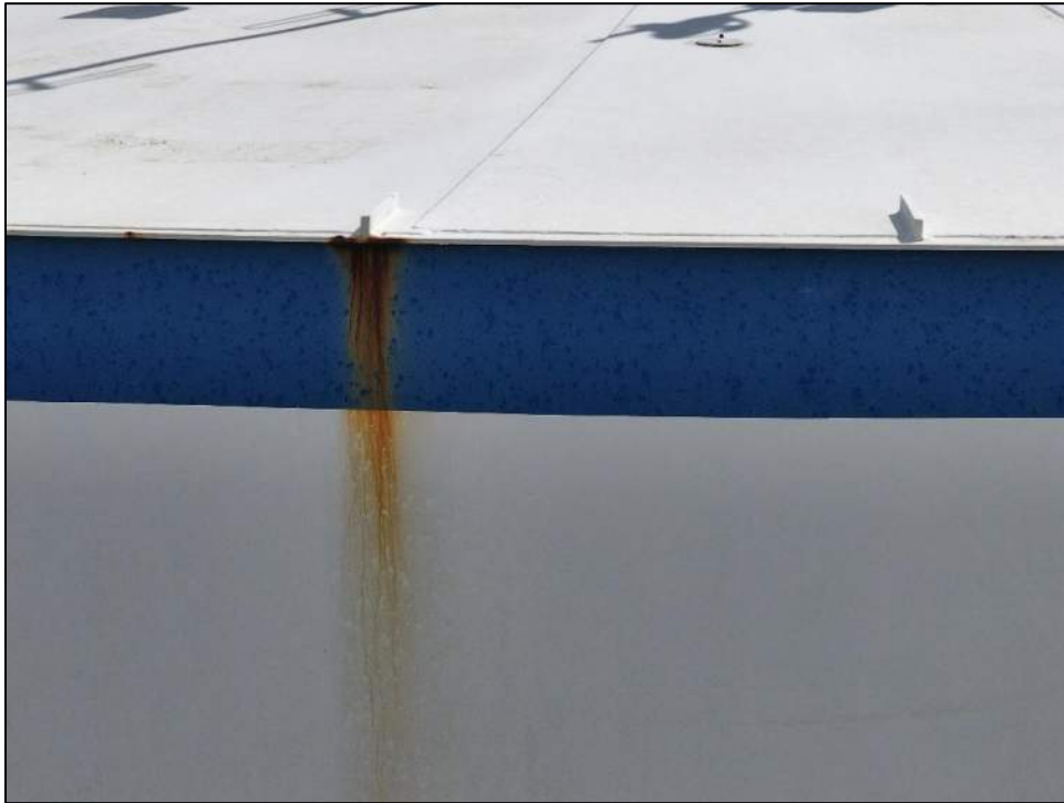
Photo 5: Hail spatter on tank wall and steel corrosion.
