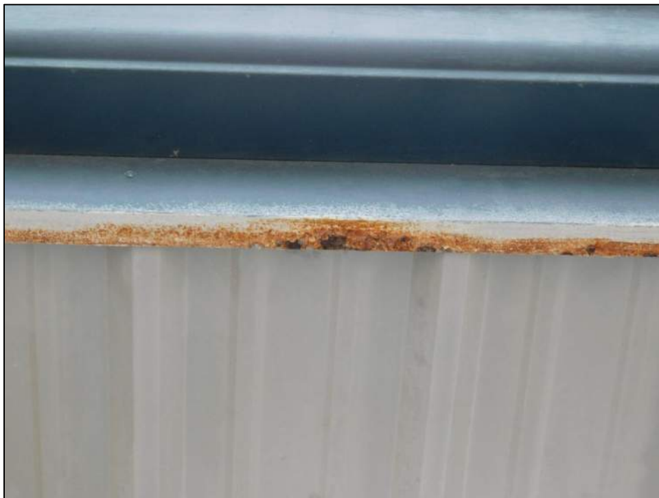
Photo 18: Front fascia corrosion.
