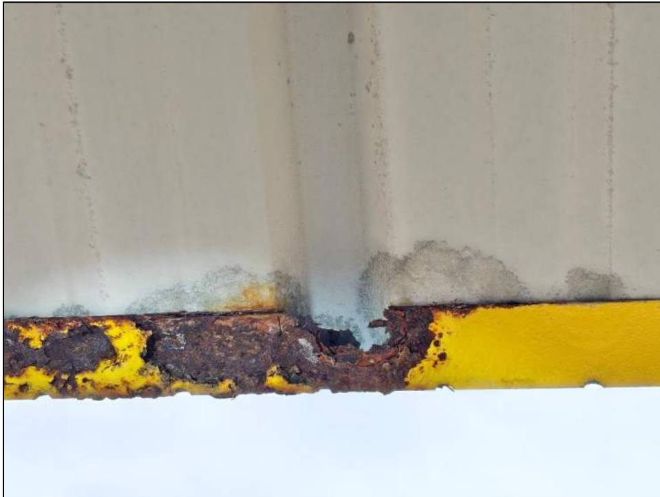
Photo 93: Typical closure metal corrosion along roof eaves.
