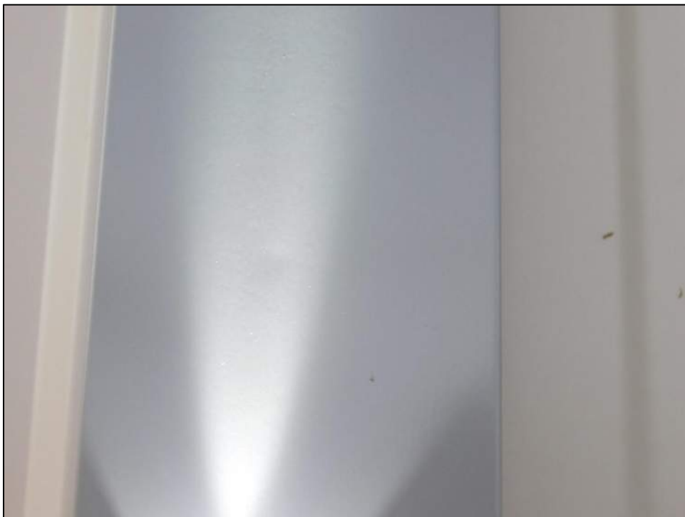
Photo 17: No coating disruptions were observed on the hail denting on the rear gutter downspout.
