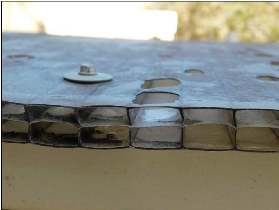
Photo 48: Close-up of the hail puncturing of the polycarbonate canopy above the police station front entry.
