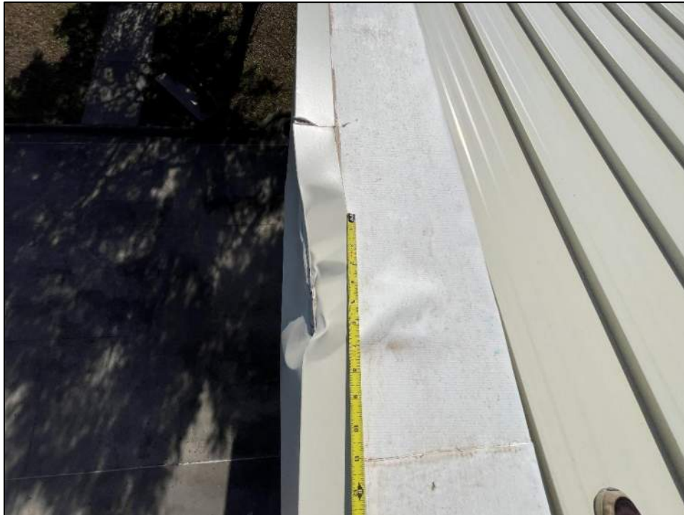
Photo 72: Mechanical denting to the north rake edge of the fire department roof that was inconsistent with hail impact.
