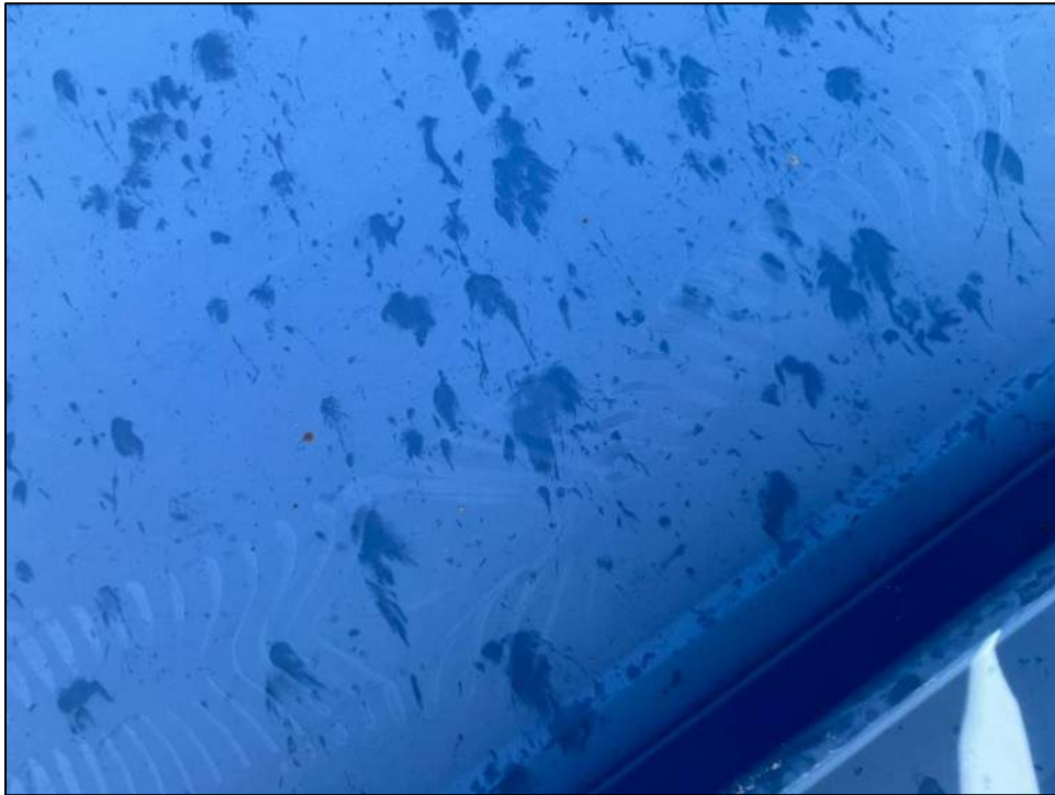
Photo 33: Close-up of hail spatters on high roof.
