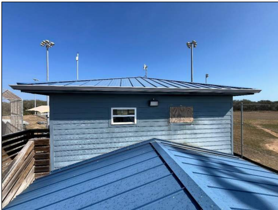
Photo 10: Coated Standing seam metal roof panels exhibited spatters and denting on all primary slopes.
