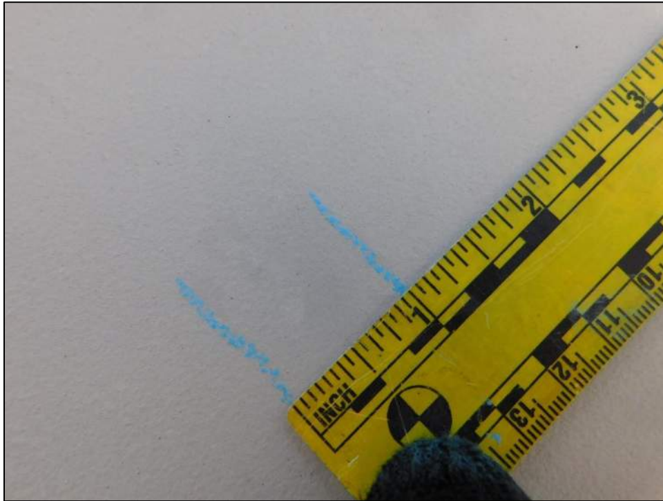
Photo 15: Hail spatters on west walls reflected maximum of 1-inch hail.
