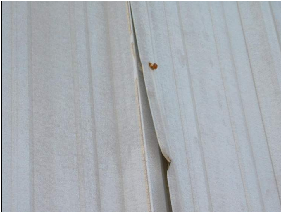
Photo 81: Corroded fastener mechanical damage on the north wall.
