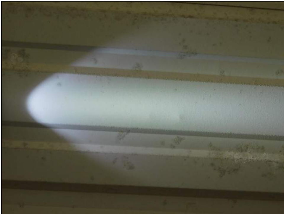
Photo 46: Denting on the underside of the carport metal roof panels consistent with hail impact.
