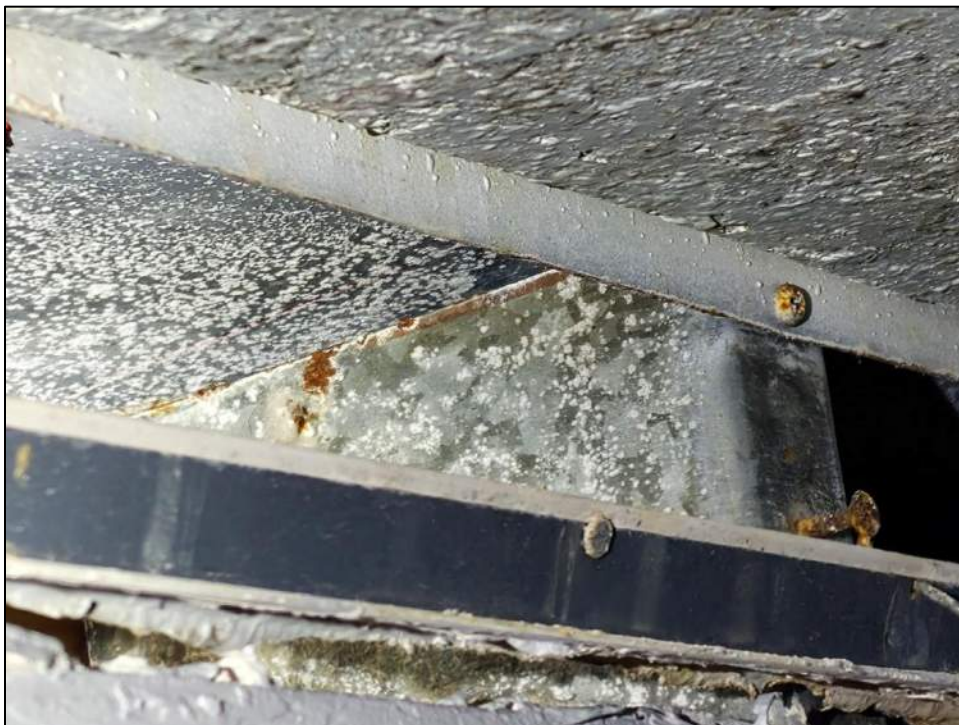
Photo 38: Wall stucco corresponding to a wall offset on the exterior were corroded. Note the rusted wall screw.
