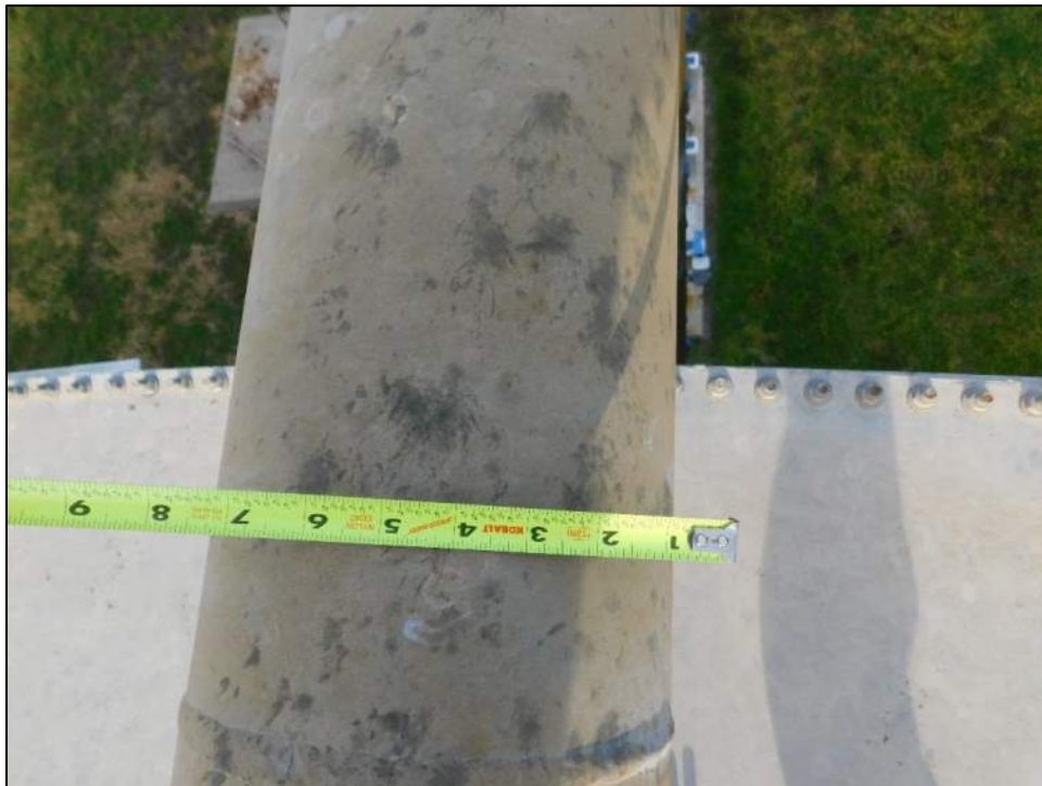
Photo 74: Hail spatter on tank rooftop piping reflective of 1.5 inch hail.
