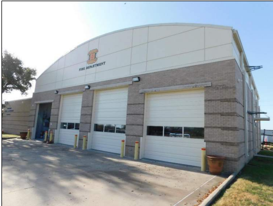
Photo 35: Front wall of the fire department had 4 roll-up doors that exhibited slight denting consistent with hail impact.
