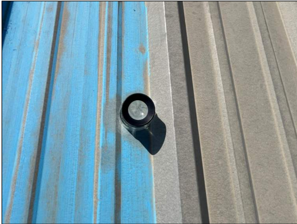
Photo 71: No coating disruptions were observed at the hail dents on the roof deck.
