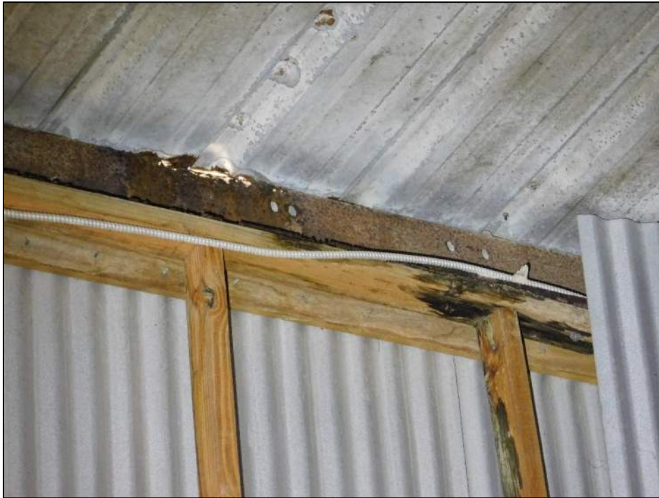
Photo 100: Corroded roof deck above the east wall in the enclosed storage room at the south end of the vehicle storage building.
