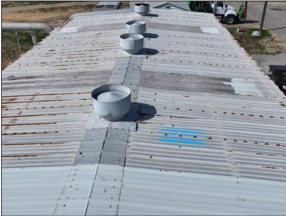
Photo 18: Roof overview. Note widespread corrosion deteriorated skylight panels (partially underlaid with metal panels) and panel overlays.
