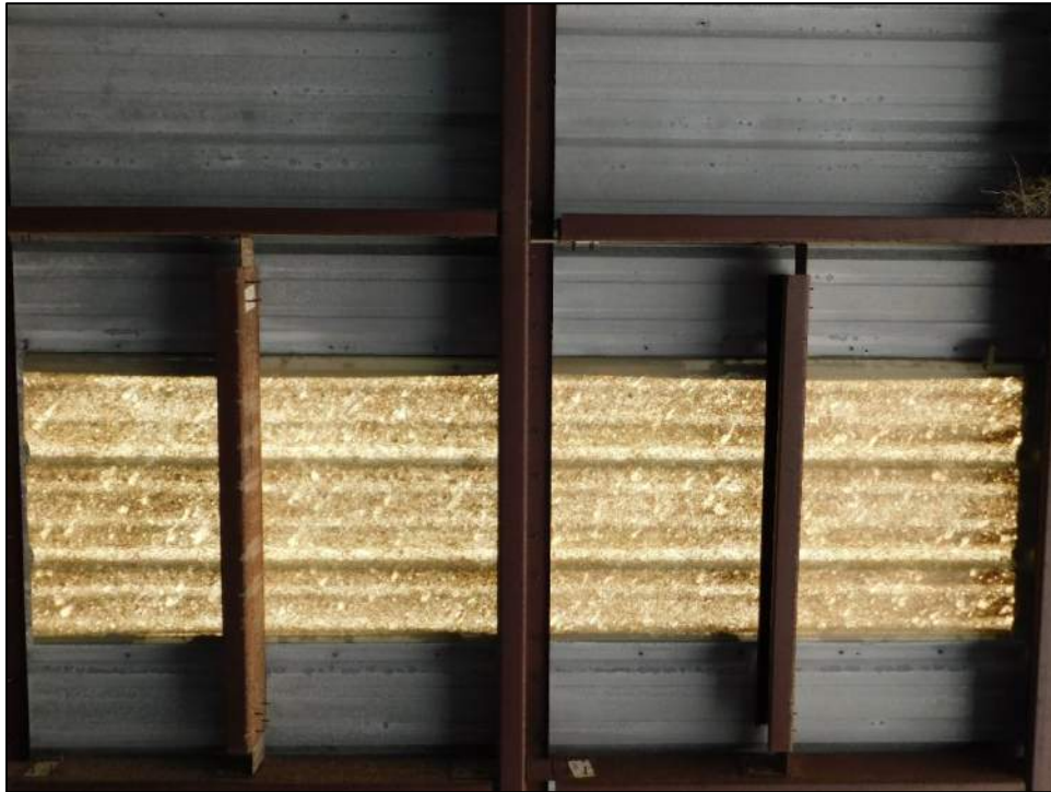
Photo 102: Skylight of the vehicle storage building were not fractured.
