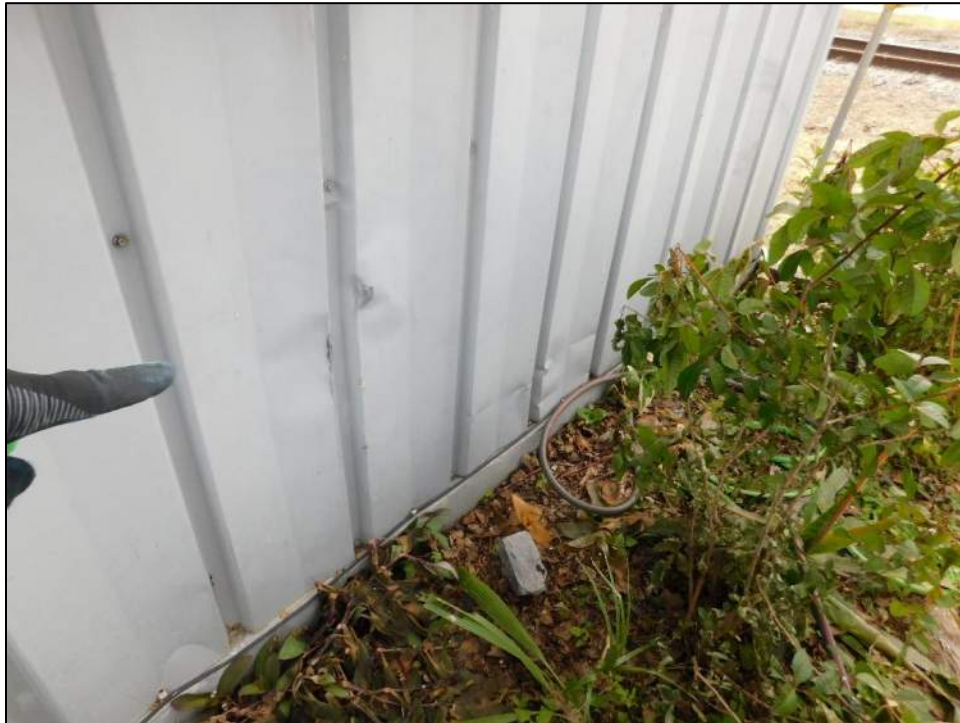
Photo 19: Mechanical damage at the lower section of the west wall.
