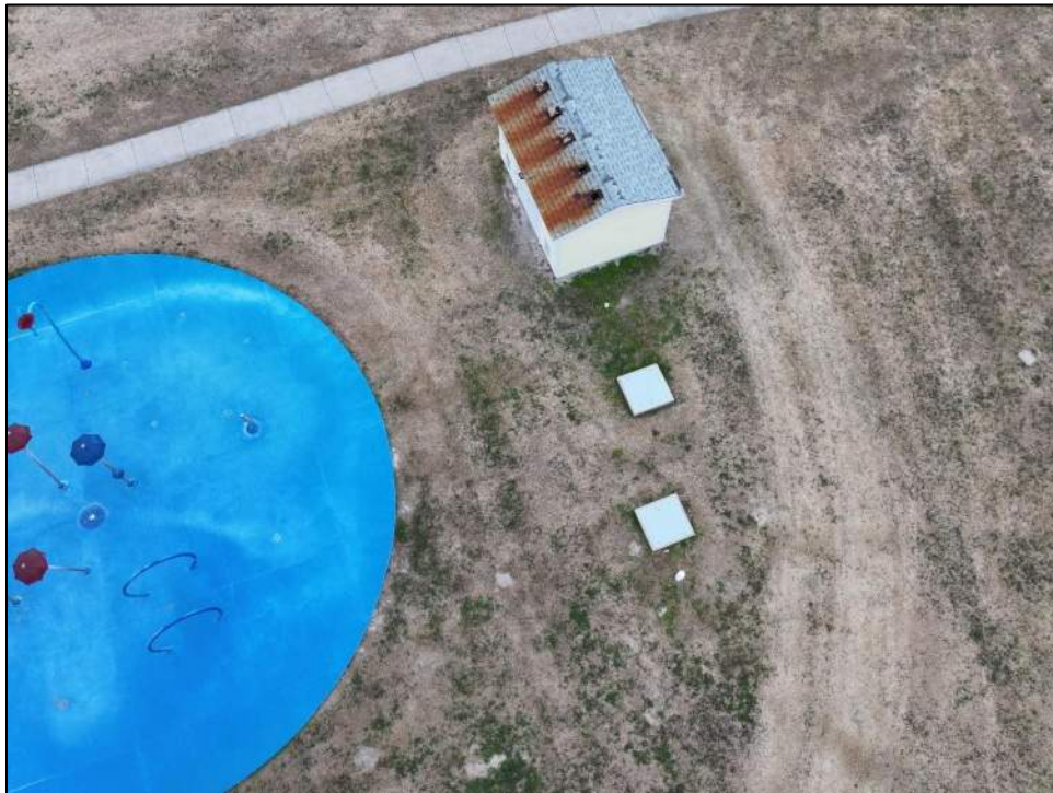
Photo 6: Deteriorated tool shed west of the splashpad.
