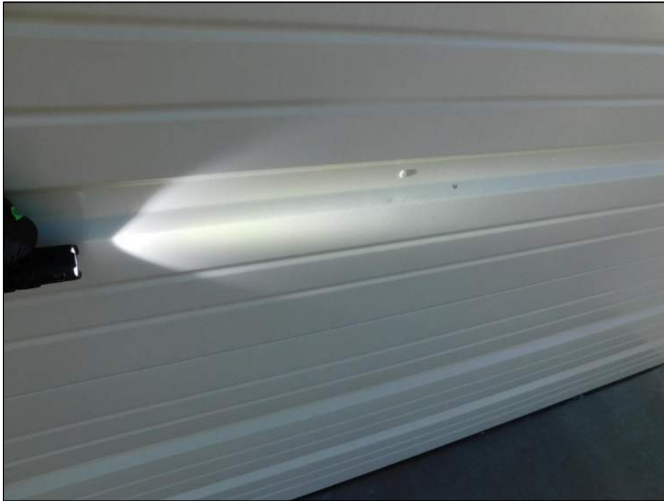
Photo 37: Slight denting on roll-up doors.
