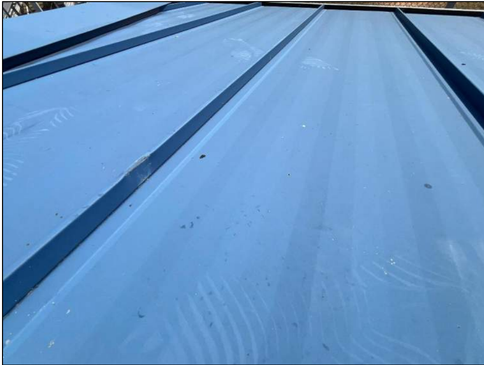
Photo 29: Scrapes caused localized coating damage and surface rusting.
