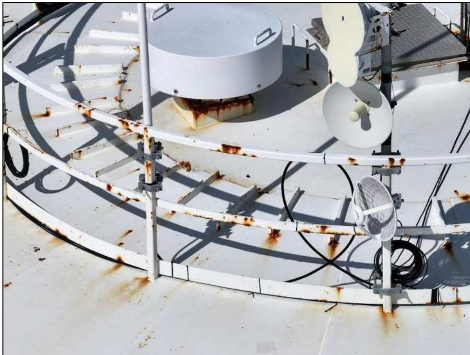
Photo 3: Typical corrosion of railing at rooftop.
