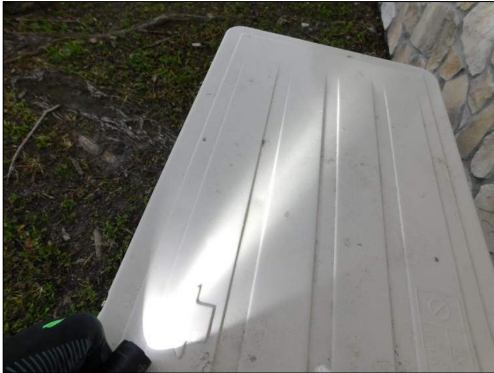
Photo 7: Hail denting was observed on the top surface of the split AC unit on the west side of the building.
