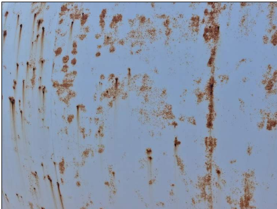
Photo 14: Close-up of typical rusting.
