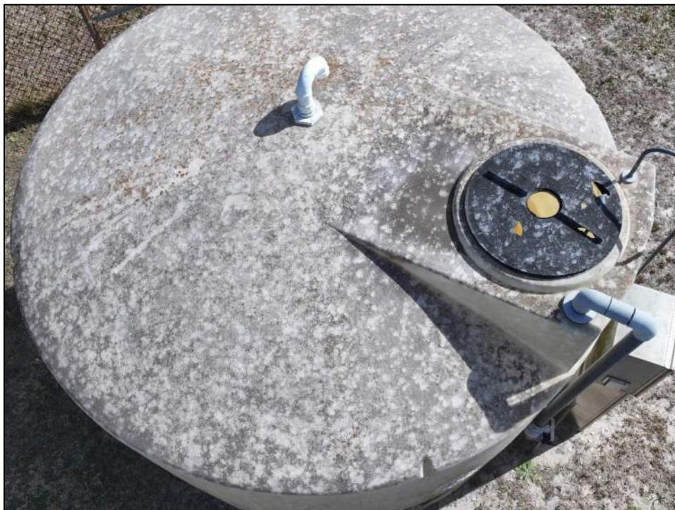
Photo 6: Hail spatters on nearby vinyl water tank consistent with 1.0- to 1.5-inch hail.
