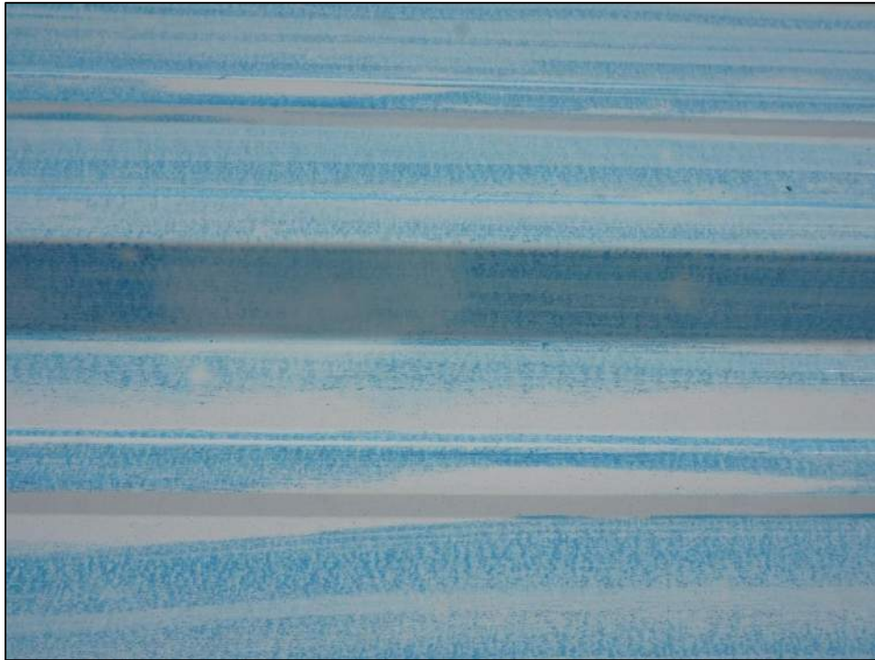
Photo 29: No coating disruptions were observed at the hail dents.
