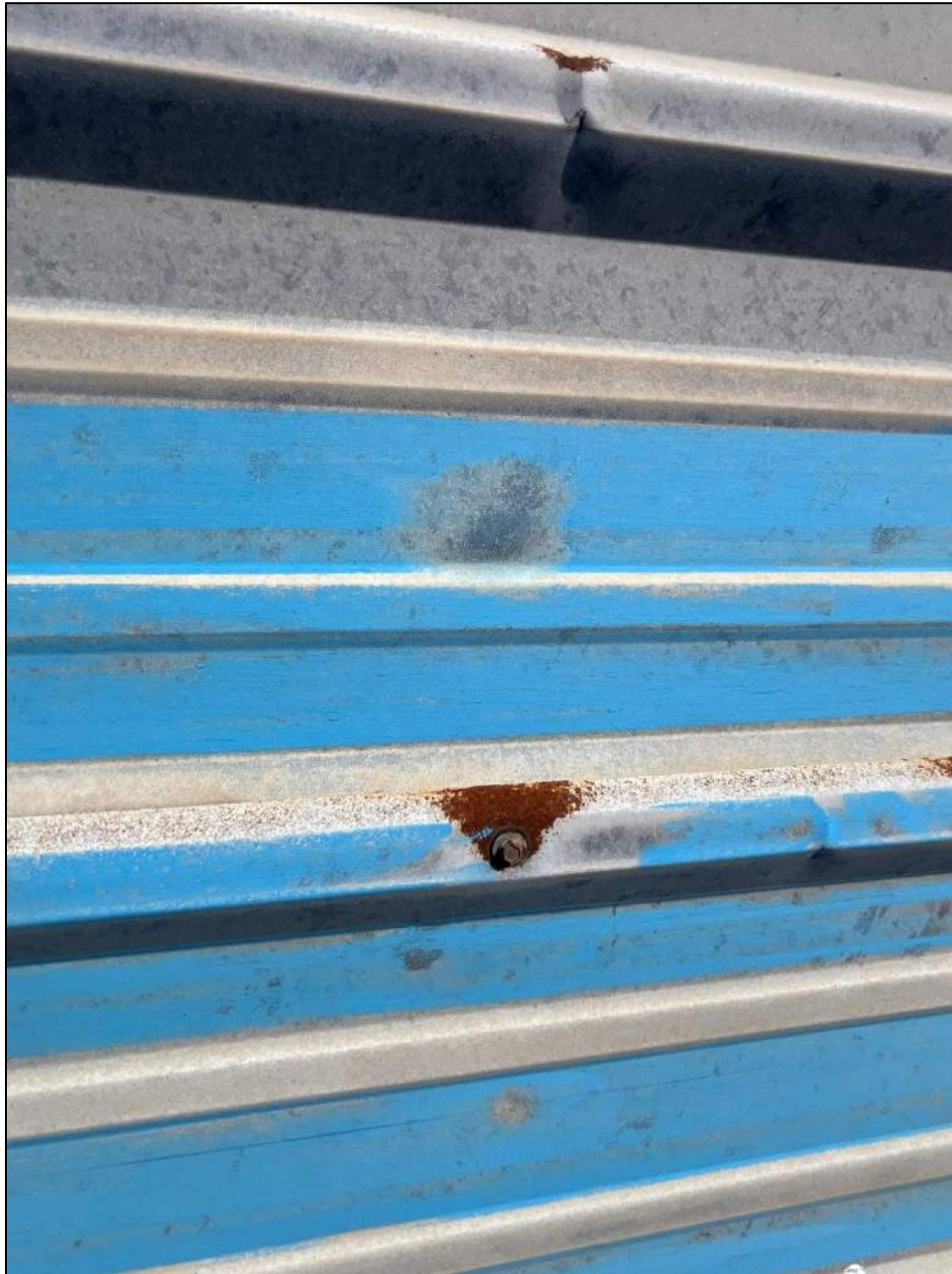
Photo 26: Denting observed on the metal roof panels had inner diameters of less than 1/2 inch.
