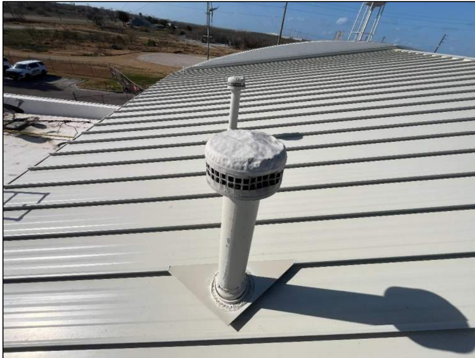
Photo 70: Dented aluminum mechanical exhaust vent on the east slope of the fire department roof consistent with hail.
