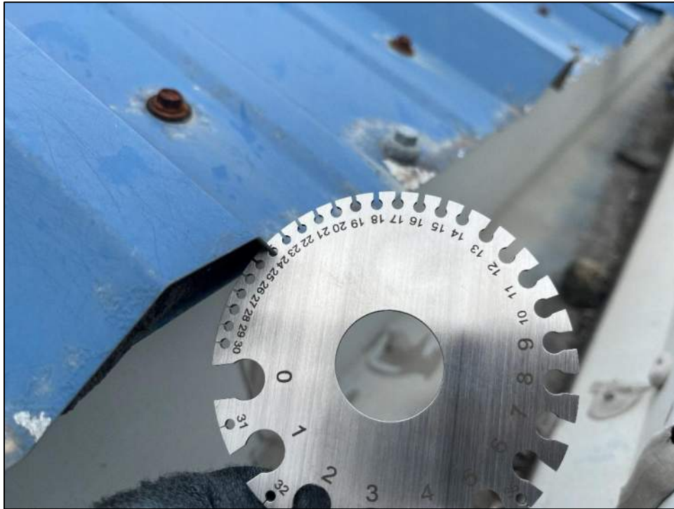
Photo 72: 24 gauge metal R-panel thickness.
