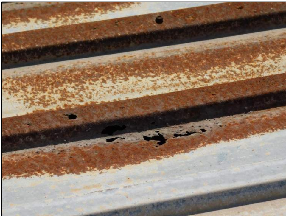
Photo 112: The storage building were severely corroded.
