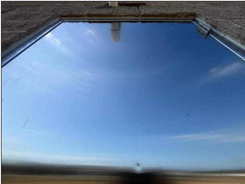
Photo 8: Stainless steel door was unaffected by hail.
