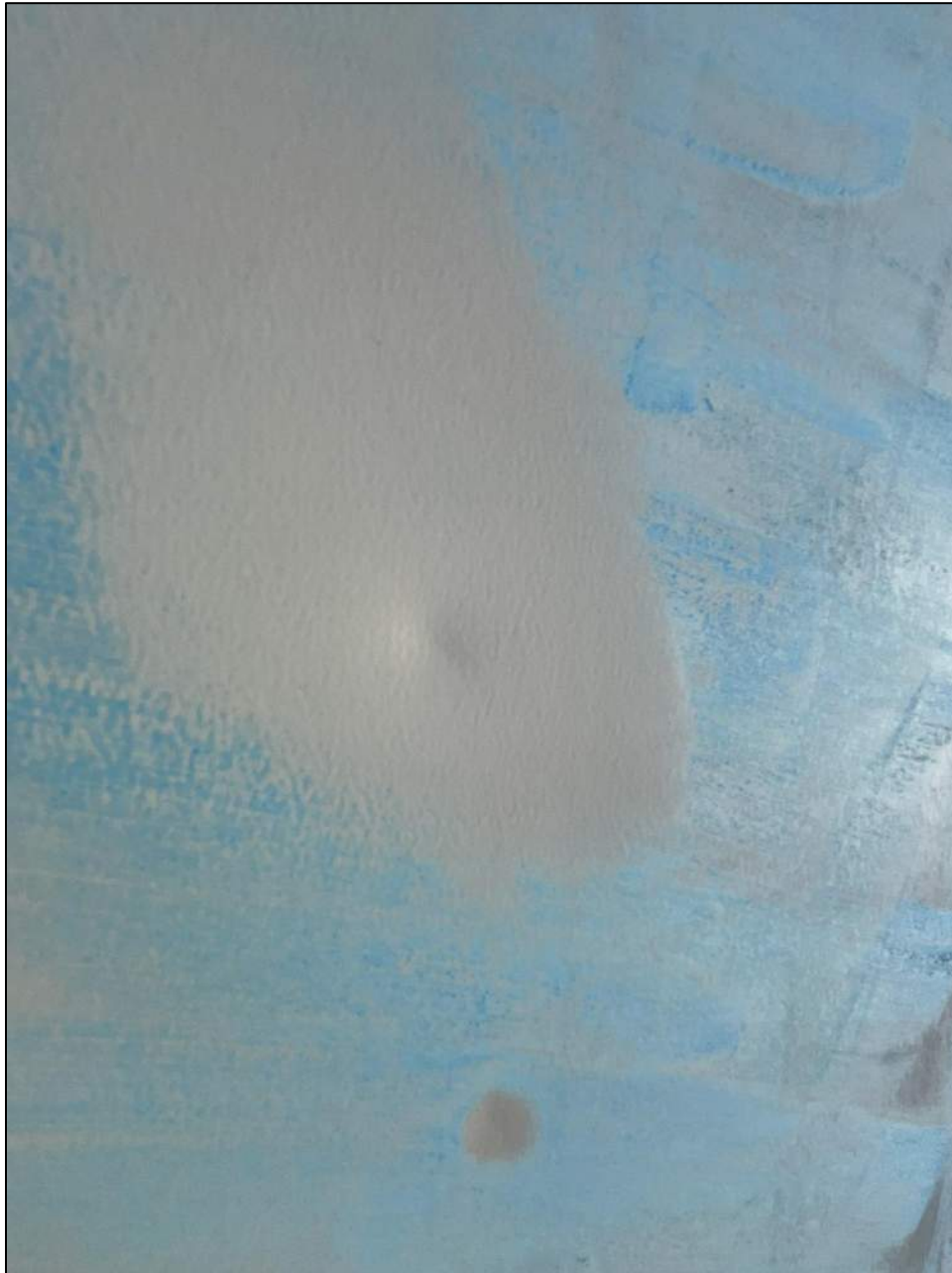
Photo 68: Dented ridge panel above the fire department. No coating disruptions were observed at the dents.
