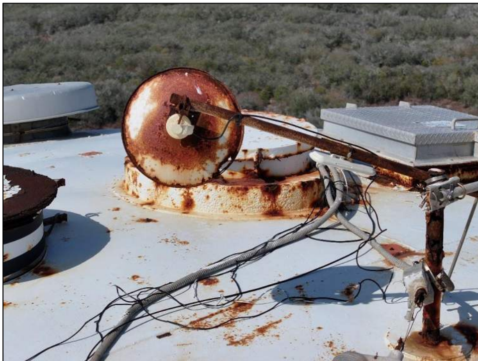
Photo 20: Additional view of severe corrosion on rooftop apparatus.
