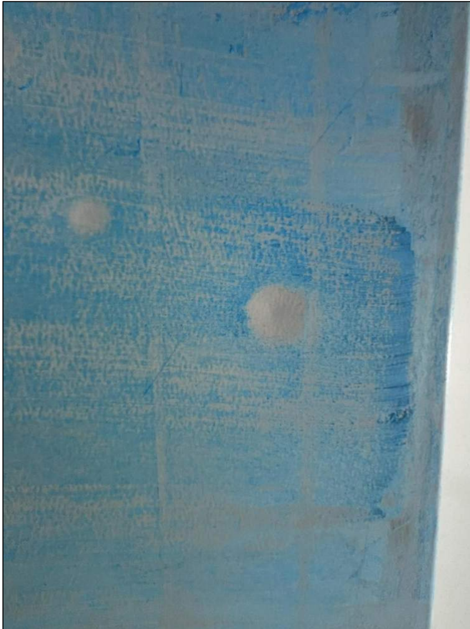
Photo 69: Dented ridge panel above the fire department. No coating disruptions were observed at the dents.
