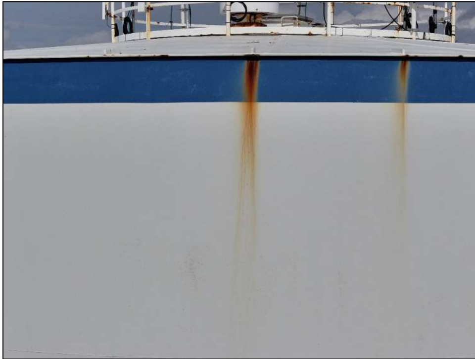
Photo 7: South elevation exhibited no hail spatters. Note steel corrosion.
