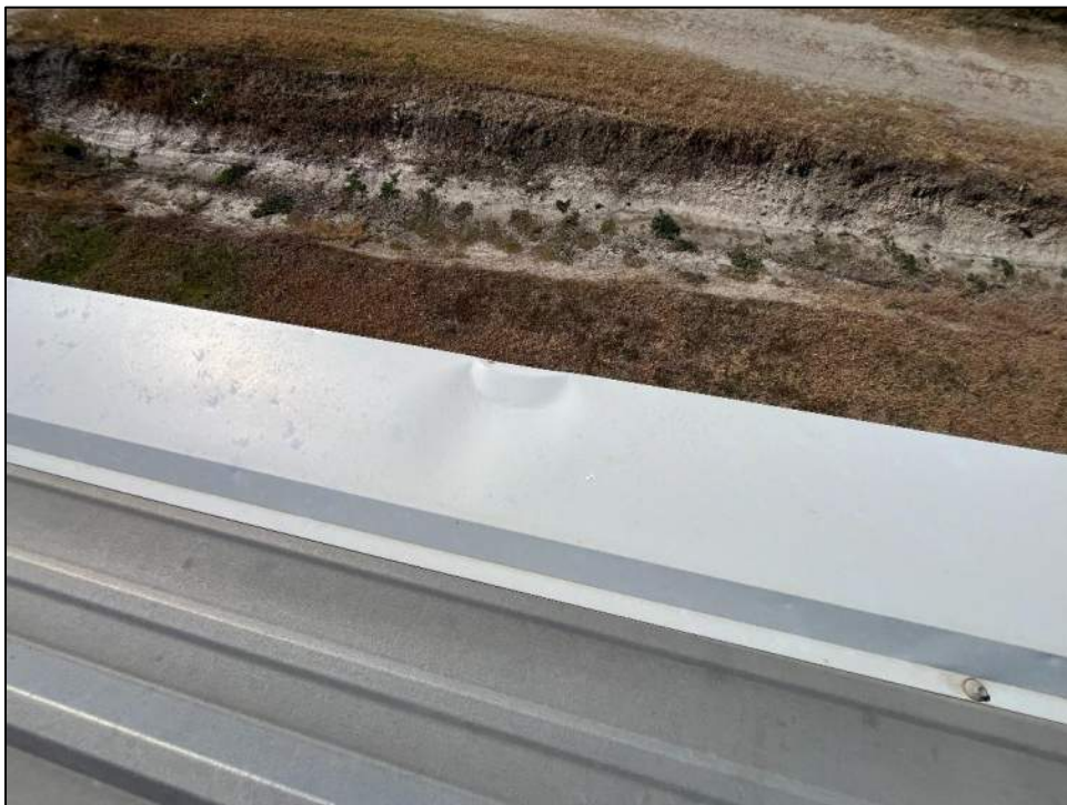
Photo 20: Edge crumpling along south roof rake consistent with mechanical impact.
