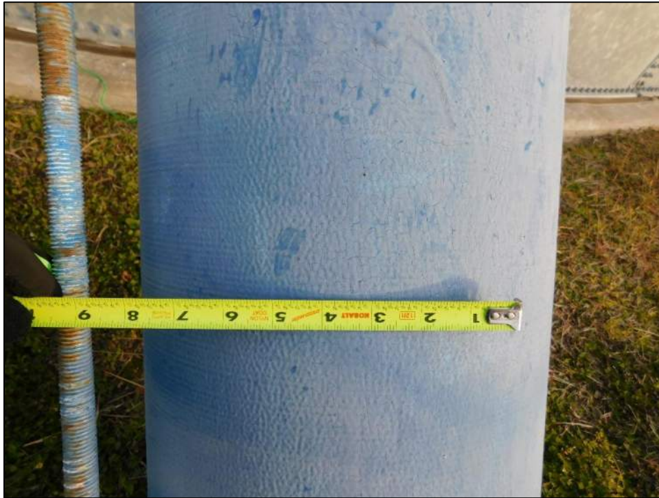
Photo 65: Hail spatter on tank piping.
