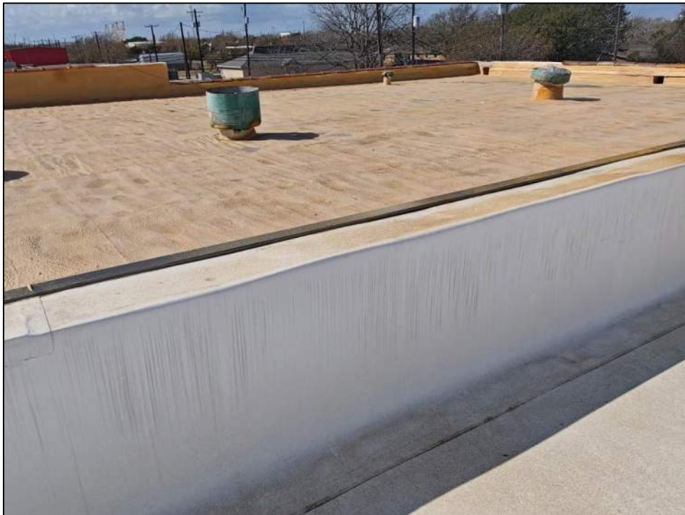
Photo 34: Unsupported PVC membranes at the base of parapets facing the direction of the hail were not punctured dimpled or scuffed.
