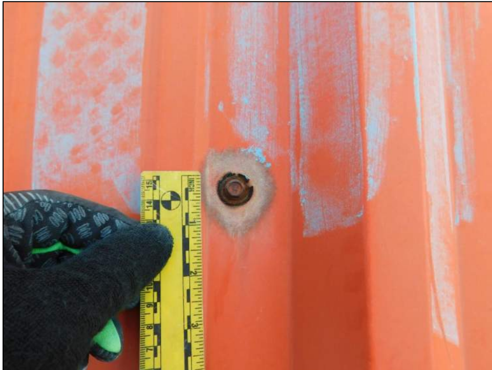
Photo 44: Typical fastener corrosion unrelated to hail impacts.
