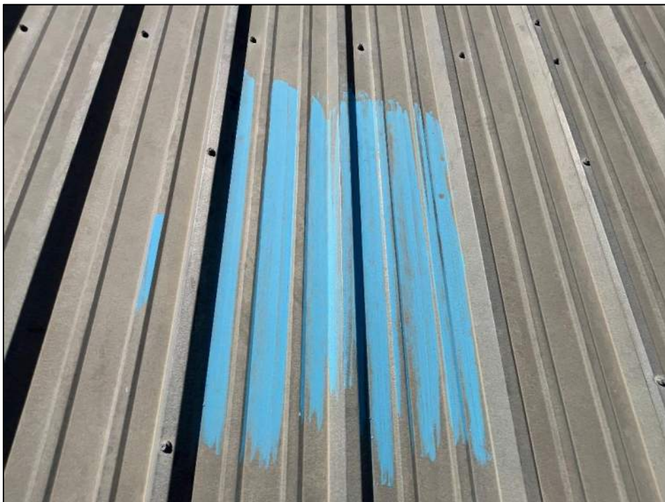
Photo 68: Denting in roof panels were minimal.
