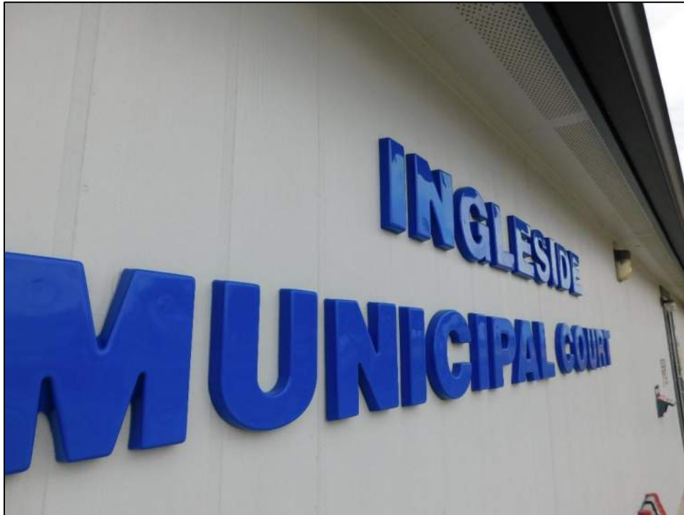
Photo 5: Dimensional building signage letters on north (front) wall were not fractured by hail impact.
