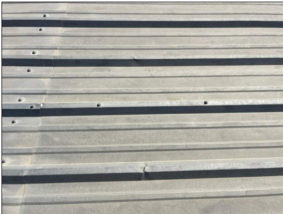
Photo 72: Rib creasing on roof unrelated to hail impact and consistent with foot traffic.
