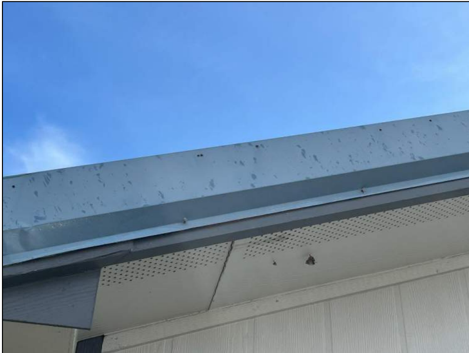
Photo 9: Hail spatters visible on the west gable rake closure metal.
