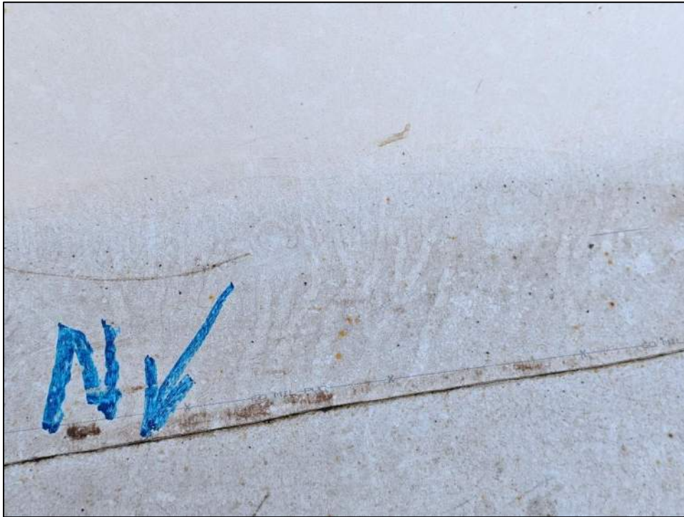
Photo 31: Unsupported PVC membranes at the base of parapets facing the direction of the hail were not punctured dimpled or scuffed.
