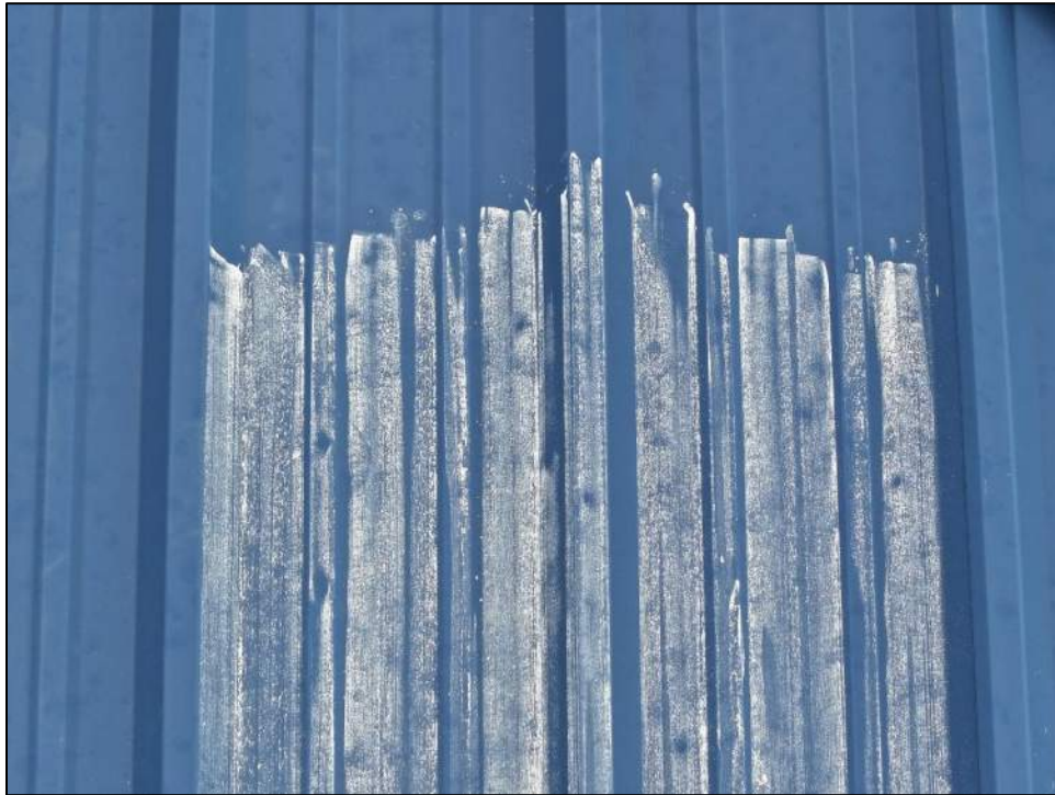
Photo 5: Close-up of the hail denting. The dents were generally shallow with an inner diameter of less than 3/8 inch.
