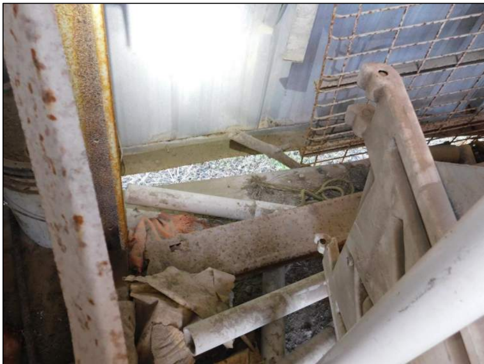
Photo 88: Bottom track of the bulged out west wall.
