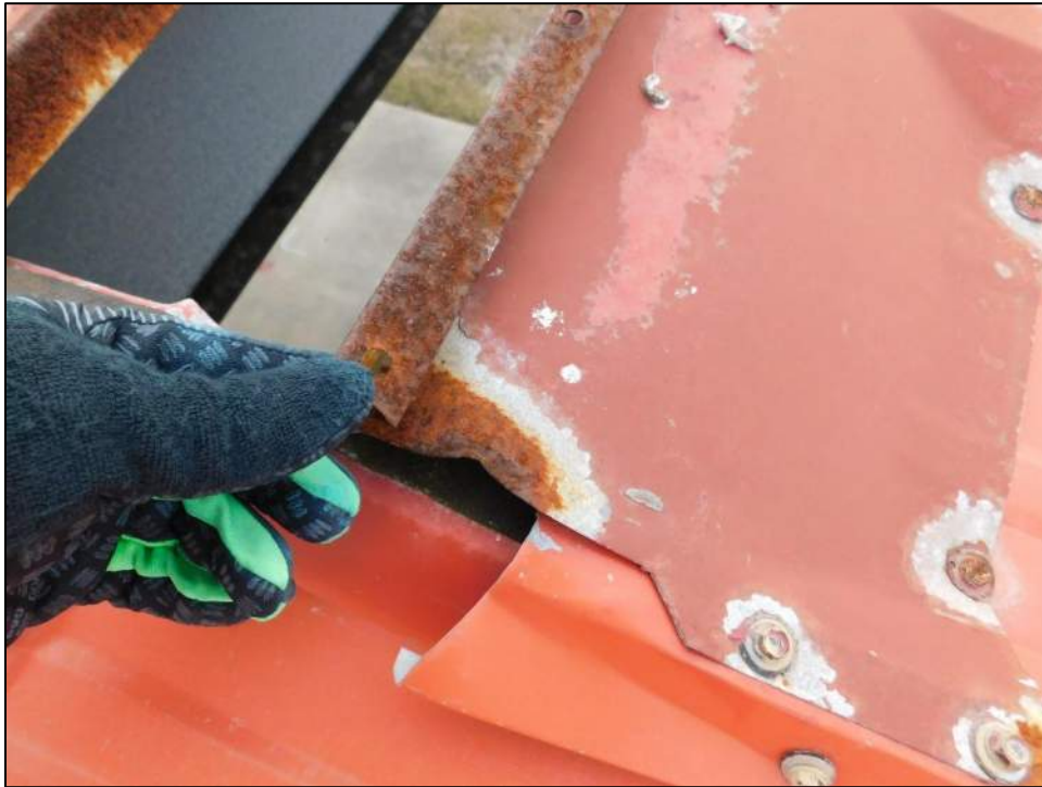
Photo 34: Corroded ridge vent curb.
