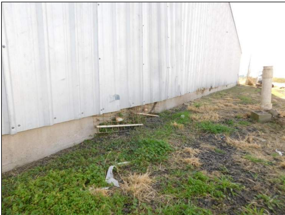
Photo 84: Lower section of the west wall bulged out.
