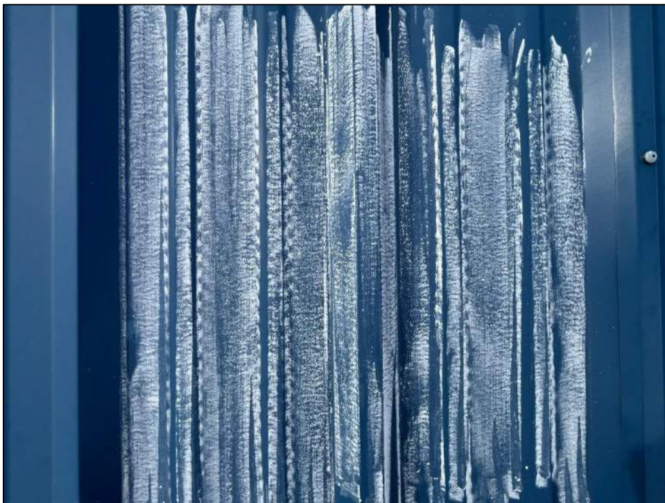
Photo 126: Hail denting on east slope was minimum compared to west and north slopes.
