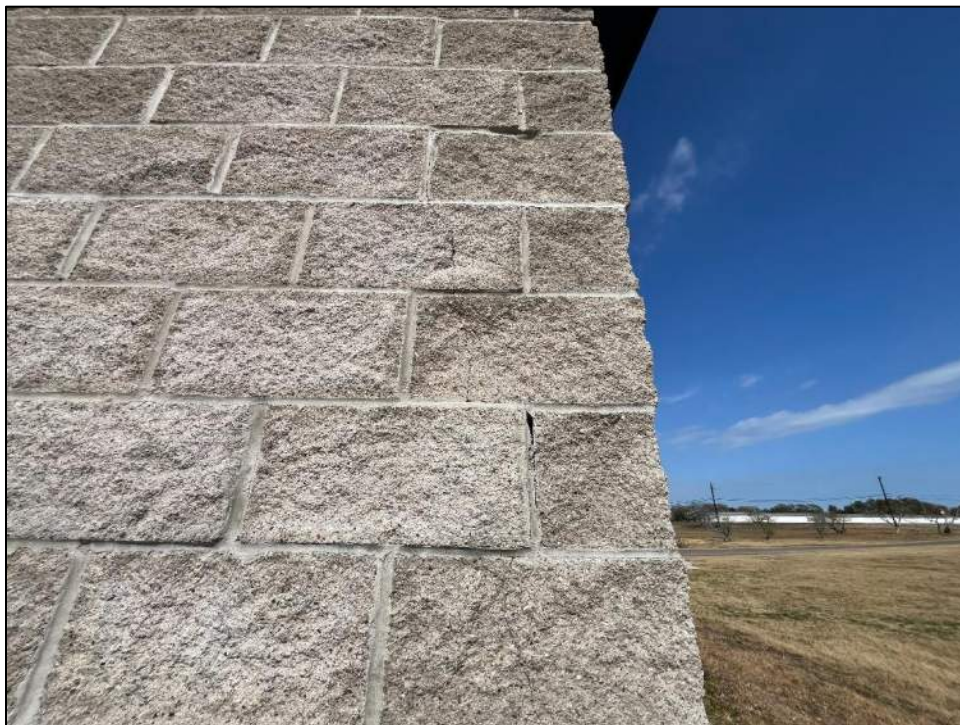
Photo 6: Masonry cracking at upper east corner unrelated to hail effects.
