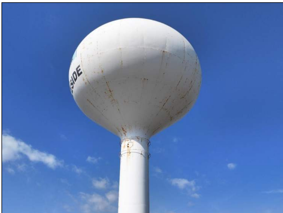
Photo 4: Underside of the tank exhibited widespread rusting.
