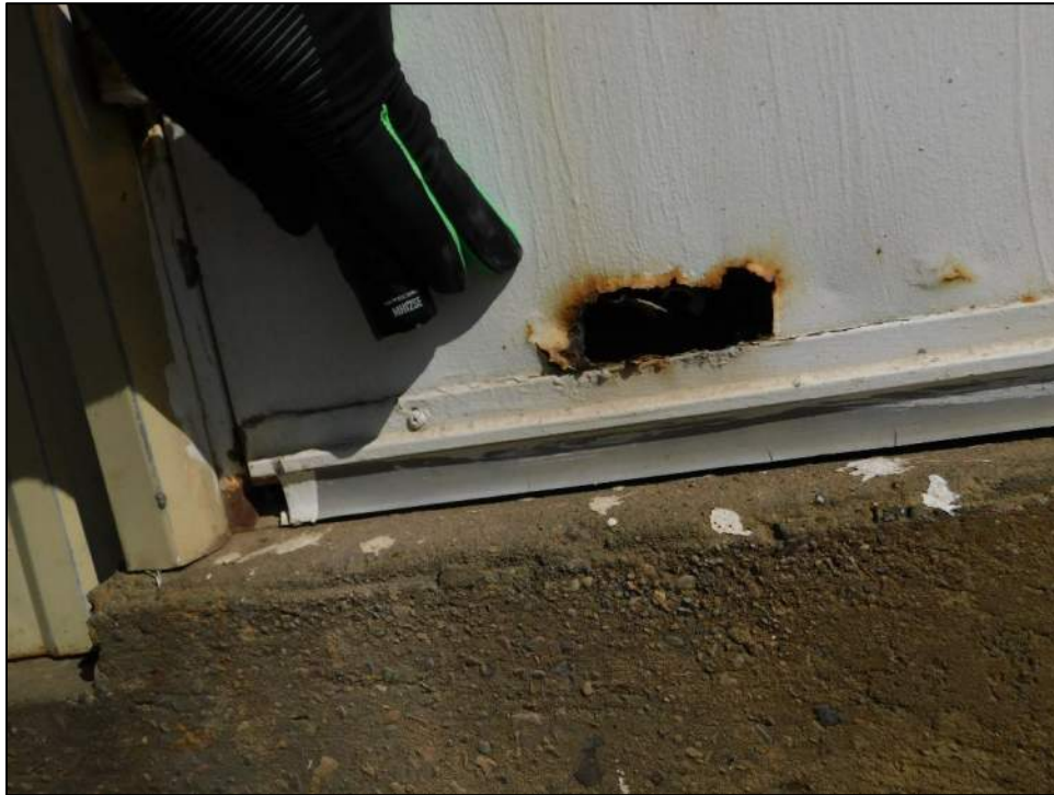
Photo 14: Corrosion at the bottom of the south entry door.
