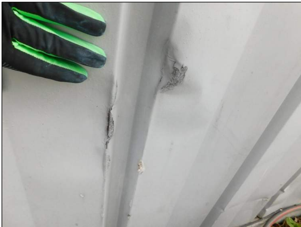
Photo 20: Closer view of the mechanical damage to the west wall lower section.
