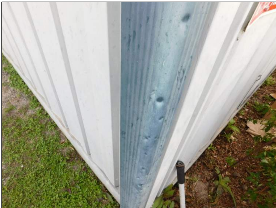
Photo 16: Dented aluminum downspout at the northwest wall corner.
