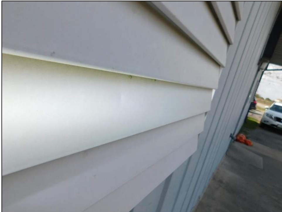
Photo 11: Aluminum shutters on front wall exhibited indentations consistent with hail impact.
