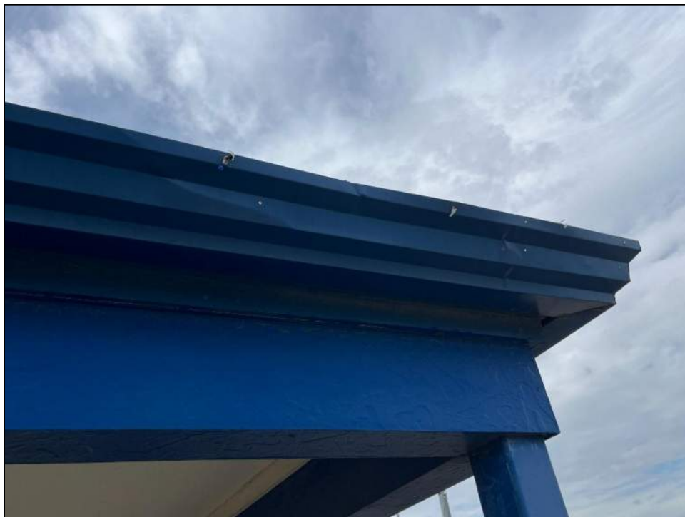
Photo 65: Mechanically deformed gutter.
