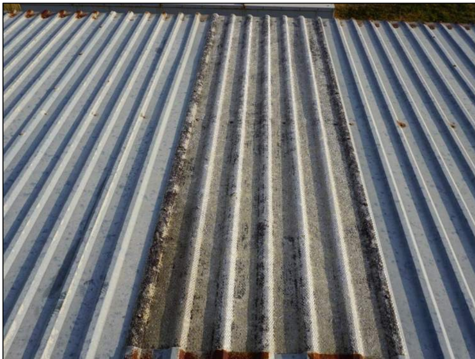
Photo 48: Deteriorated skylight panels exhibited isolated hail impact fractures.
