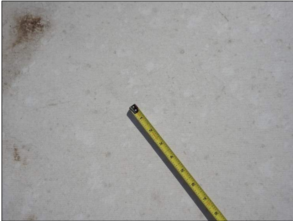
Photo 9: Spatters on PVC roofing reflect 1-inch hail.
