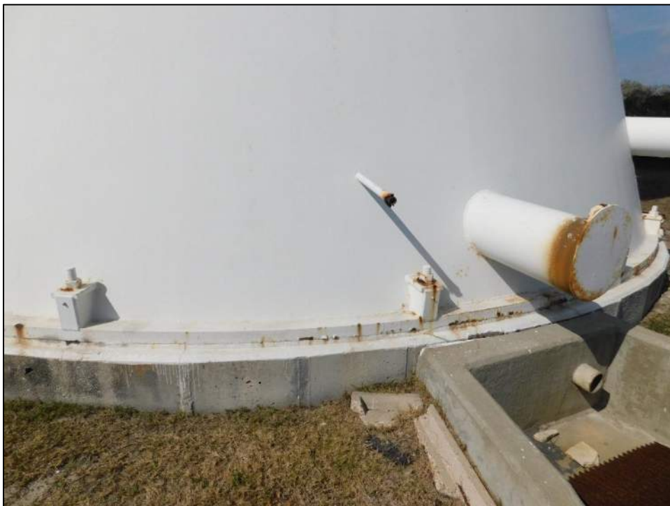
Photo 10: Corroded drain pipe.
