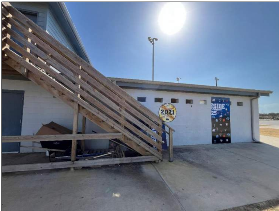
Photo 4: West elevation. Wooden stairs facing west exhibited hail spatters.
