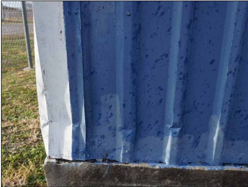
Photo 43: Mechanical damage at the lower east corner of the north wall irrelevant to hail effects.
