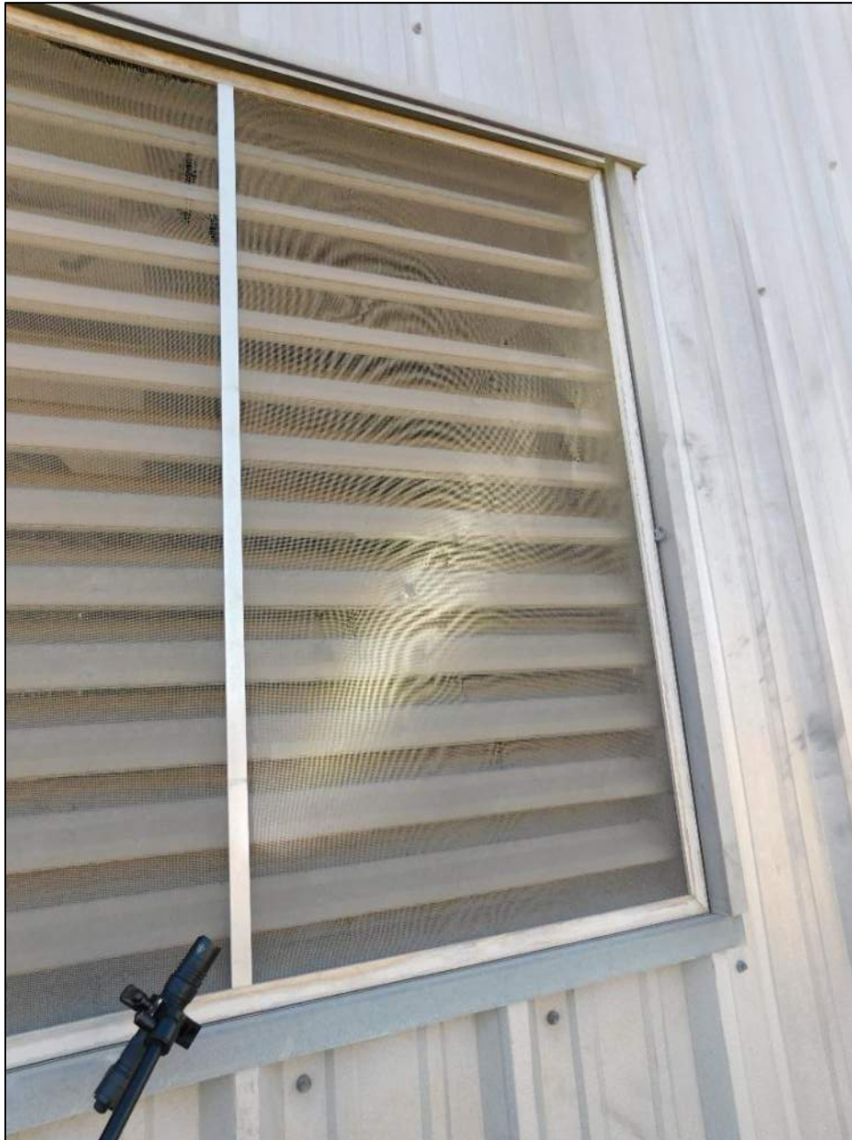
Photo 57: Dimpling of screen at louver windows along the north wall consistent with hail impact.
