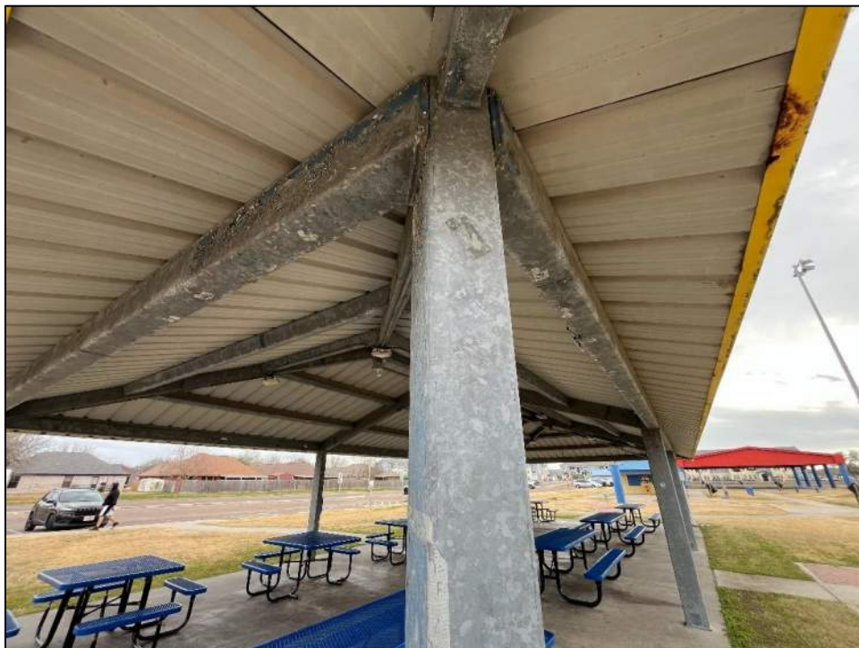
Photo 79: Tube steel framing remained intact.
