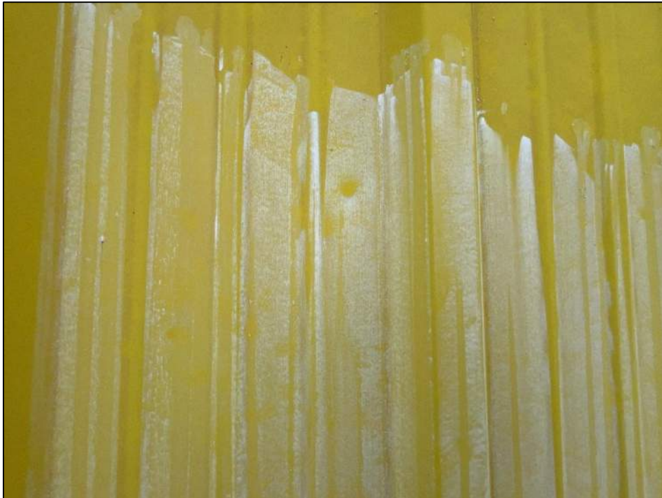
Photo 84: Inner diameter of hail dents on north slope were less than 1/2 inch.
