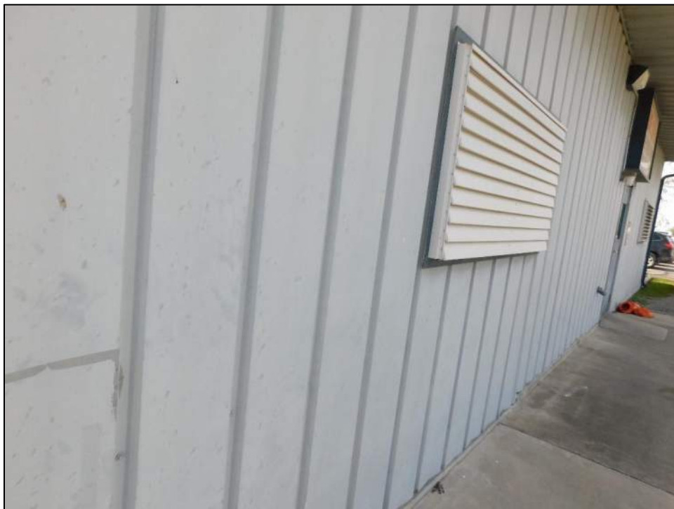
Photo 10: Spatters on front wall.
