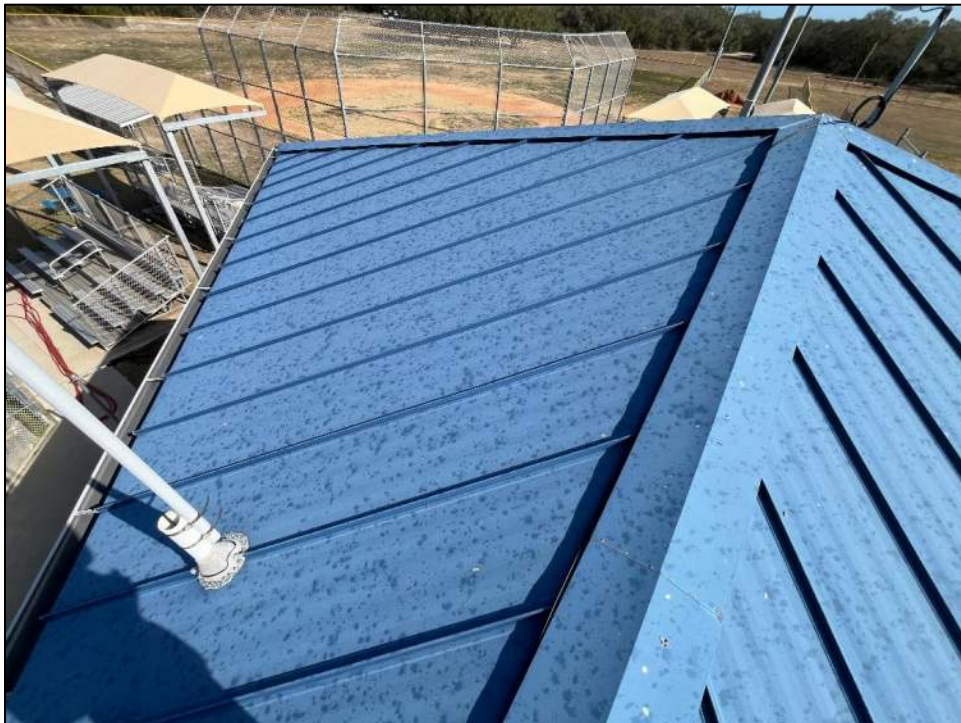
Photo 30: Widespread hail spatters observed on the high roof.
