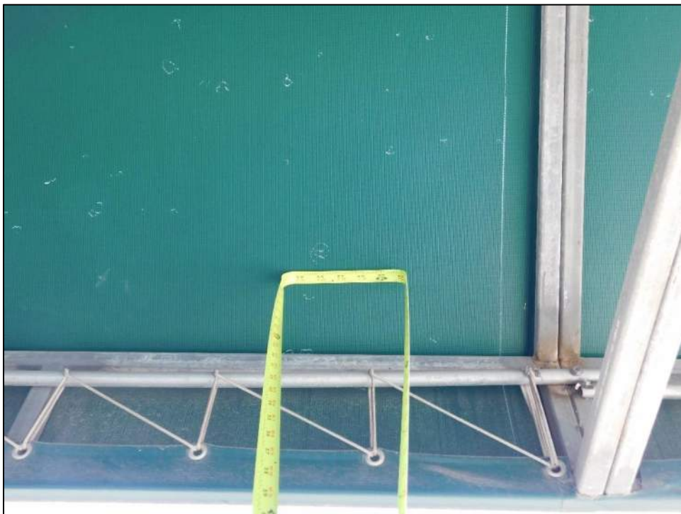
Photo 20: Hail impact fractures observed from the underside of the PVC fabric awning.
