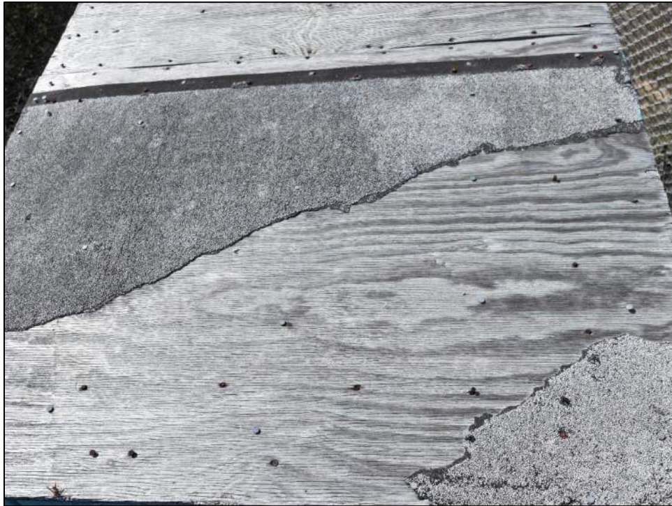
Photo 79: No wood grain crushing or disruption observed on the deteriorated shed roof deck (exposed due to rolled-roofing deterioration).
