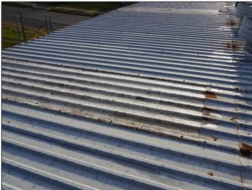
Photo 46: Deteriorated skylight panels exhibited isolated hail impact fractures.
