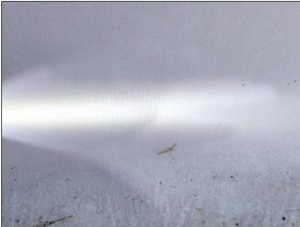
Photo 32: Unsupported PVC membranes at the base of parapets facing the direction of the hail were not punctured dimpled or scuffed.
