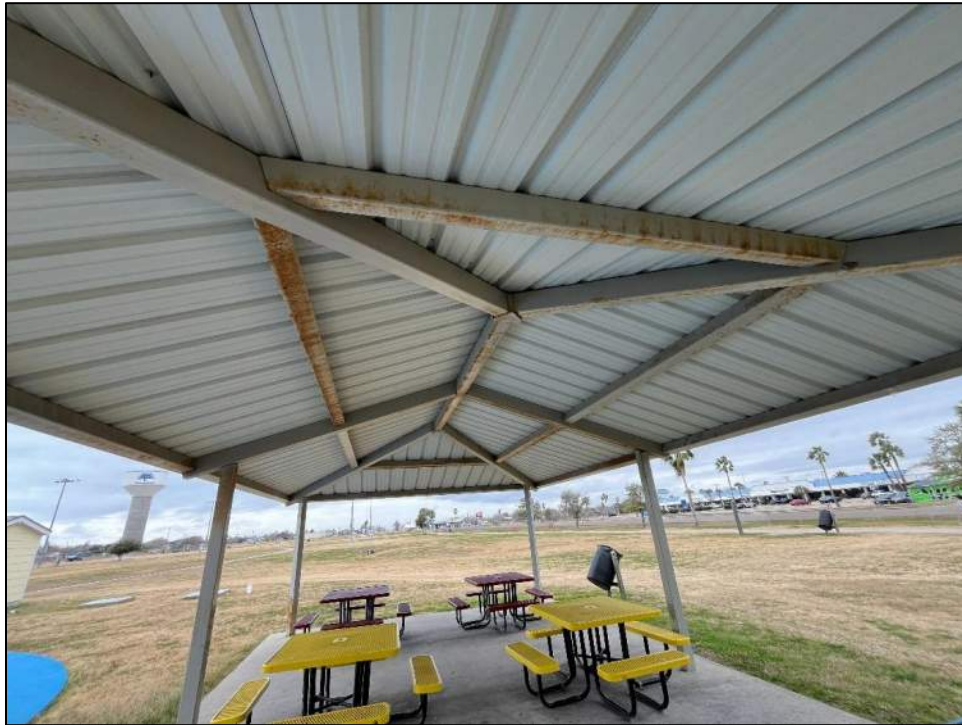
Photo 9: Underside view of the pavilion structure. Tube steel frames remained intact in addition to rusting.
