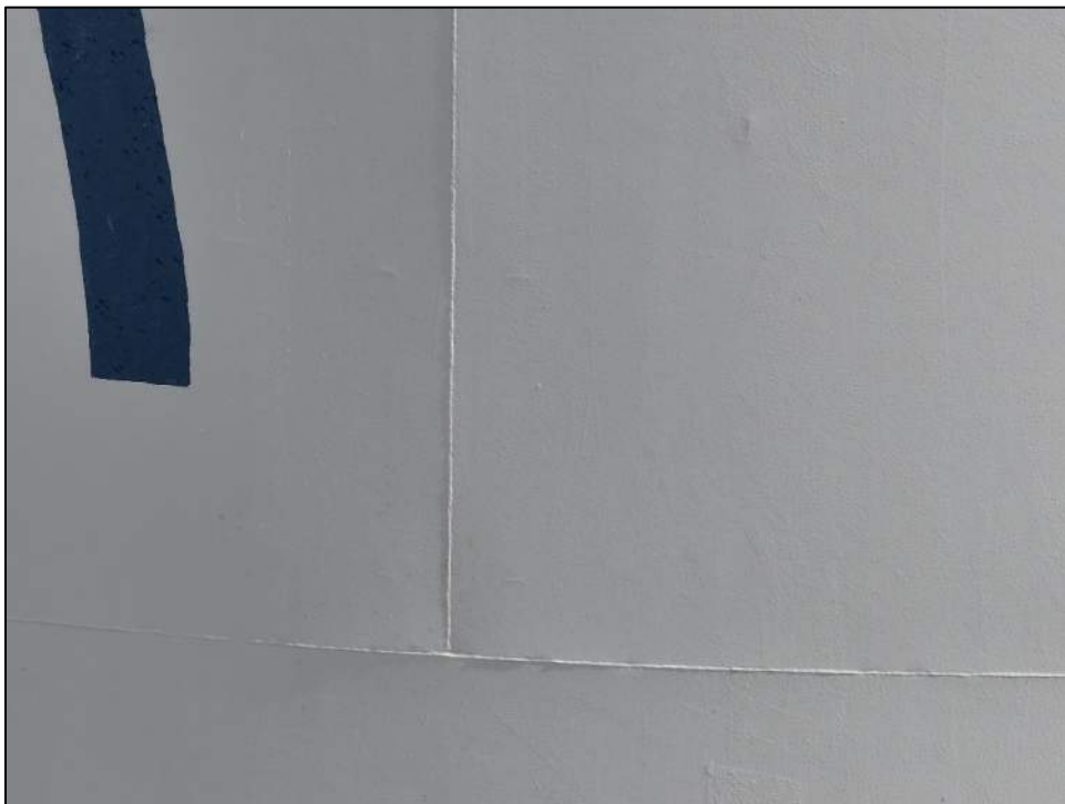
Photo 6: Wall surfaces remained intact from hail impact.
