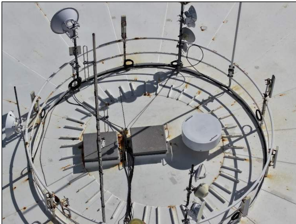
Photo 2: Rooftop appurtenance remained attached to the circular ring frame and upright.
