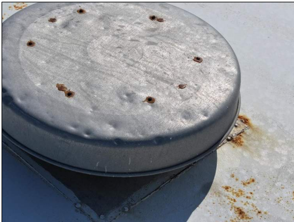
Photo 22: Hail denting on circular aluminum vent cover were consistent with recent hail impact.
