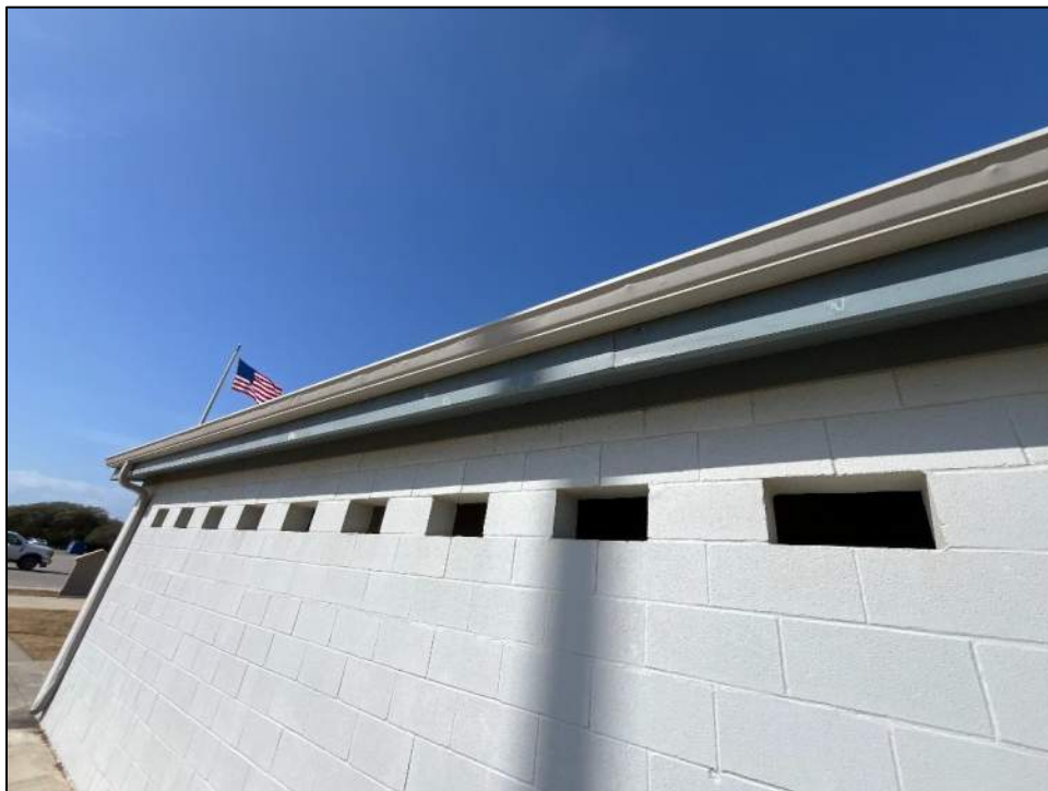
Photo 6: Gutter walls facing north exhibited outward denting consistent with the November 1, 2025 hail impact.
