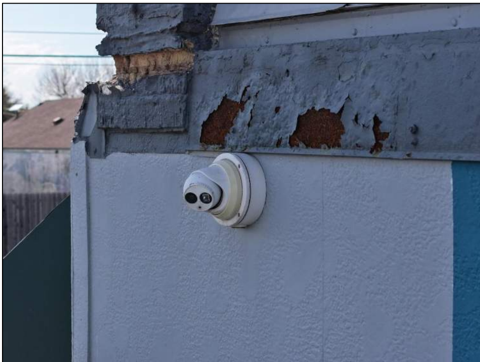
Photo 6: Pre-existing paint peel in north wall.
