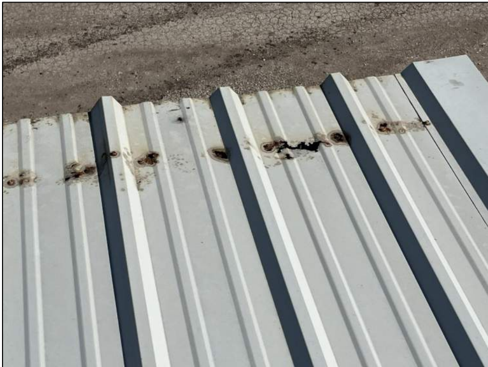
Photo 30: Severe deck edge corrosion along north edge of the canopy extension that were irrelevant to hail impact.
