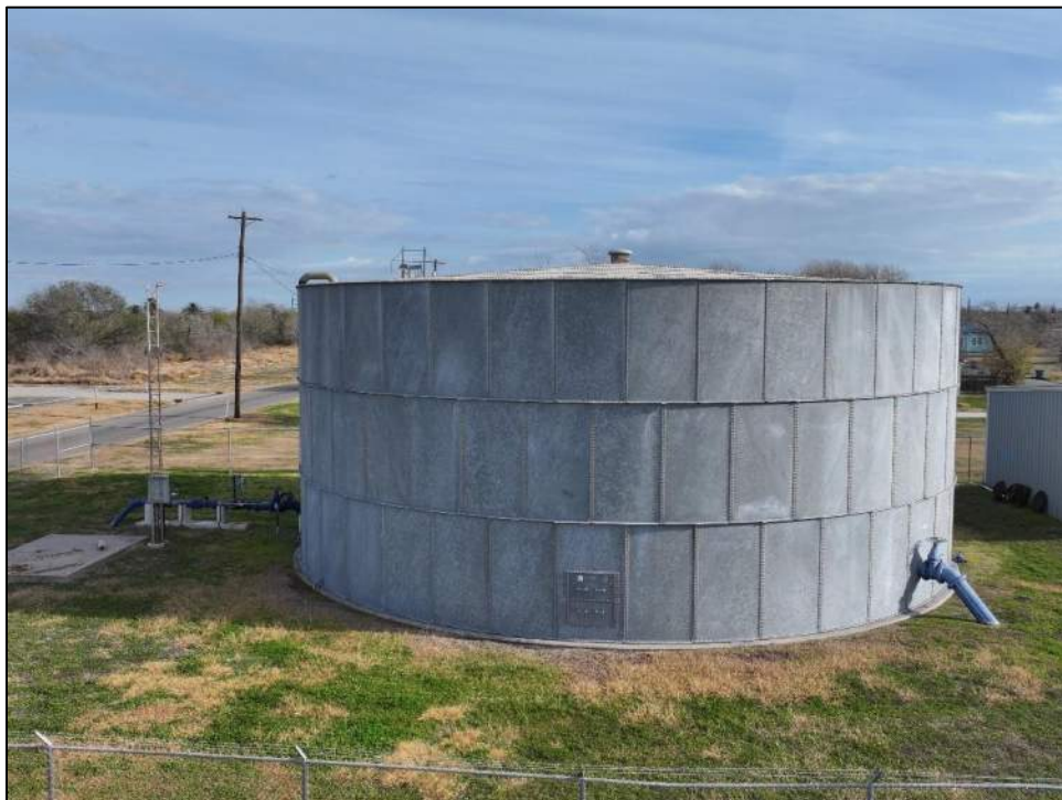
Photo 60: Water department ground water tank overview.
