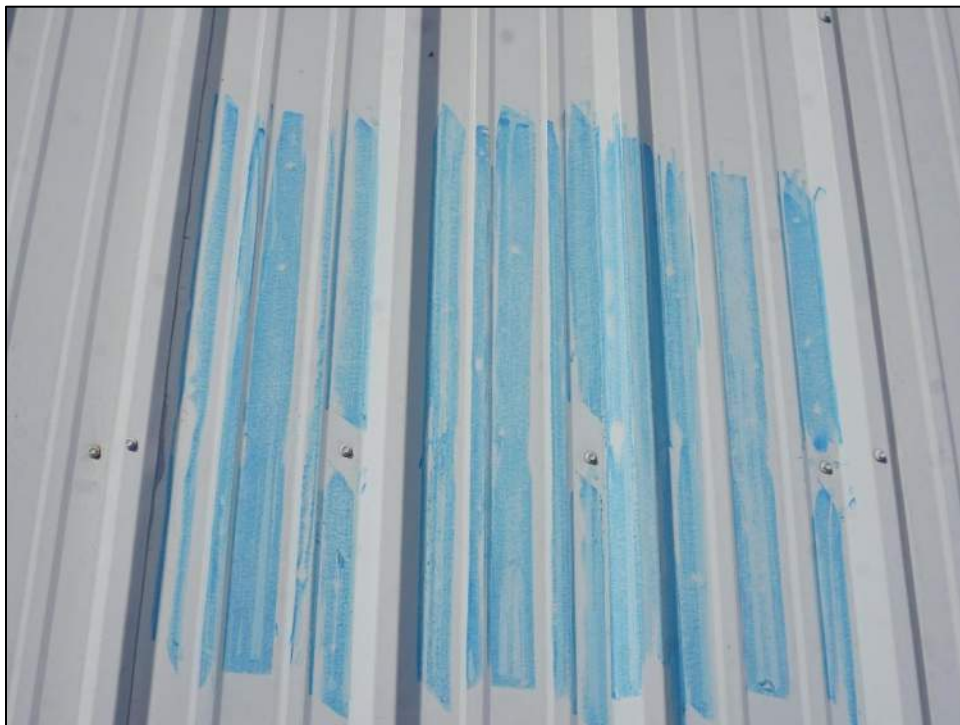
Photo 24: North slope hail dents had inner diameter less than 1/2 inch.
