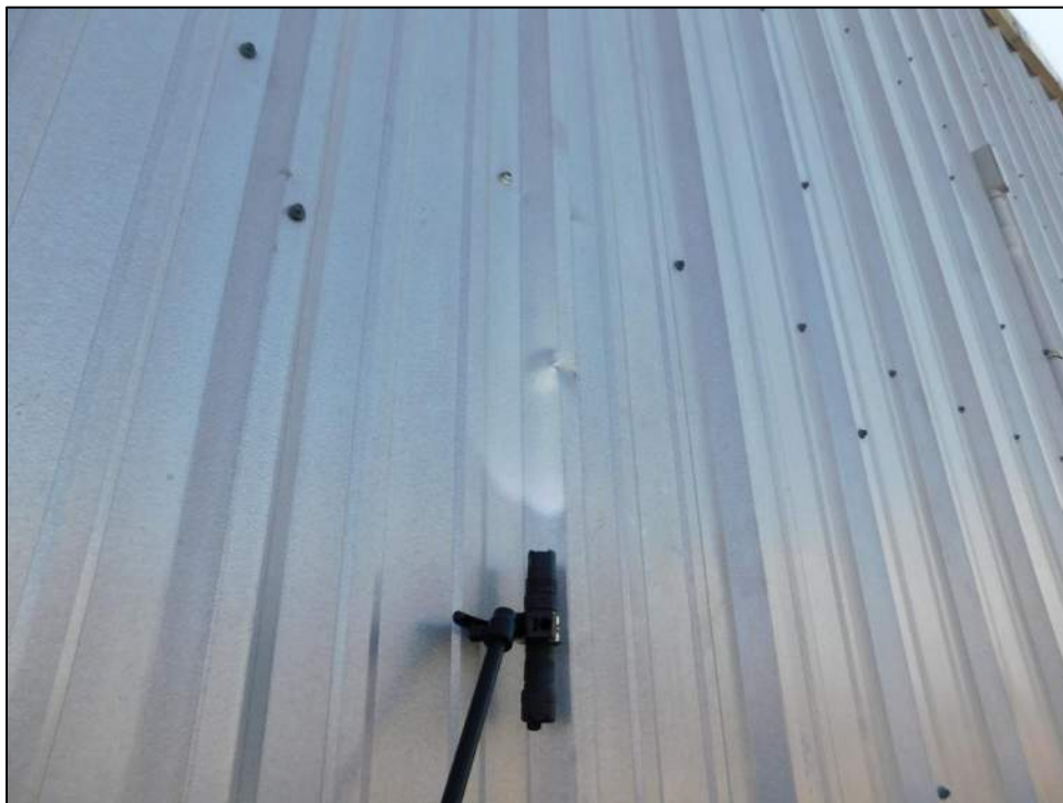
Photo 62: Rib creasing on west wall inconsistent with hail impact.
