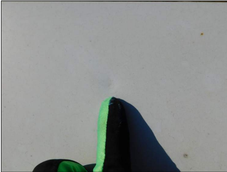
Photo 103: Hail denting on the closure metal exhibited no disruptions to the surface coating.
