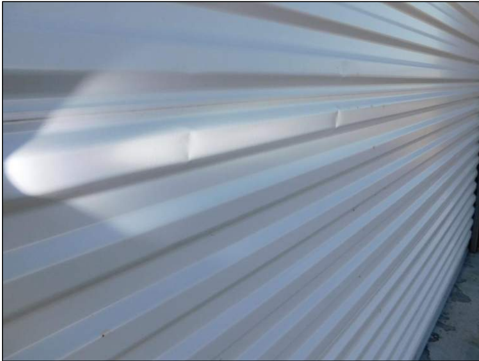
Photo 11: Creasing visible at the lower sections of the south roll-up door.
