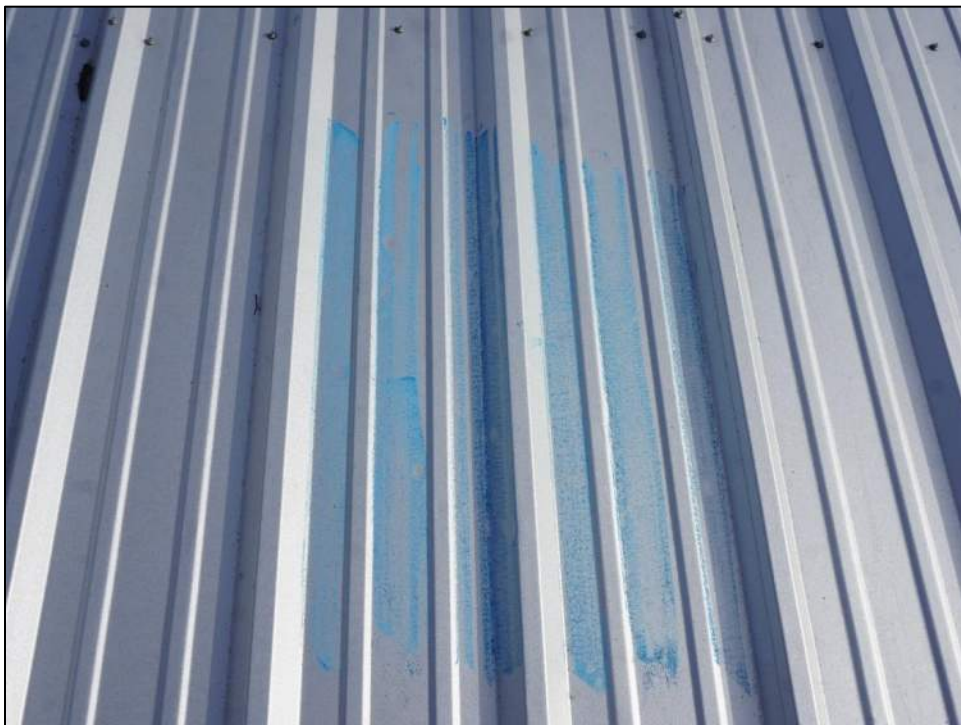
Photo 21: Hail denting on south slope had an inner diameter of less than 3/8 inch.
