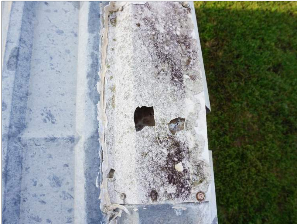
Photo 47: Fractured deteriorated vinyl closure flashing at the east and west ridge ends consistent with weathering and recent hail impact.
