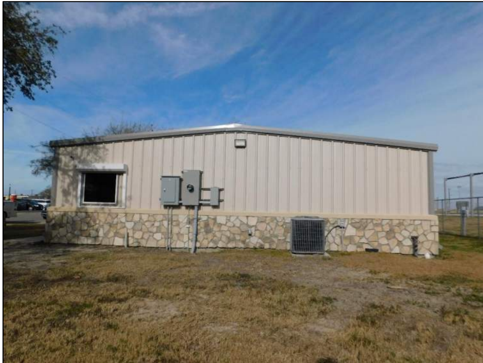
Photo 5: East elevation. The window glazing remained intact. No hail spatters were observed on the electrical panels.
