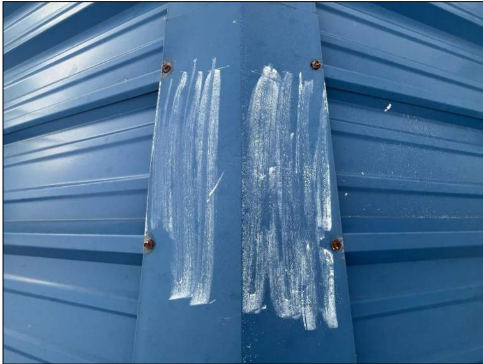
Photo 17: Ridge caps exhibited slight denting. Note the rusted fasteners.
