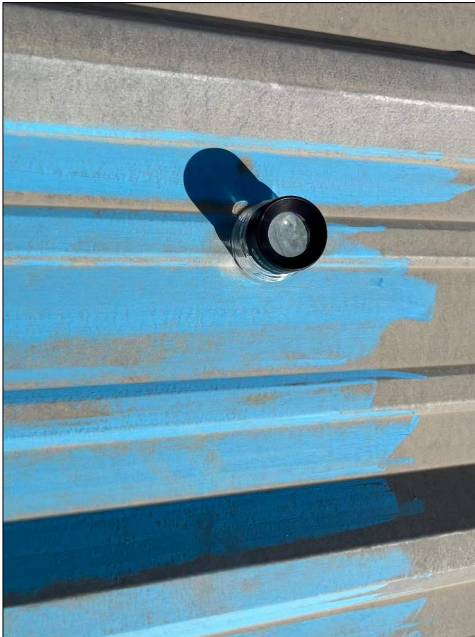
Photo 96: No coating disruptions were observed at the hail denting.
