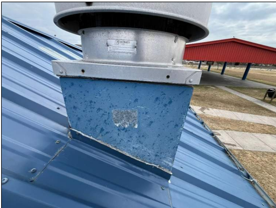
Photo 131: Hail spatters on north-facing curb of a vent hood on the west slope.
