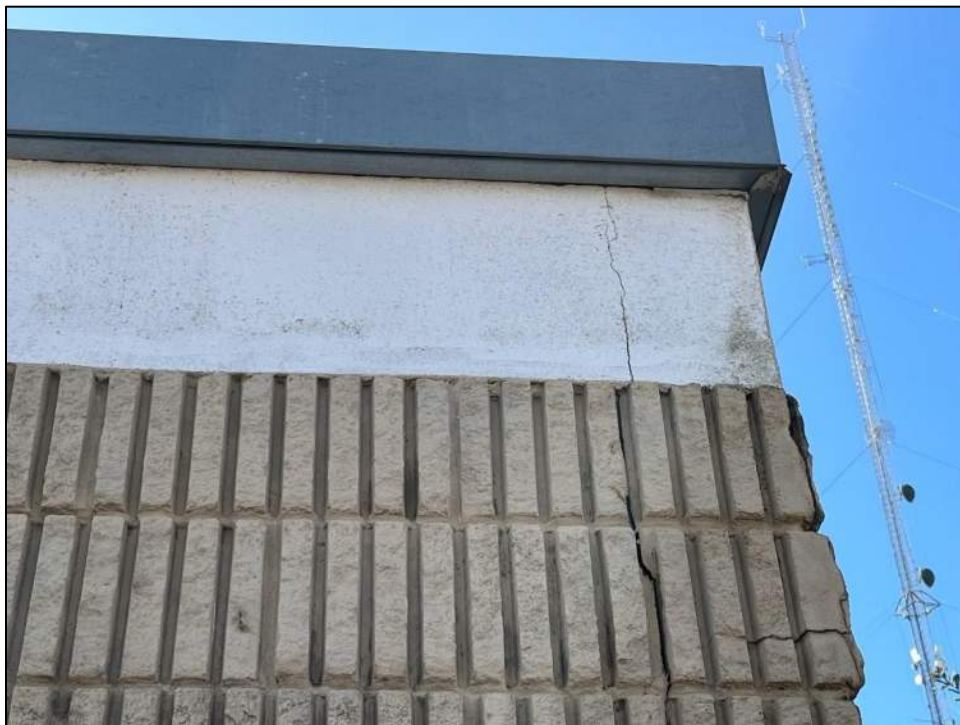
Photo 39: Cracked masonry wall corner (northwest) unrelated to hail impact.
