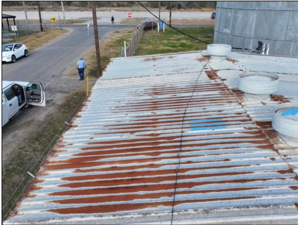
Photo 45: Widespread corrosion on the roof deck irrelevant to the subject hail storm.
