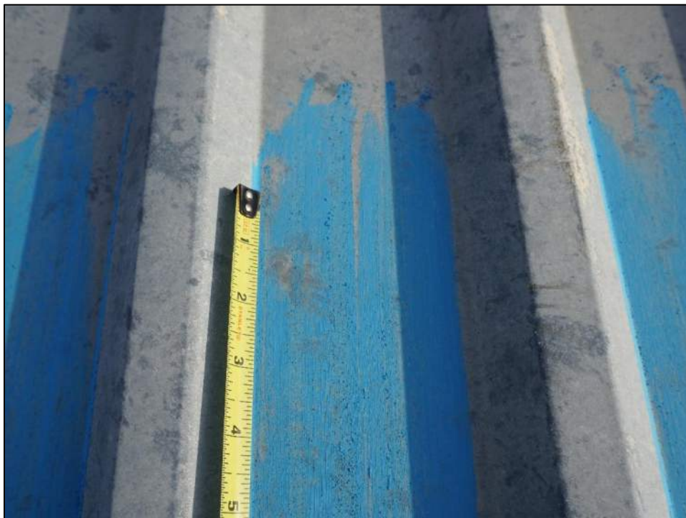
Photo 52: Hail denting on metal roof deck.
