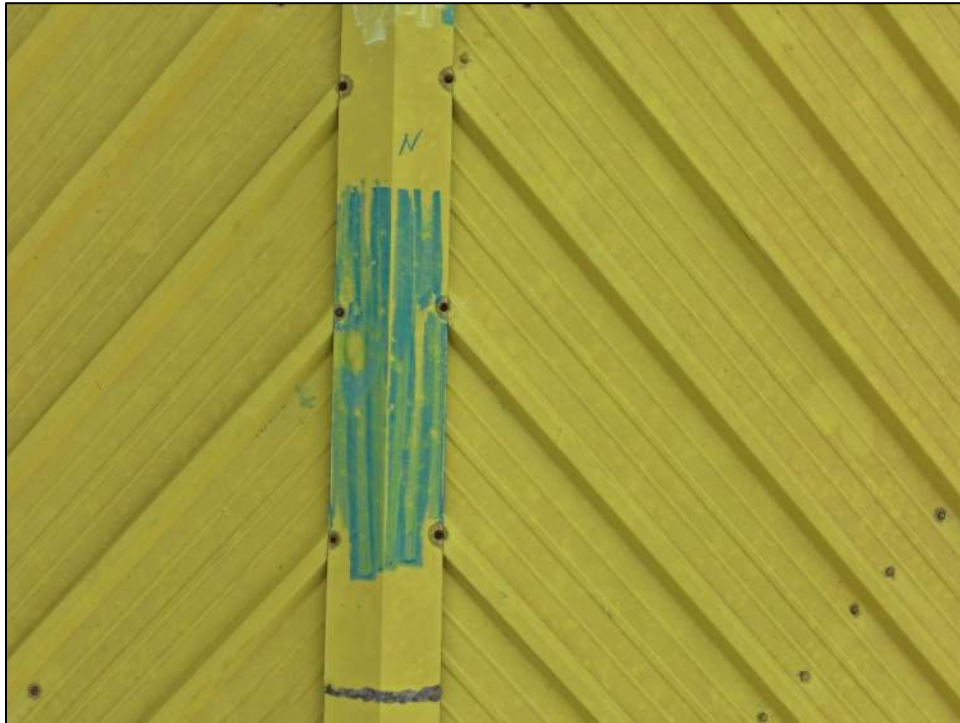
Photo 82: Dents in north-facing ridge cap were consistent with recent hail impact.
