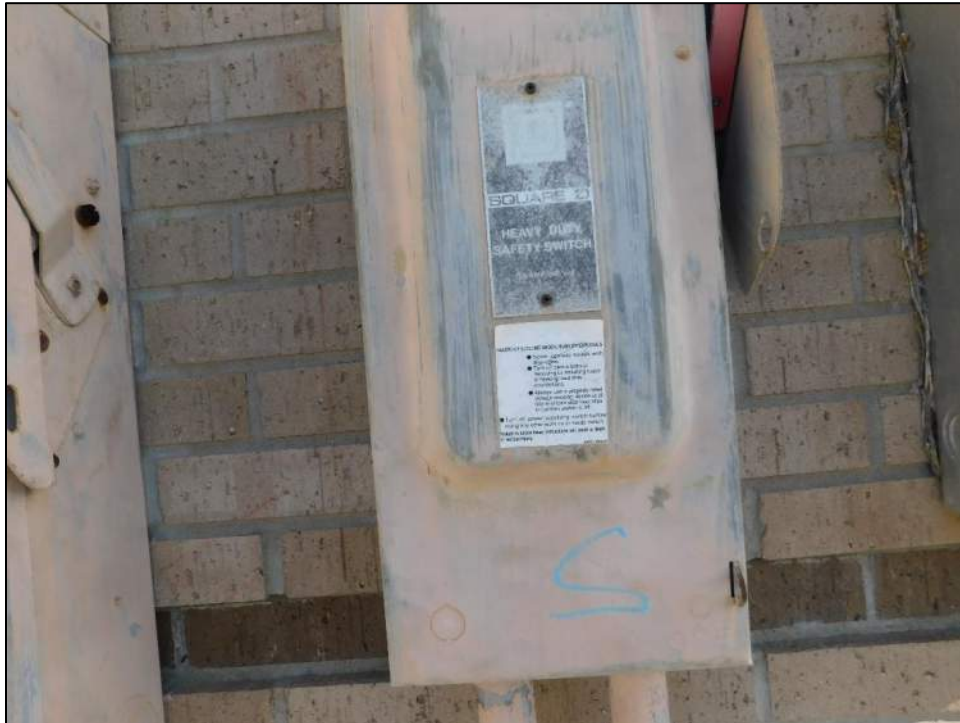
Photo 43: No hail spatter on south-face electrical safety switch boxes.
