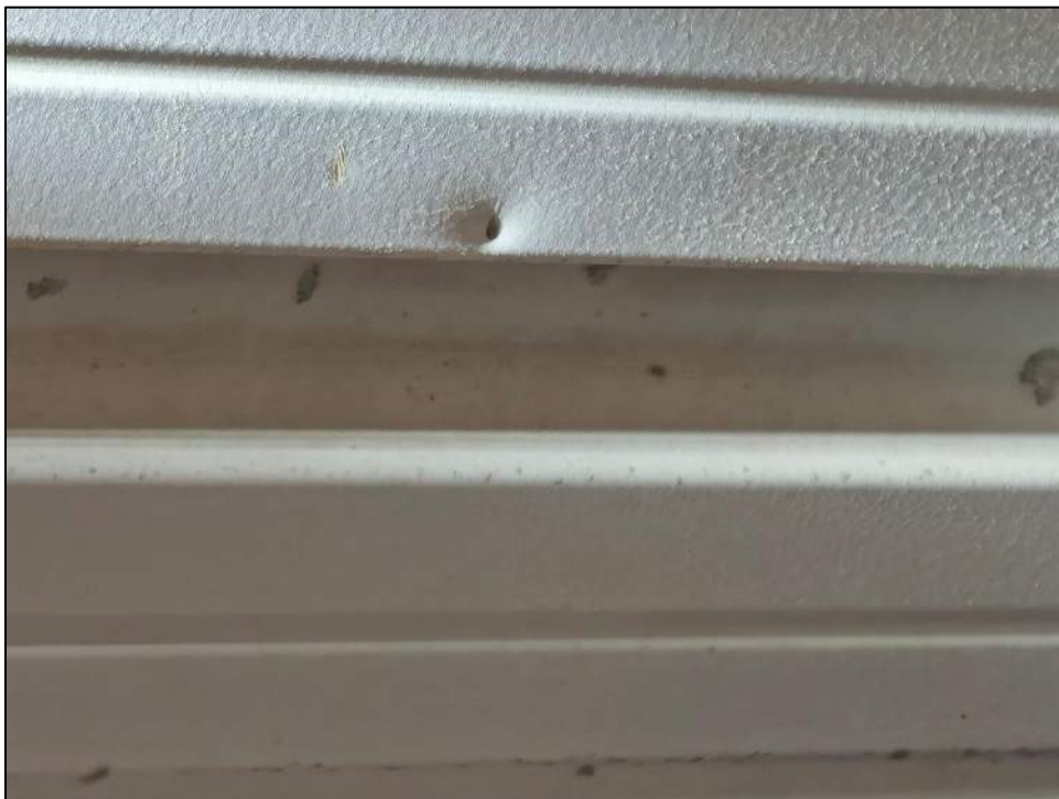
Photo 89: Close-up view of the underside of the metal roof deck with the upward denting.
