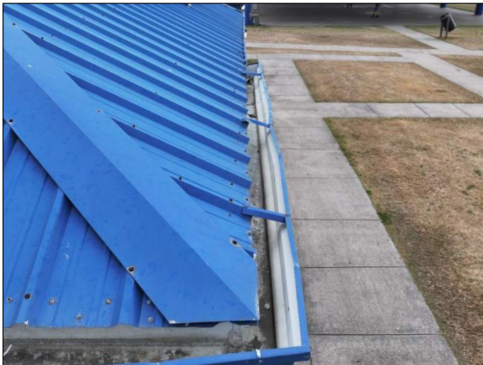
Photo 53: Mechanically deformed gutter along west slope eave.
