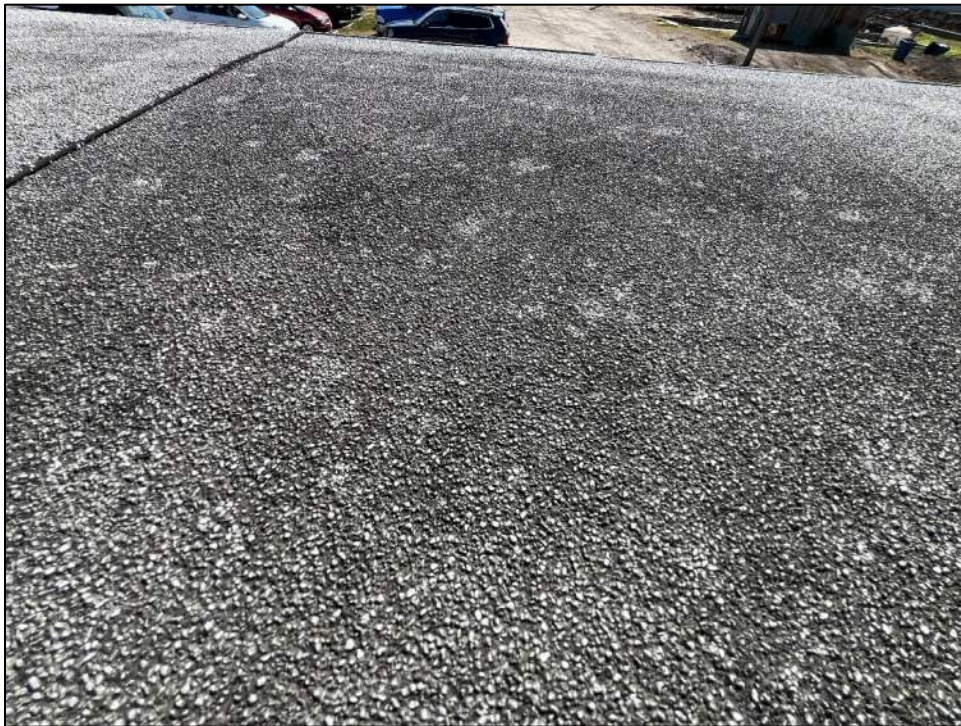
Photo 45: Hail dimpling or granule disruptions were observed at the hail spatters.
