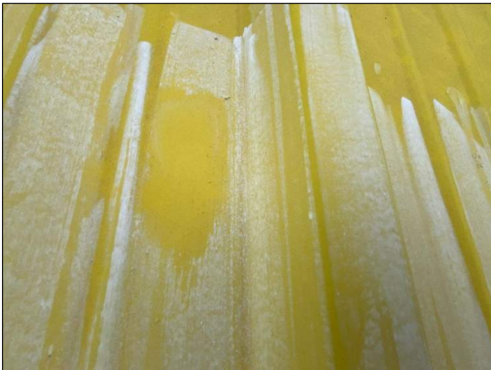
Photo 85: No coating disruptions were observed at the hail dents.
