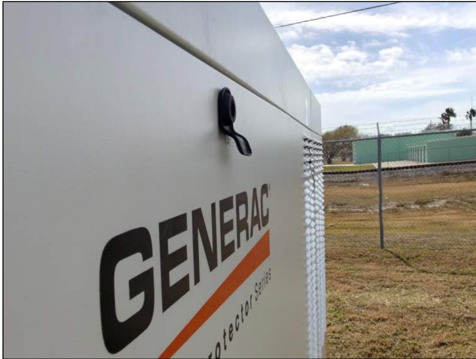
Photo 20: Ground-based generator wall casing remained free of denting.
