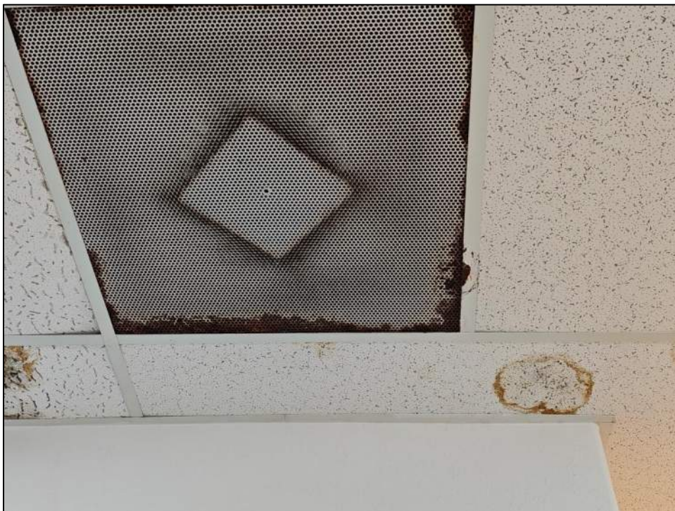
Photo 32: Aged stains on ceiling was confirmed by building staff as pre-existing. No additional new roof leaks or stained ceiling tiles were reported since the storm.
