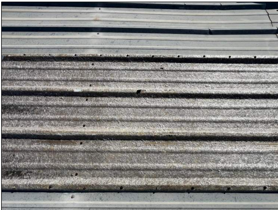
Photo 25: Isolated fractures in deteriorated skylight panels were consistent with hail impact.
