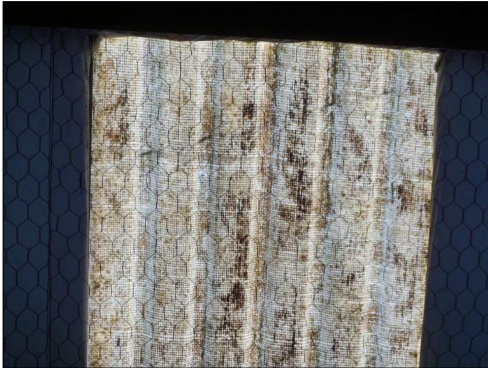
Photo 59: Isolate circular fractures in skylight panels consistent with hail impact.
