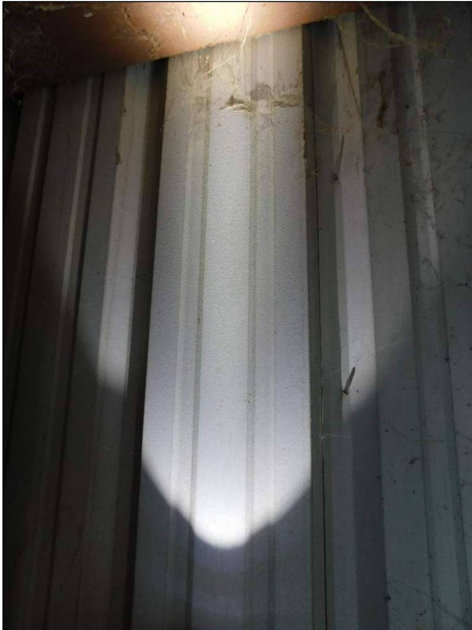
Photo 17: No hail denting observed on the interior surface of the north walls where hail spatters were observed on the exterior surfaces.
