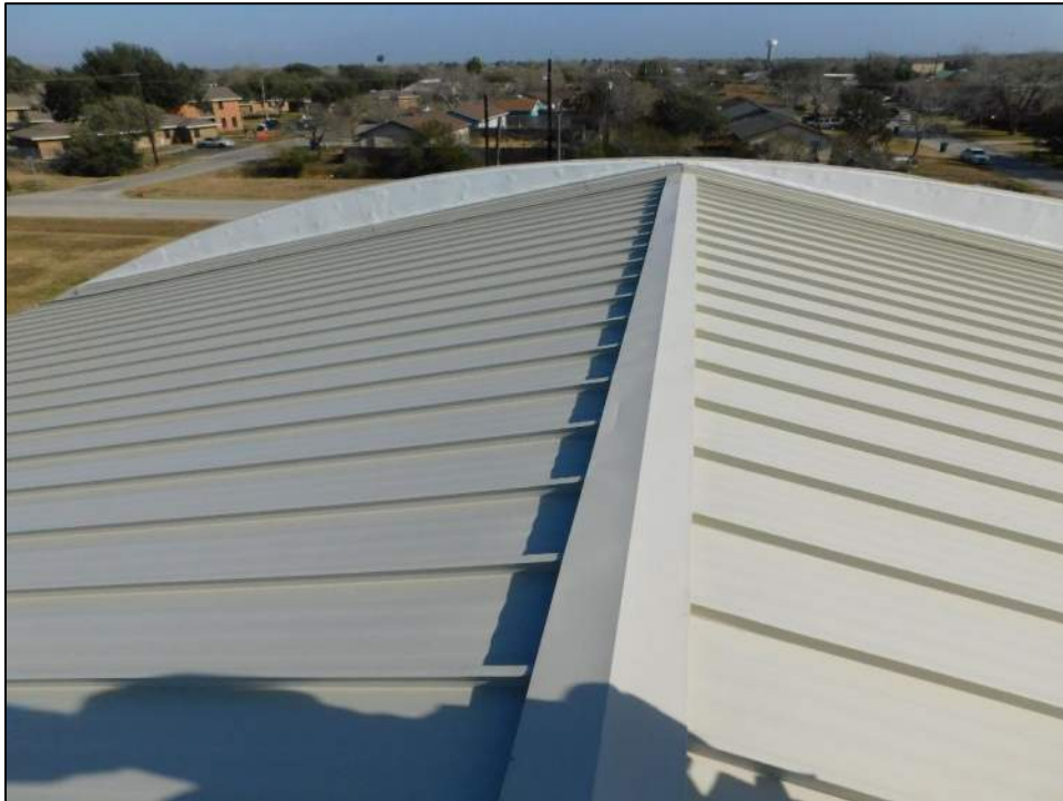
Photo 63: Metal ridge of the fire department building roof remained securely attached.
