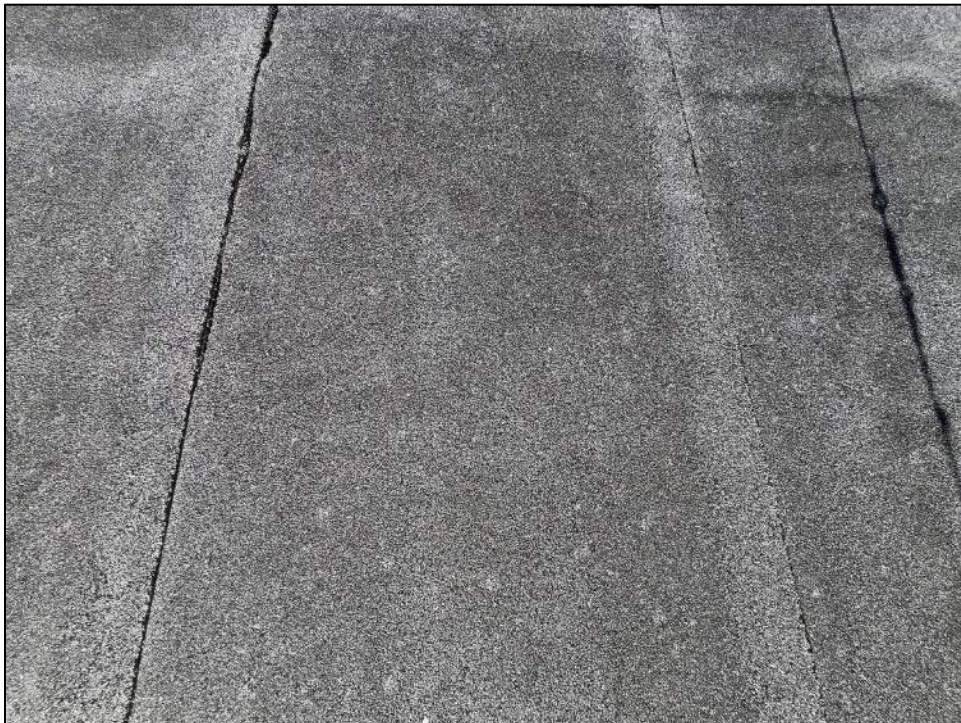
Photo 43: Spatters consistent with recent hail was observed on the algae-covered mod-bit roofing.
