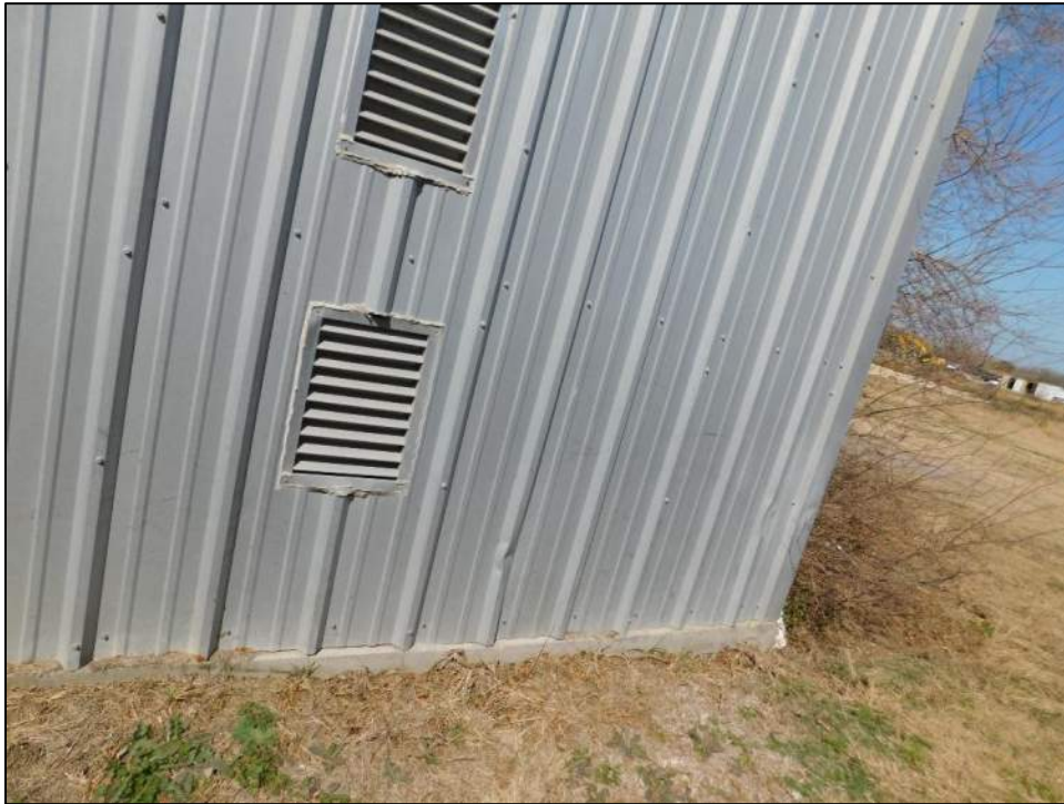
Photo 56: Mechanical dents in lower section of east wall unaffected by hail.
