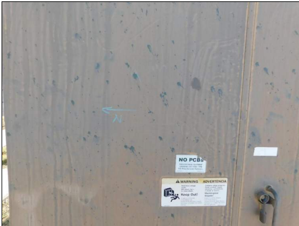
Photo 41: Transformer along rear side of the building exhibited hail spatters consistent with 1.25-inch at maximum size most being under 0.75 inches.
