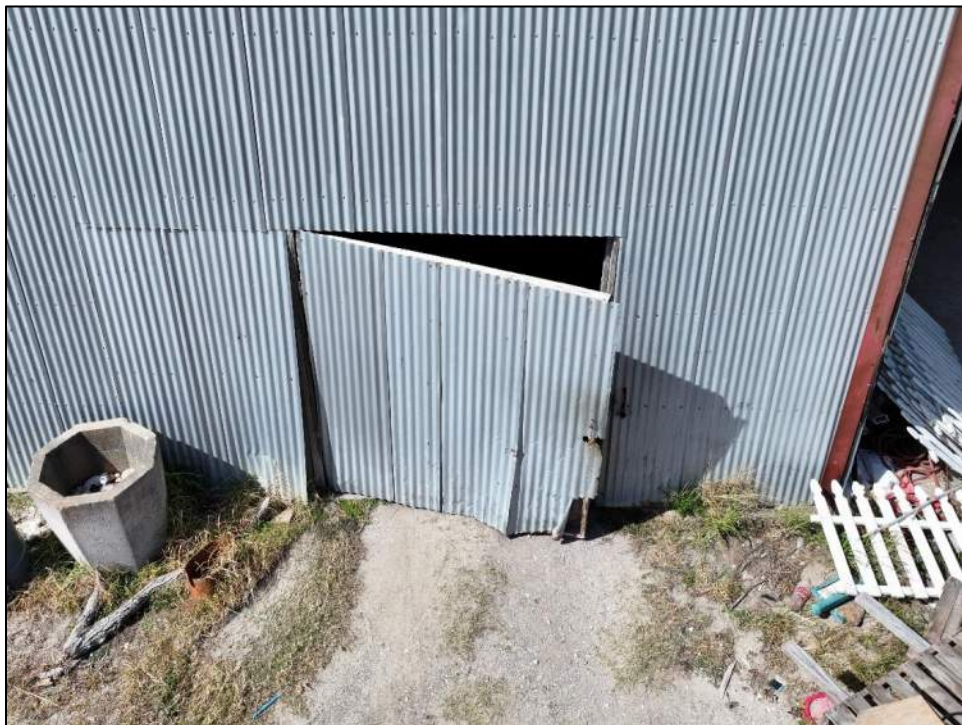
Photo 80: Deformed door of the vehicle storage building.
