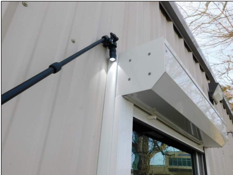
Photo 10: No hail denting was present in the window guard housing.
