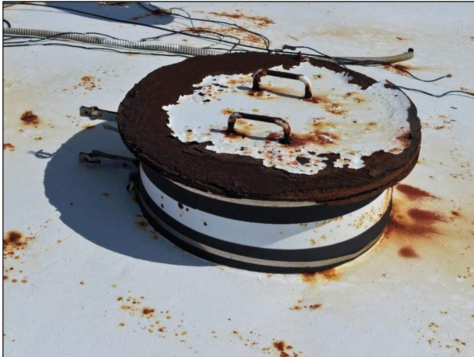
Photo 17: Vent coverings on the top of the tanks were severely corroded.
