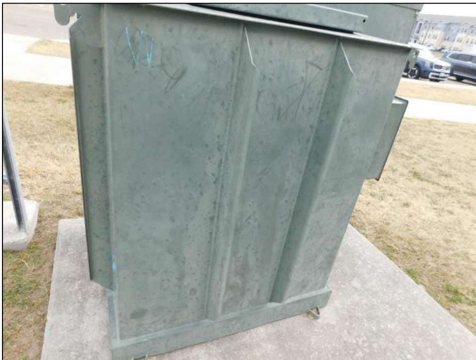
Photo 26: Hail spatters consistent with 0.75- to 1.0-inch hail on west-facing surfaces.
