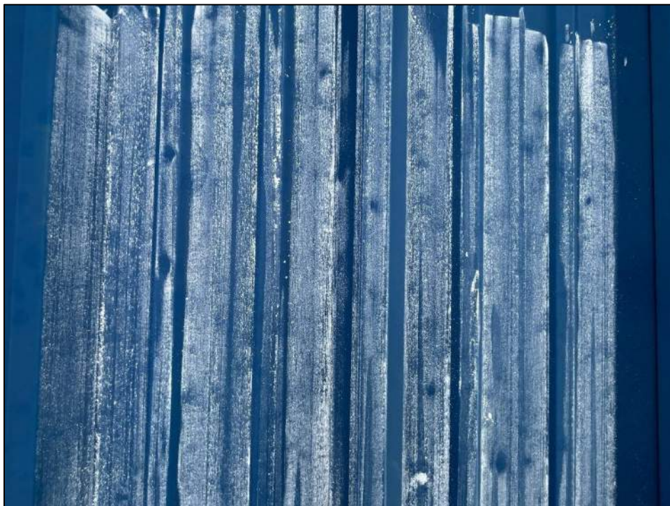
Photo 14: Close-up of the hail denting. The dents were generally shallow with an inner diameter of less than 3/8 inch.
