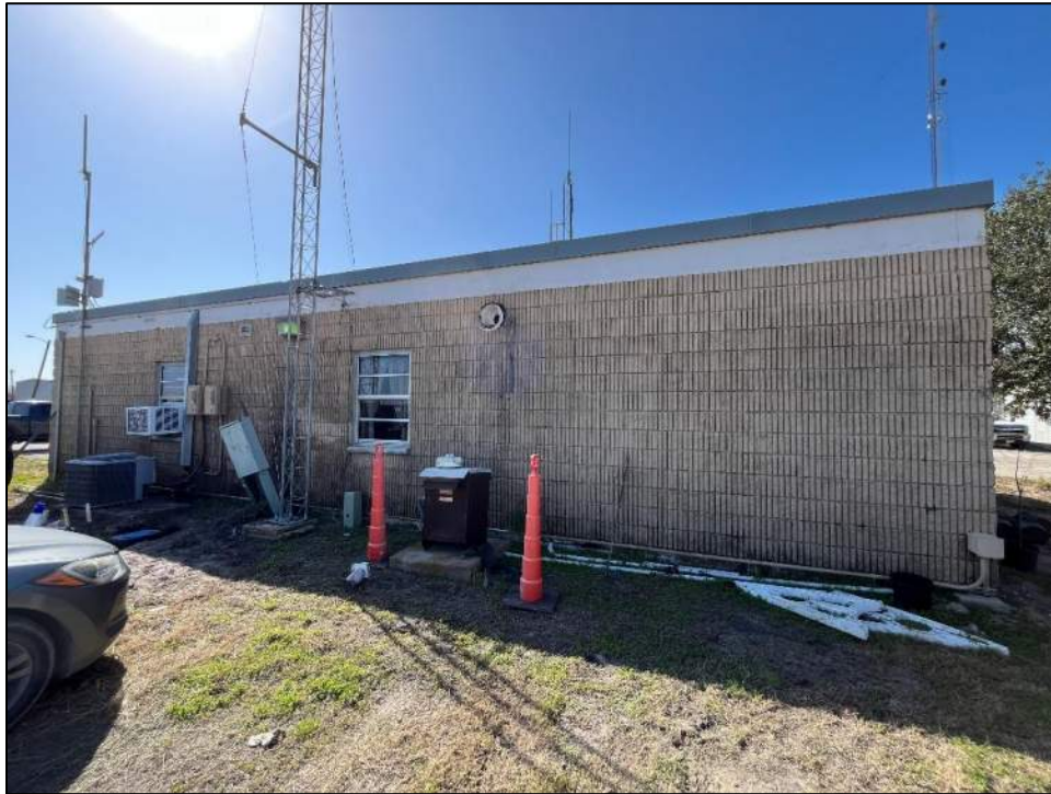
Photo 38: North elevation. Windows remained intact.
