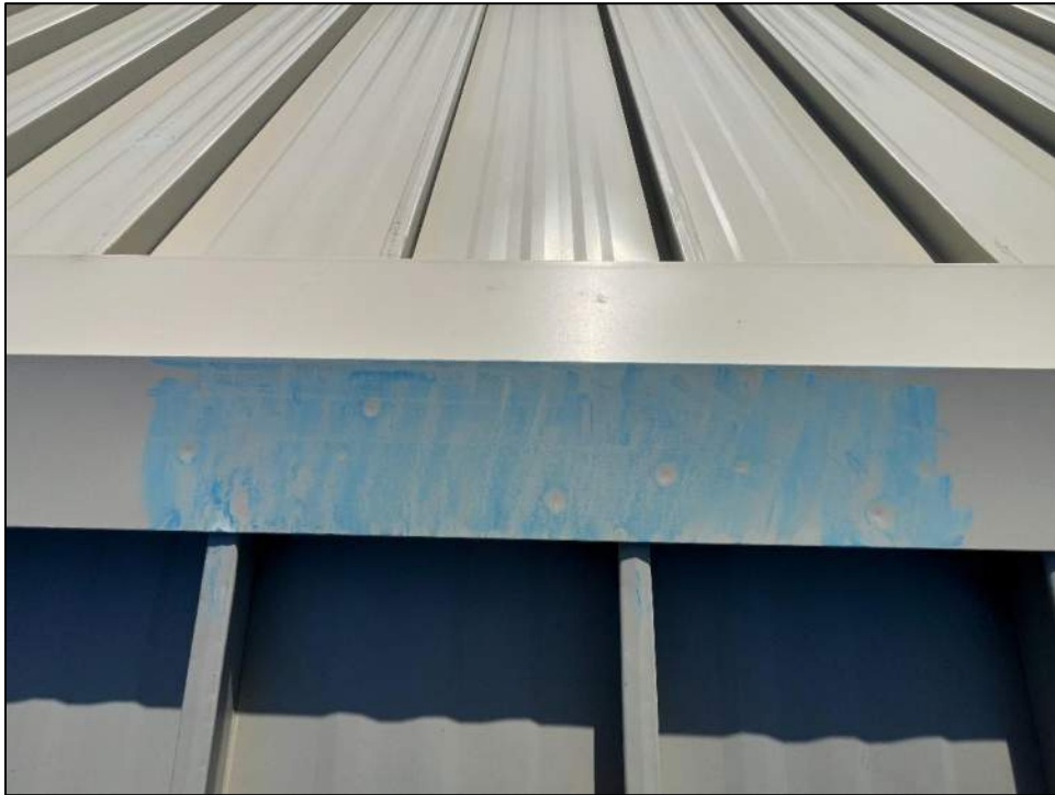
Photo 67: Dented ridge panel above the fire department. No coating disruptions were observed at the dents.
