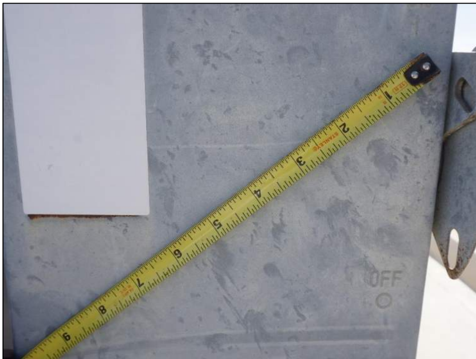
Photo 8: Hail spatters on rooftop units reflect 1-inch hail.
