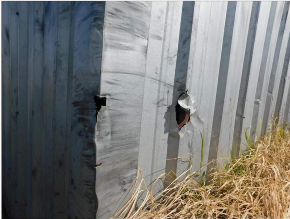
Photo 85: Mechanical damage to south wall (southwest corner) unrelated to hail impact.
