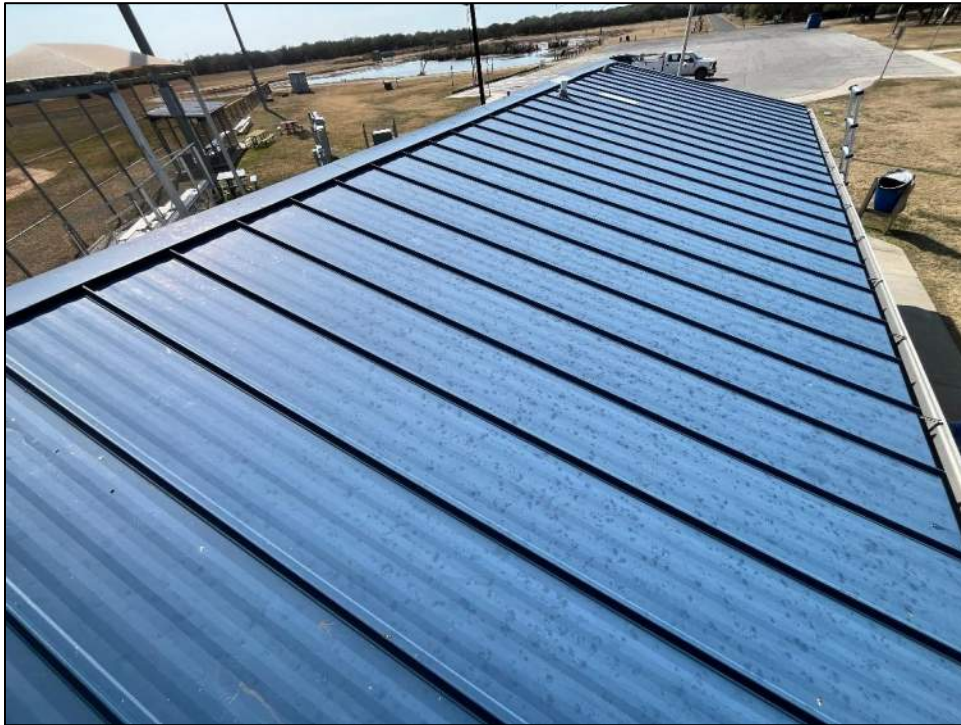
Photo 11: Hail denting and spatters on north slope were more severe than east and south slopes.
