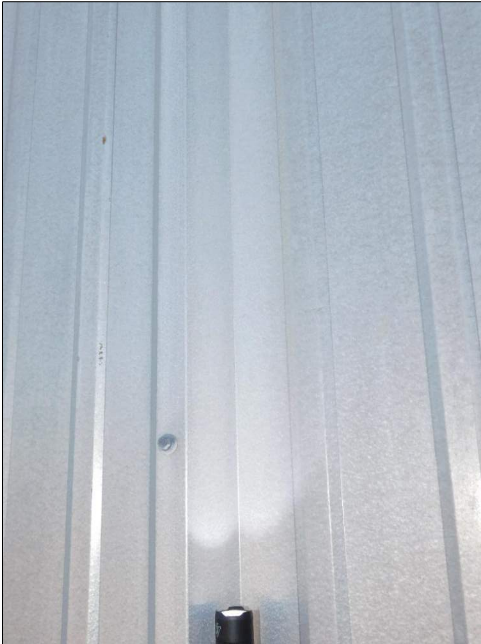
Photo 60: No denting was observed on the north wall.
