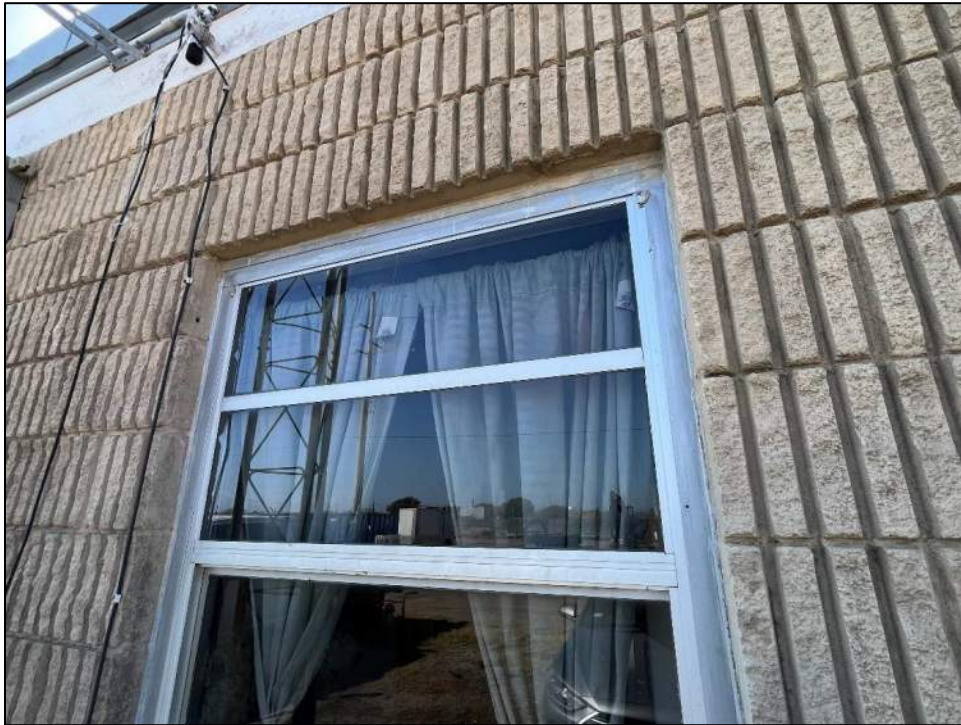
Photo 40: North wall (exposed to direct hail impact) window glazing remained intact.
