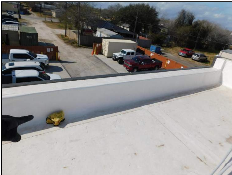
Photo 24: Unsupported PVC membranes at the base of parapets facing the direction of the hail were not punctured dimpled or scuffed.
