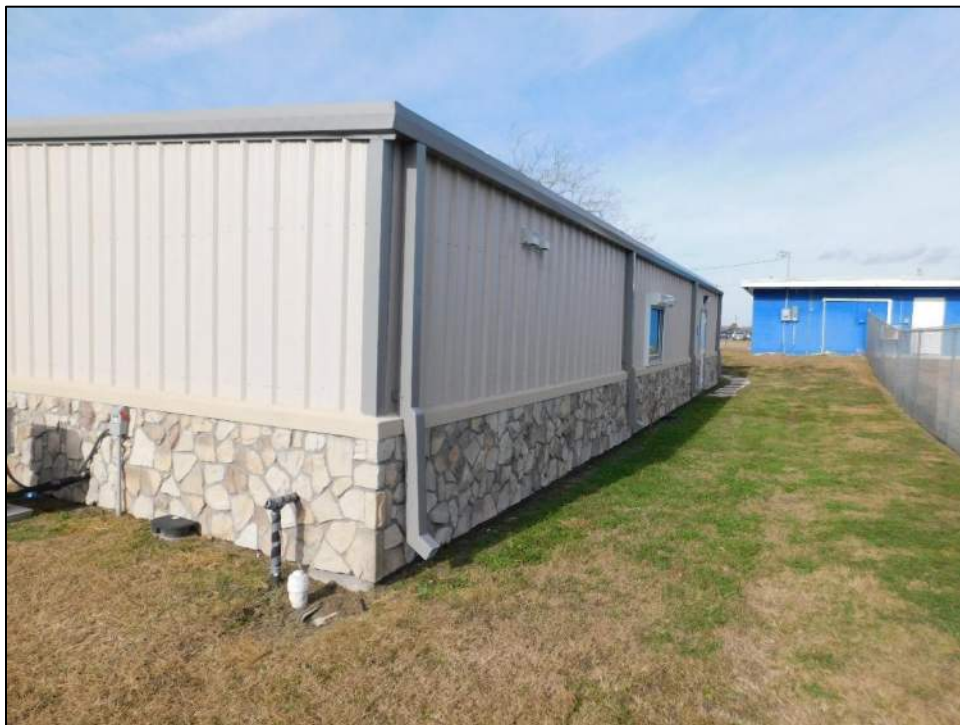
Photo 4: North elevation. Window glazing and door remained intact.
