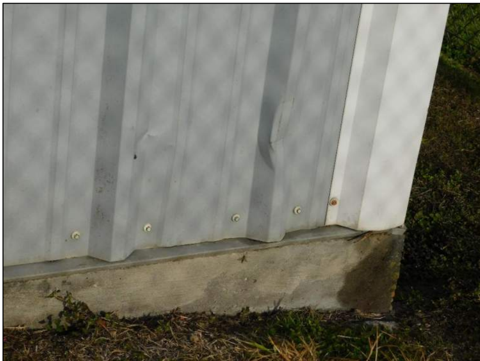
Photo 8: Mechanical damage at east elevation lower section.
