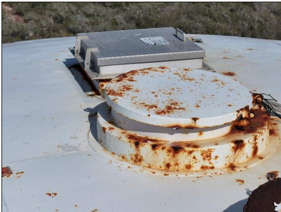
Photo 18: Steel plate vent coverings remained otherwise intact.
