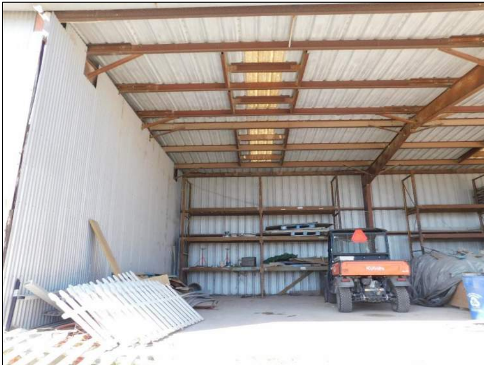
Photo 101: Skylight of the vehicle storage building were not fractured.
