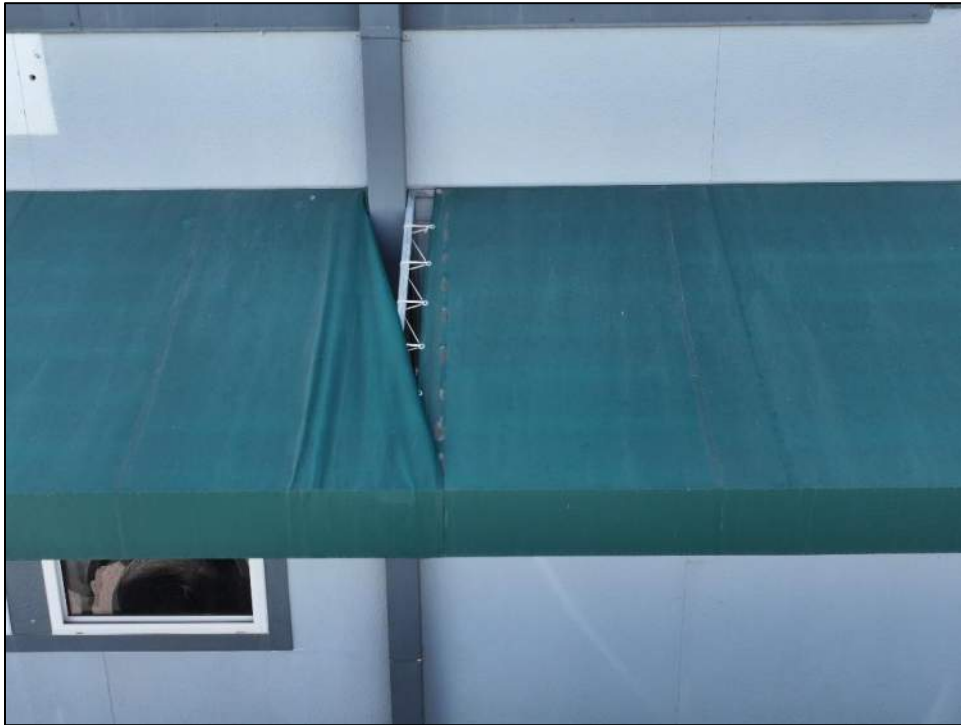
Photo 5: Pre-existing awning separation at a downspout.
