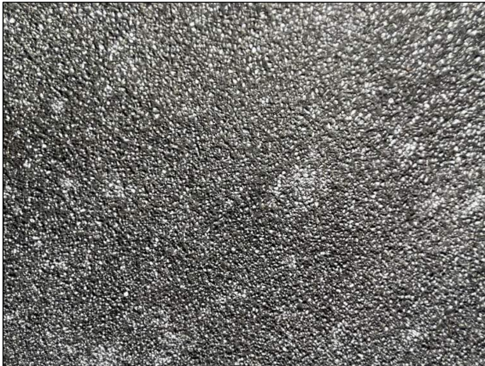
Photo 47: No granule displacement was observed at the largest hail spatters.
