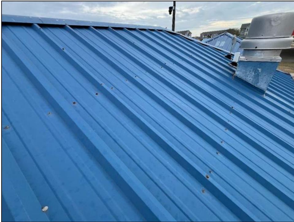
Photo 68: West slope. Note widespread fastener corrosion.
