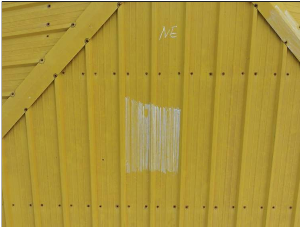
Photo 80: North slope. Note fastener corrosion.
