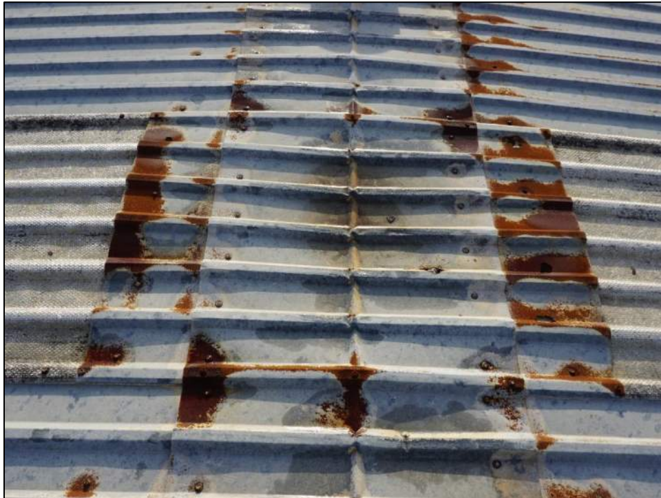
Photo 49: Buckled ridge cap at east end of ridge unrelated to hail effects.
