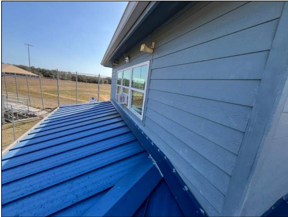
Photo 23: East-facing walls and windows remained absent of hail spatters.
