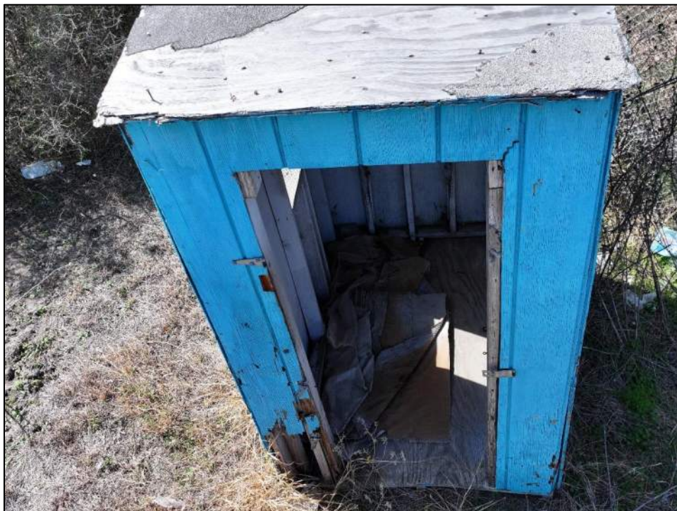
Photo 78: A deteriorated shed located to the south of the vehicle storage building.
