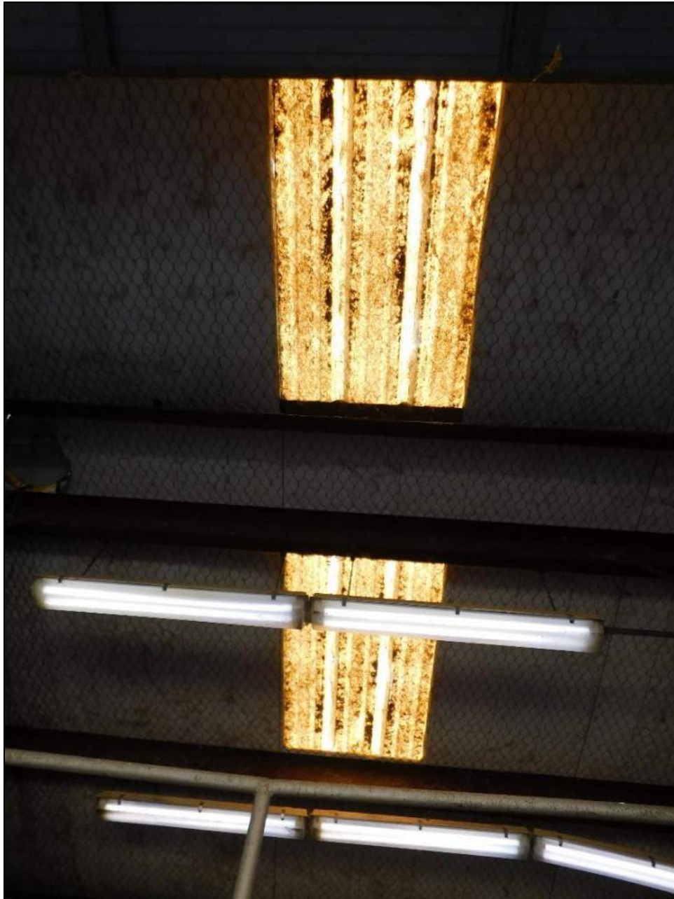
Photo 31: Skylight panels exhibited deterioration and isolated punctures consistent with hail impact.
