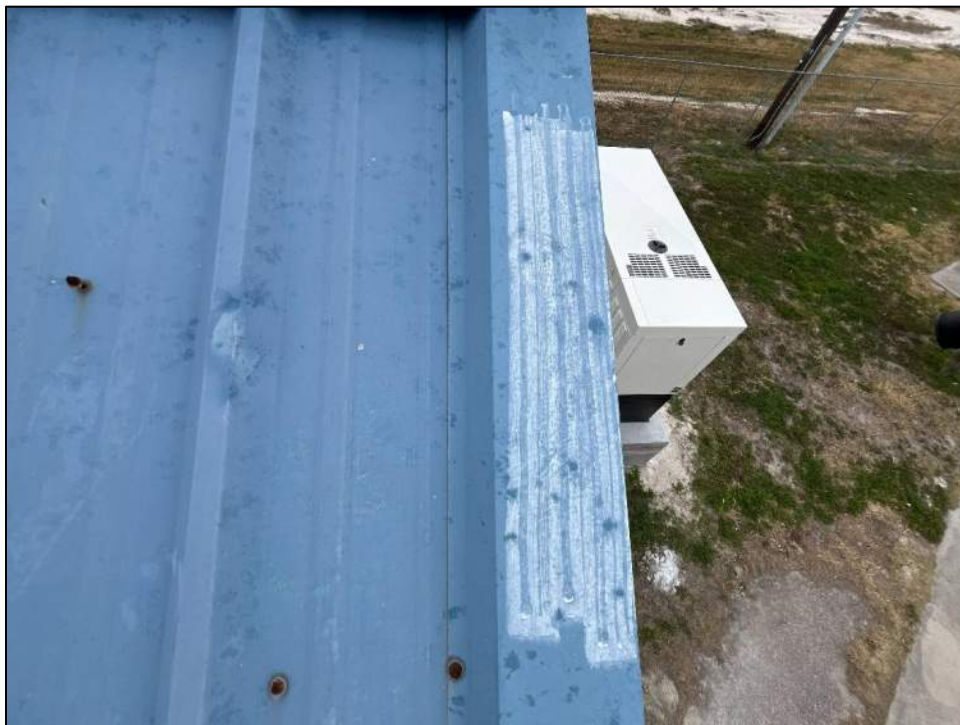
Photo 18: Hail denting on west gable rake closure metal.
