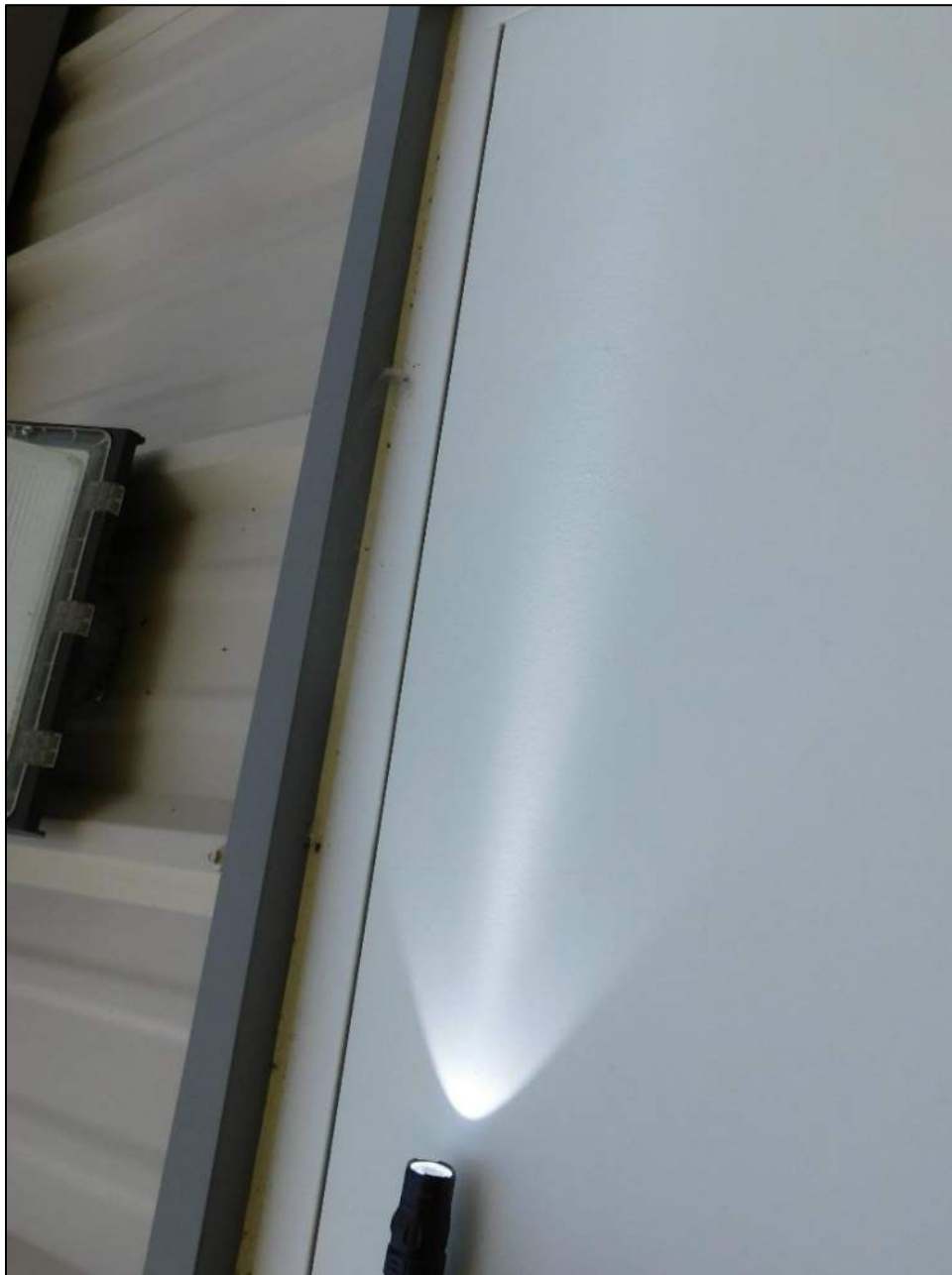
Photo 15: No hail denting observed on the rear door.
