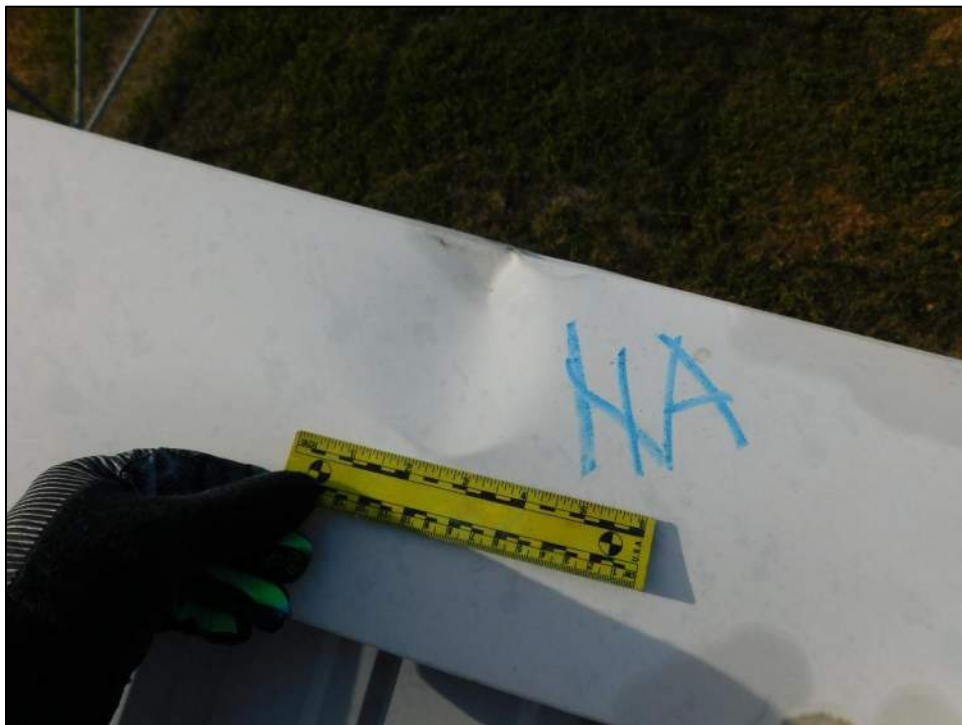
Photo 18: Mechanical damage to the front closure metal irrelevant to hail impact.
