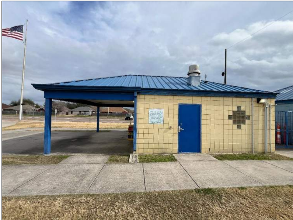
Photo 62: West elevation. No glass masonry units were fractured.
