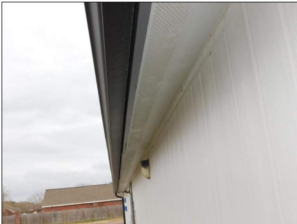
Photo 6: Dents were visible in the bottom of the front wall gutters.
