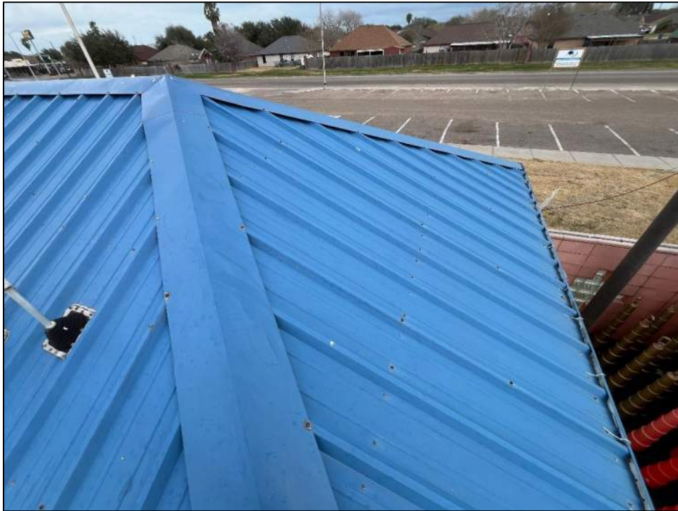
Photo 70: South slope. Note widespread fastener corrosion.
