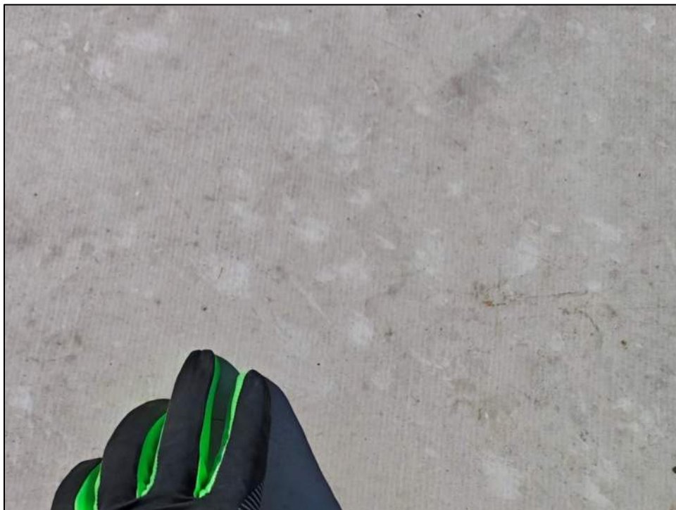
Photo 28: Largest hail spatter on the PVC roofing was 1-inch maximum base width.
