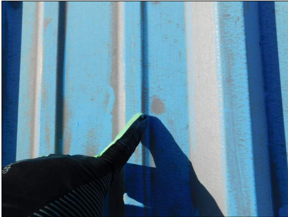
Photo 105: Hail denting observed on the galvalume metal roof decking had maximum inner diameter of less than 1/2 inch.
