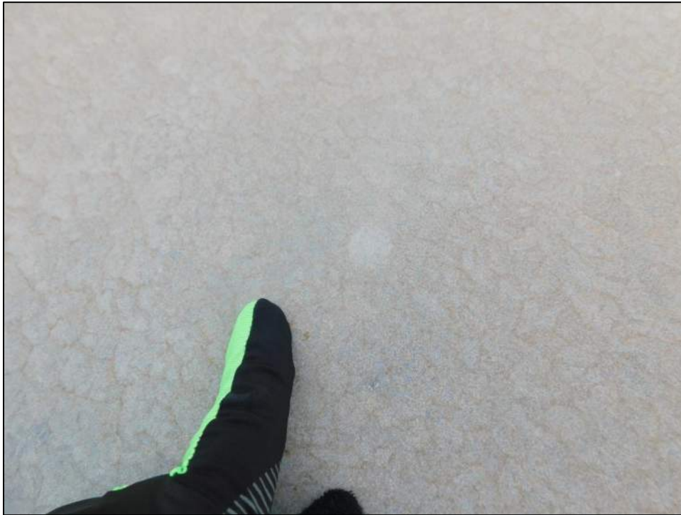
Photo 70: No hail impact mark was discernible on the tank roof.
