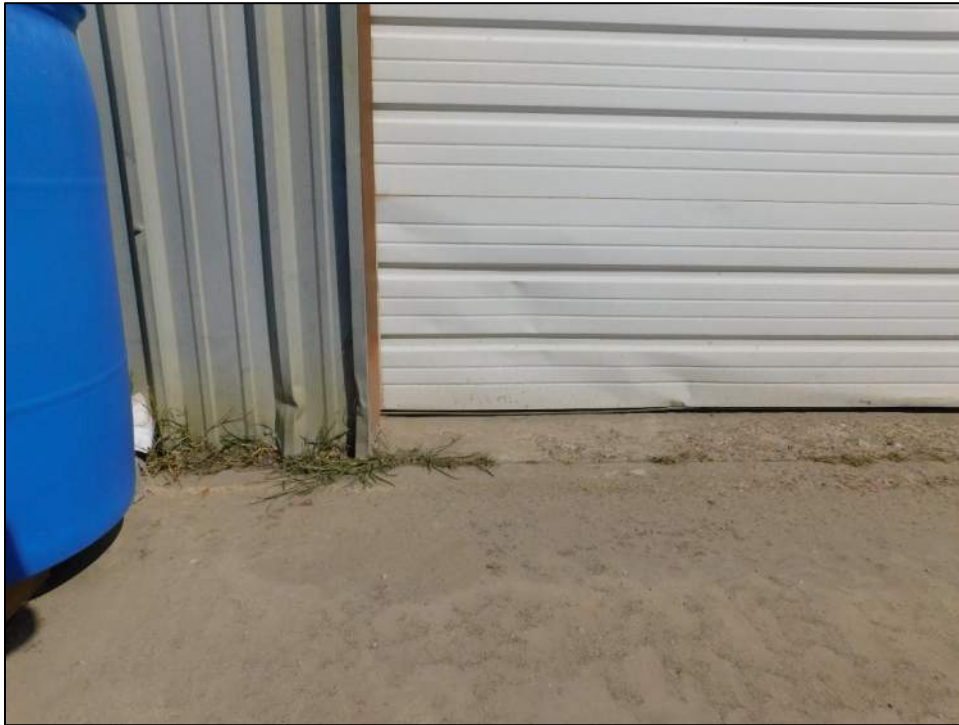
Photo 63: mechanically dented lower section of roll-up door at front (south) wall unaffected by hail.
