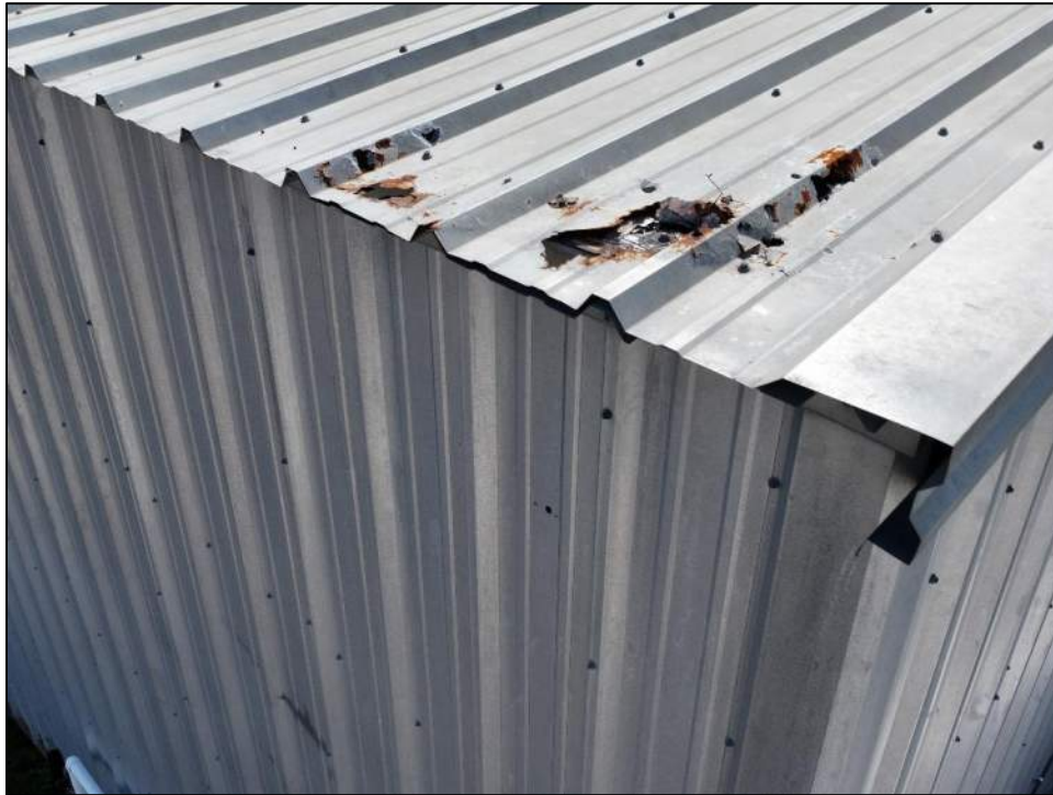
Photo 54: Corroded deck typically found at the four corners of the roof.
