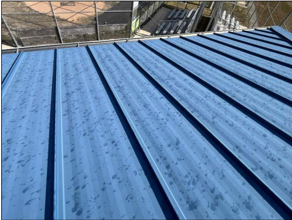
Photo 31: Widespread hail spatters observed on the high roof.
