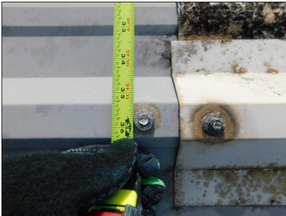
Photo 24: Corroded deck fasteners (typical condition).
