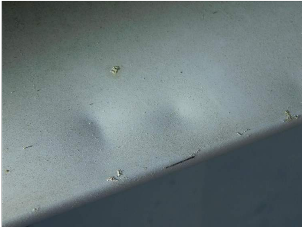
Photo 15: No coating disruption at the dents in the front wall aluminum shutters.
