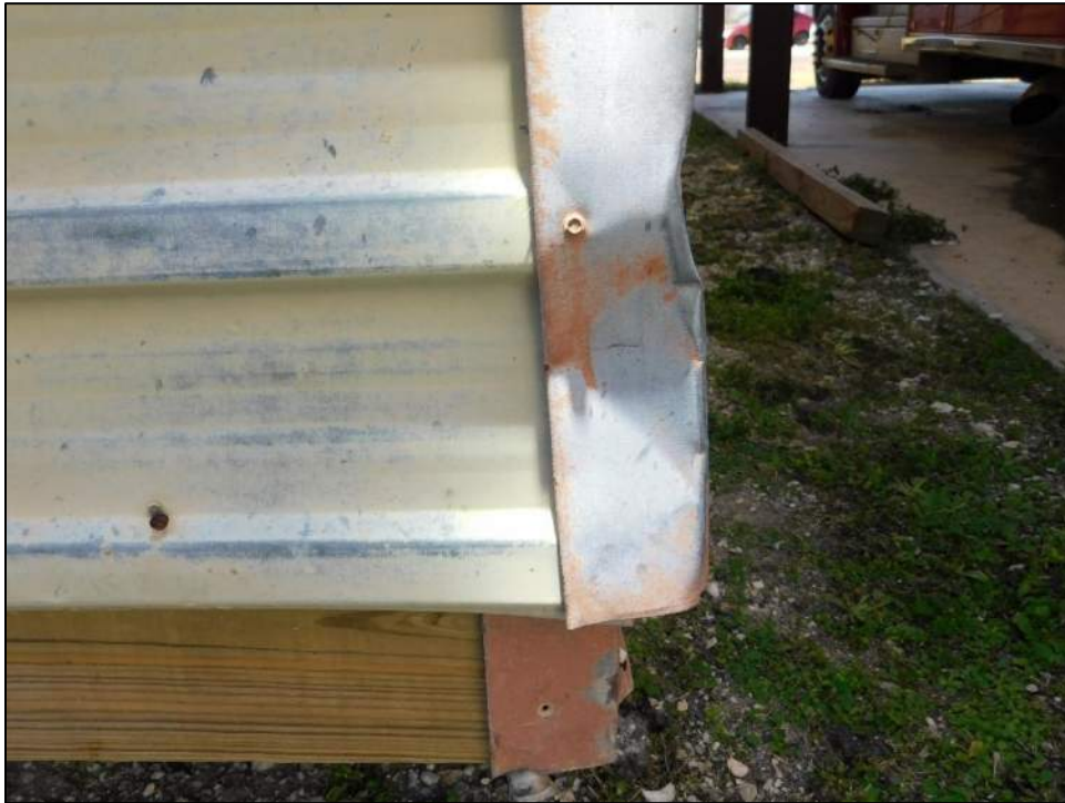
Photo 96: Crushed edge trim at northwest corner of the storage building that was inconsistent with hail impact.
