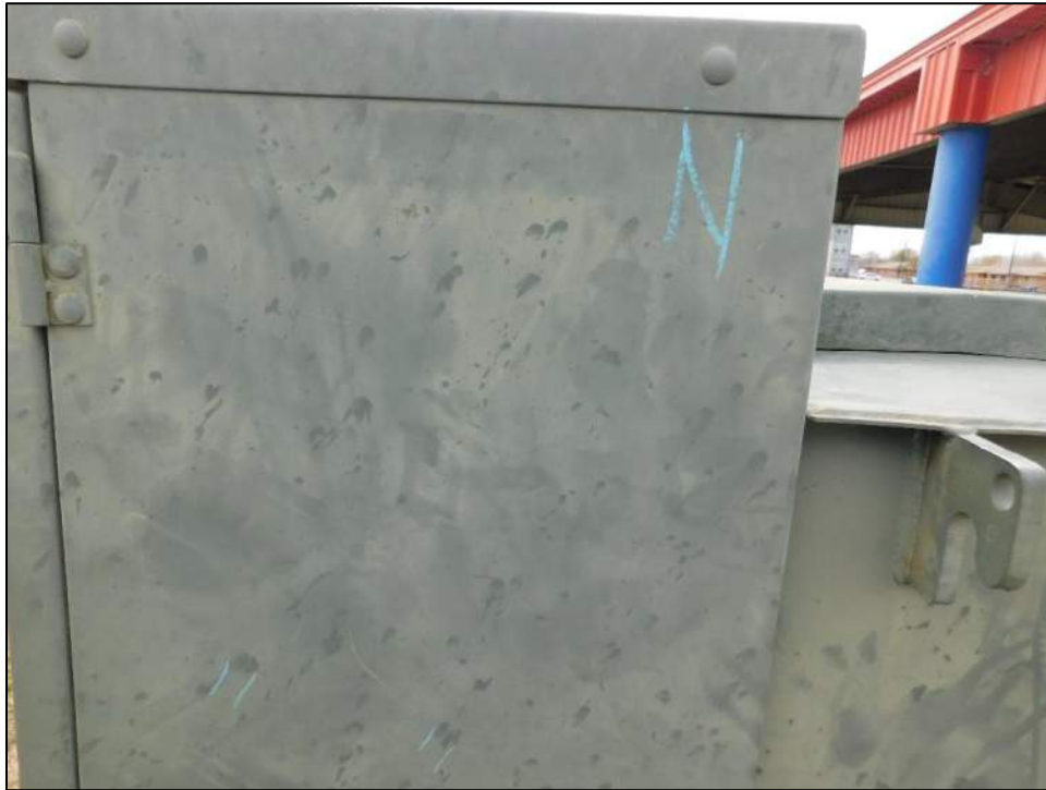
Photo 27: Hail spatters consistent with 0.75- to 1.0-inch hail on north-facing surfaces.
