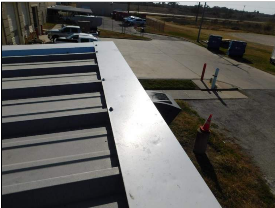
Photo 102: Dented closure along south roof eave consistent with hail impact.
