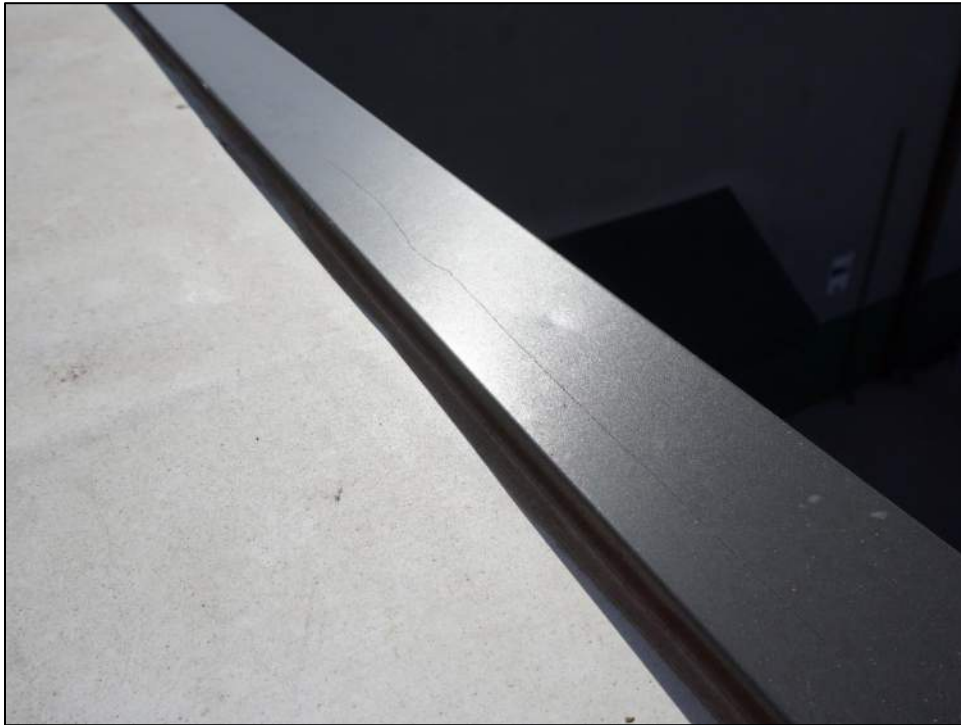
Photo 21: Cosmetic denting in coping metal above rear parapet wall.
