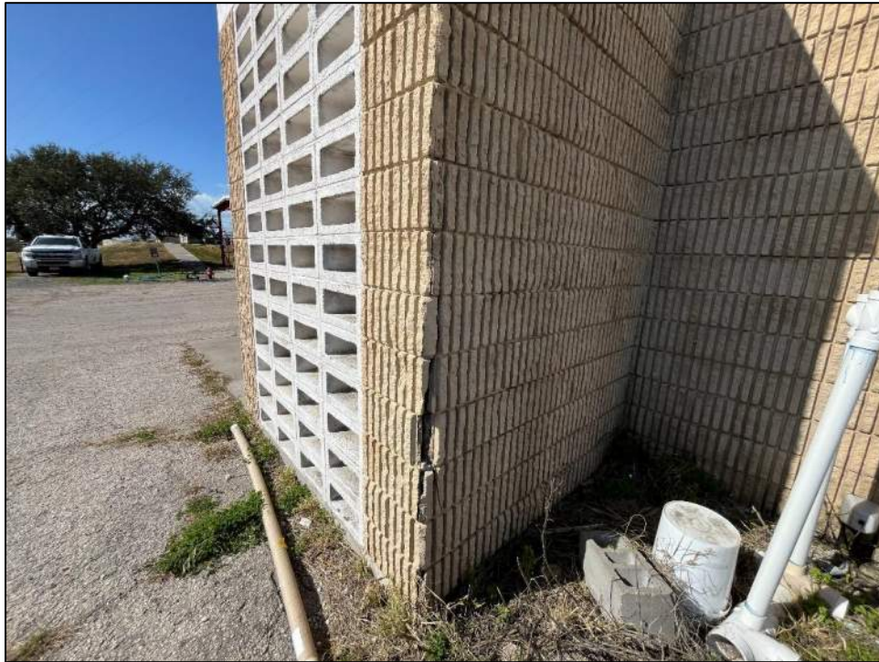
Photo 34: Cracked masonry veneer irrelevant to hail.
