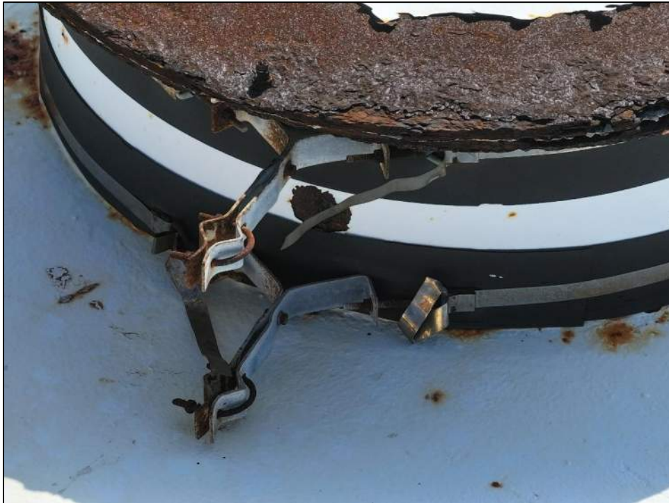
Photo 25: Close-up of corroded vent cover steel plates unrelated to hail effects.
