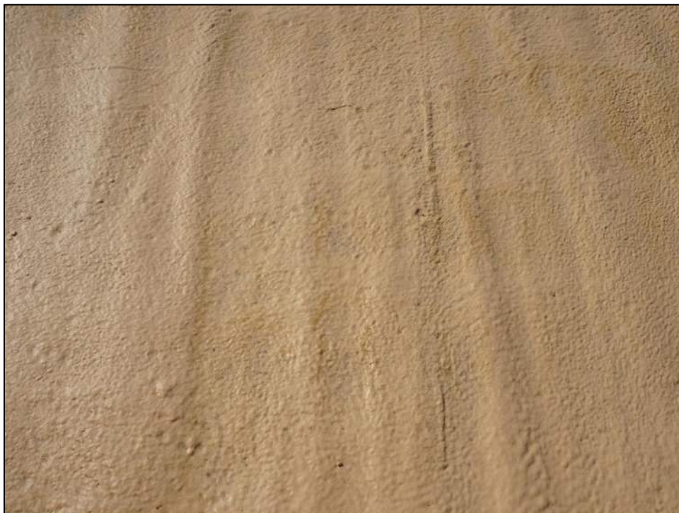
Photo 10: Nearby SPF coating exhibited no widespread coating fractures.
