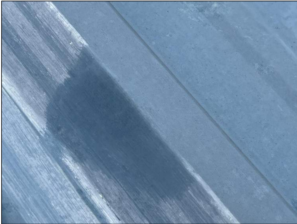
Photo 26: No coating disruption at hail spatters on south slope.
