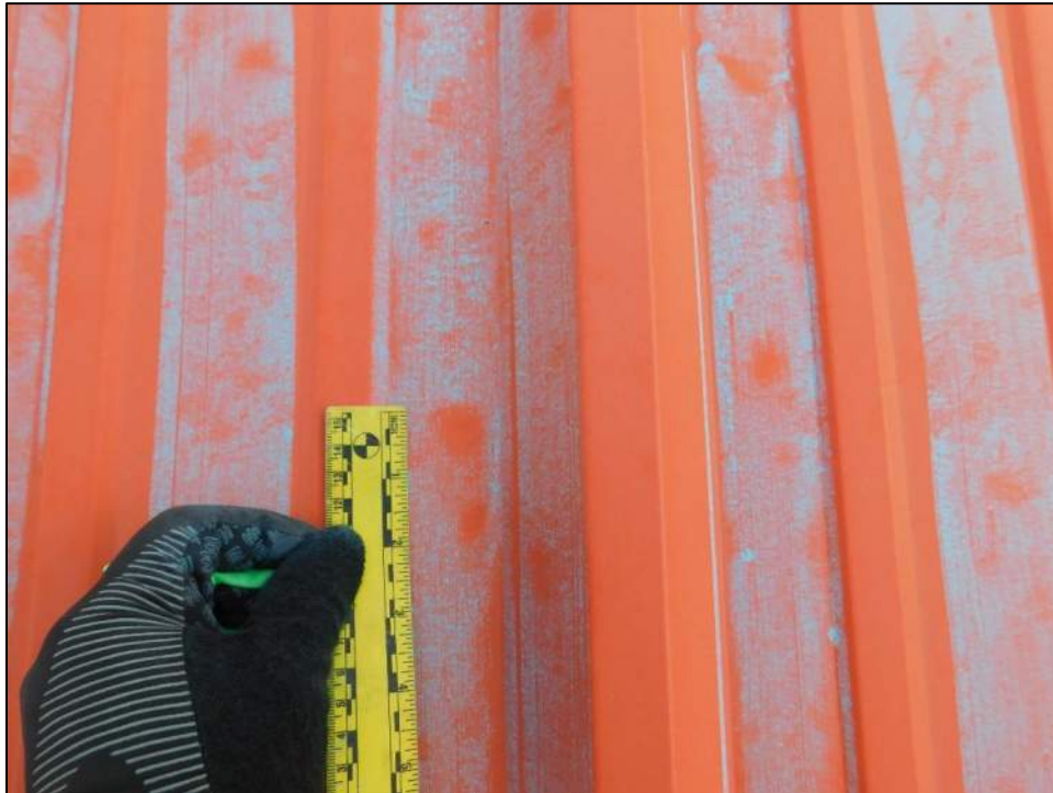
Photo 46: West slope indentations were similarly 1/2-inch in maximum inner diameter with coating disruptions observed.
