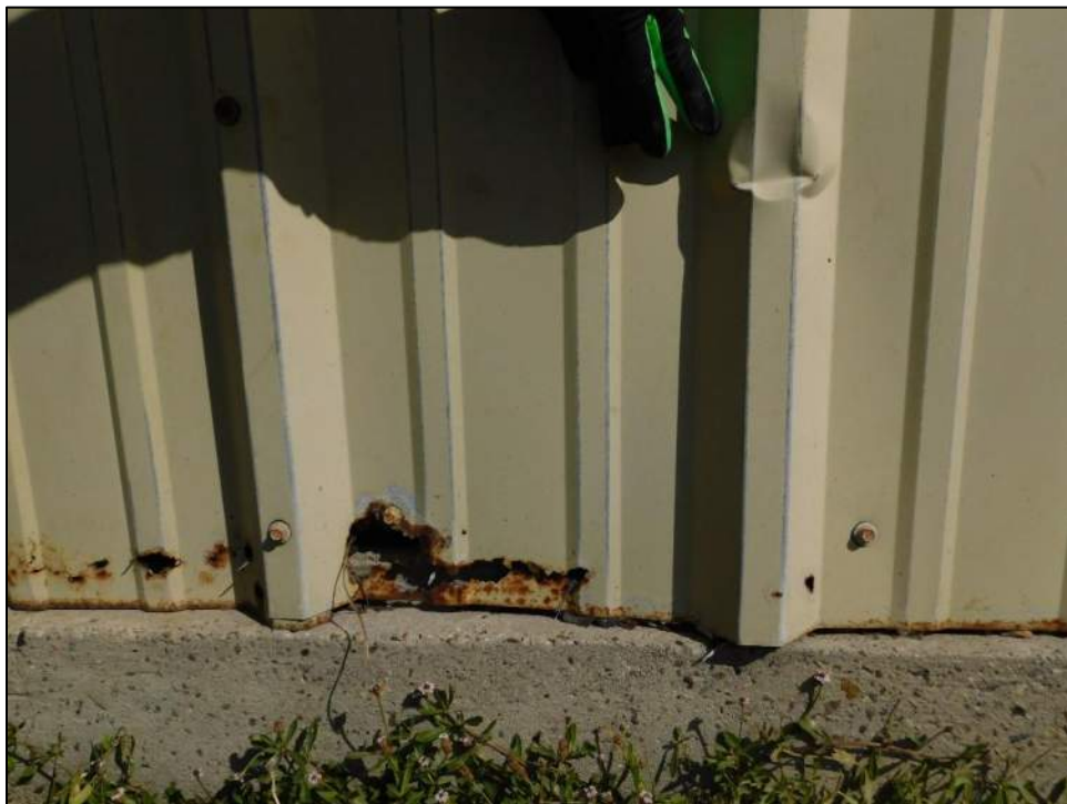
Photo 15: Wall panel mechanical denting and corrosion at the bottom of the south wall.
