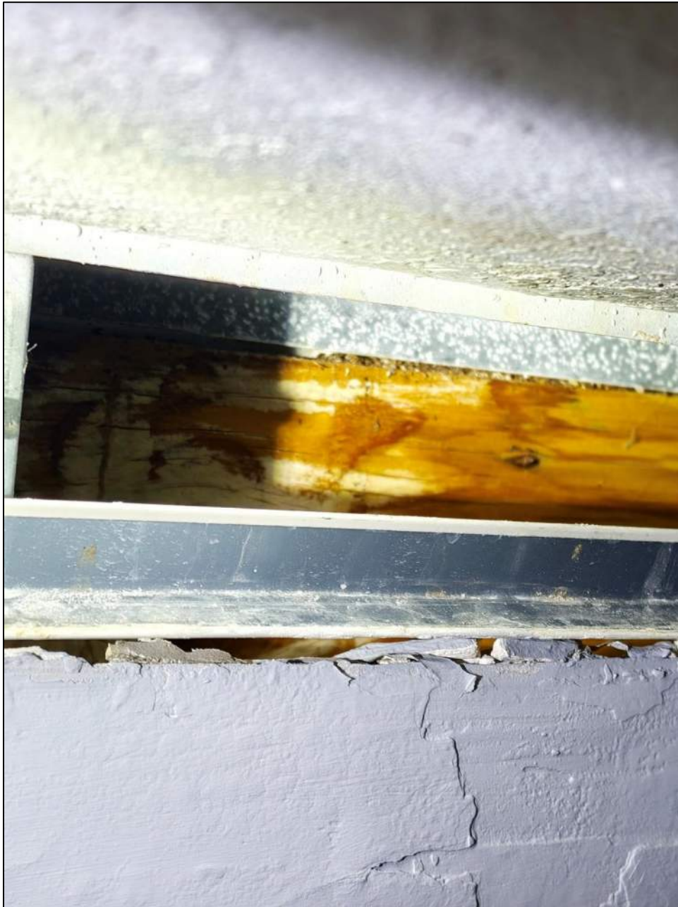
Photo 39: Plywood wall sheathing above the stained ceiling tile were darkly stained.
