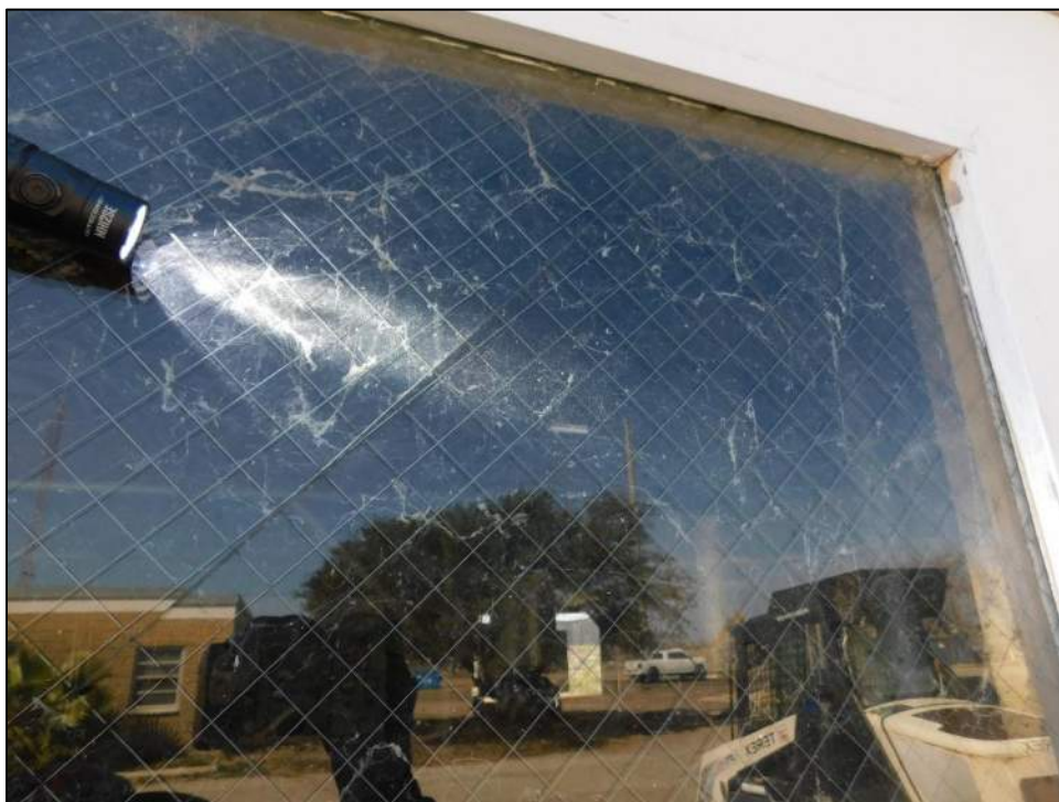
Photo 6: Cracked door glazing showed soiling along the crack edges.
