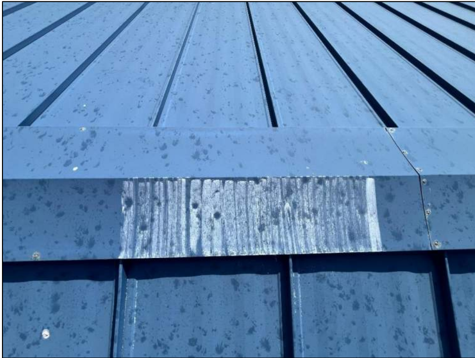
Photo 17: Hail denting was similarly observed along ridge caps.
