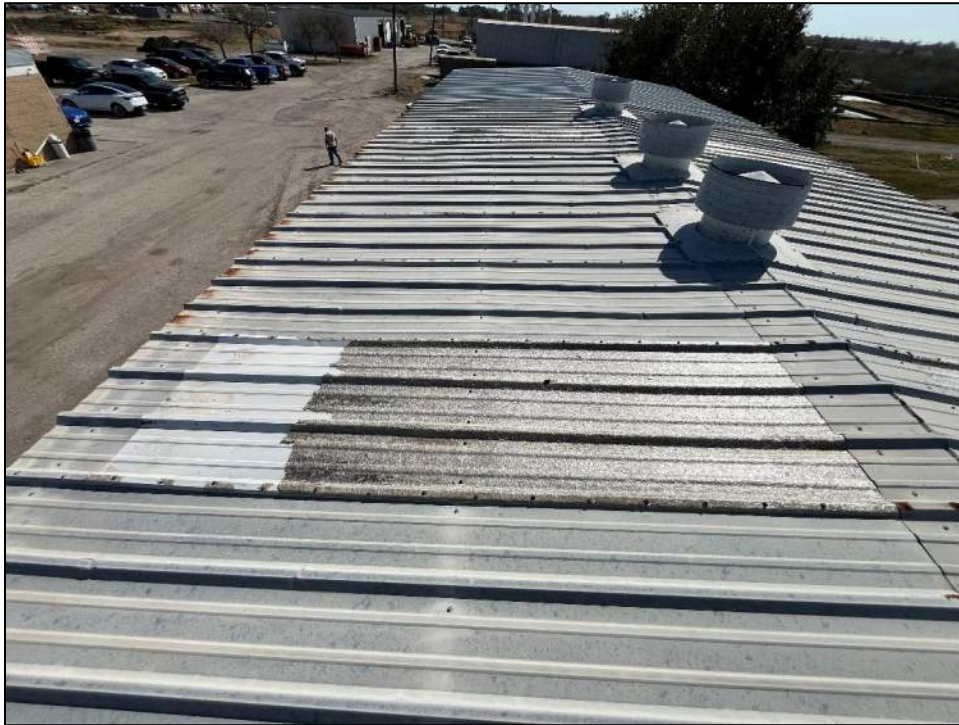
Photo 24: Deteriorated skylight panels were underlaid with metal panels.
