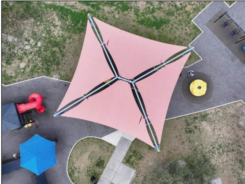
Photo 97: Top view of the HDPE fabric canopy. Note three tears at anchorage points.
