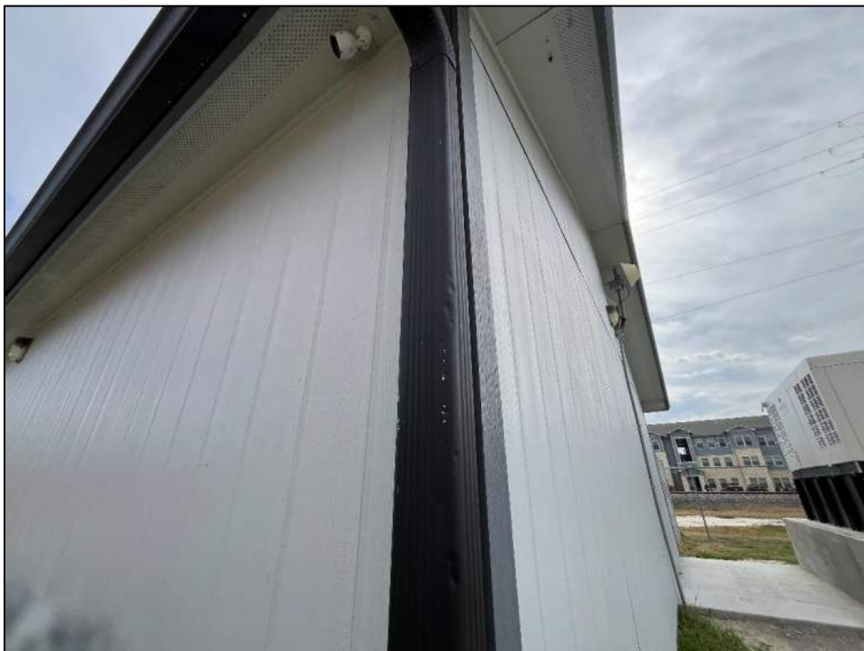
Photo 10: dented downspout at northwest building corner.
