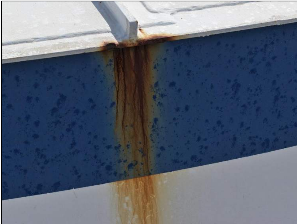
Photo 9: Close-up of West-facing tank wall with hail spatter marks consistent with approximately 1-inch hail. Note steel corrosion.
