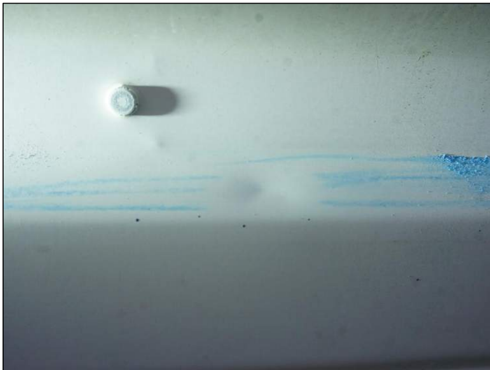
Photo 42: Hail denting on the roll-up door was unaccompanied by coating disruptions.
