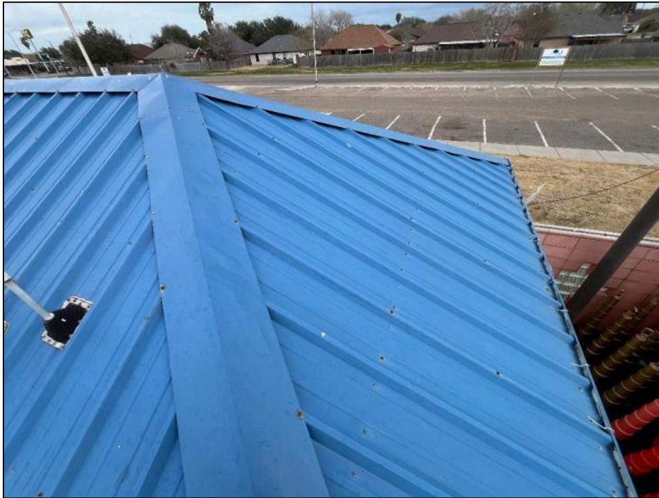
Photo 70: South slope. Note widespread fastener corrosion.
