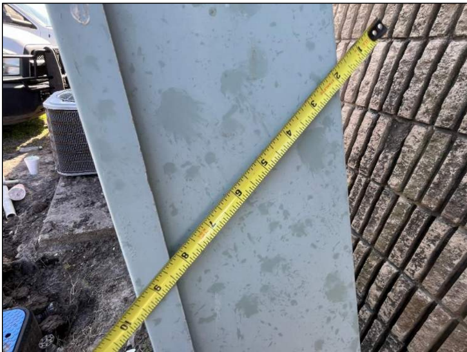
Photo 41: Largest hail spatter on a electrical box on the north wall (west surface) measured 1.0 inches in base width.
