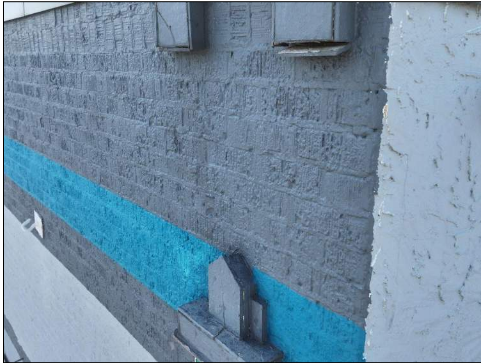
Photo 3: North wall. Separated roof decorative feature was a pre-existing condition.
