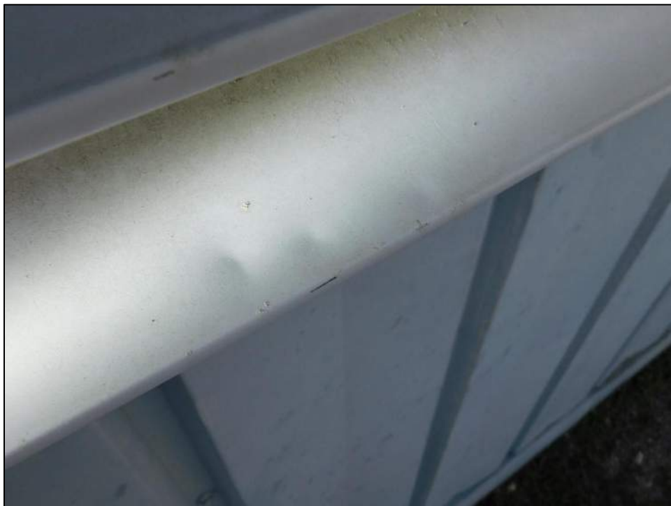
Photo 14: Dents in front elevation aluminum shutters consistent with hail impact.
