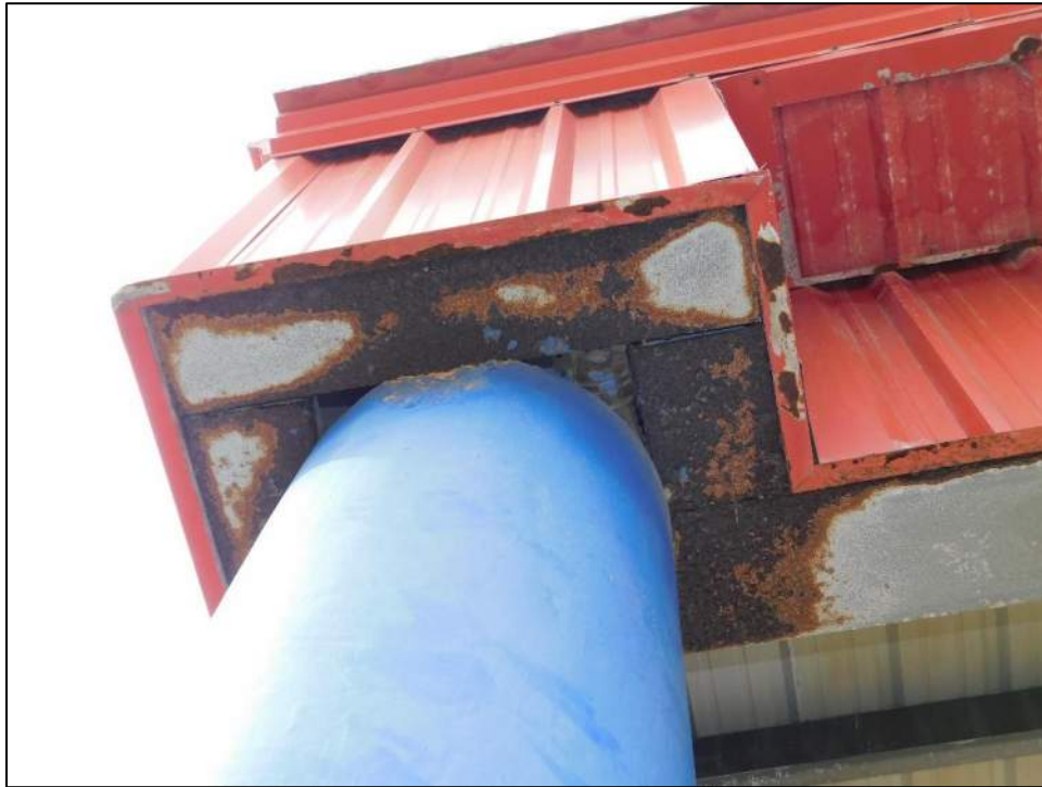
Photo 19: Typical corrosion of metal soffit above concrete columns beneath the sports court roof.
