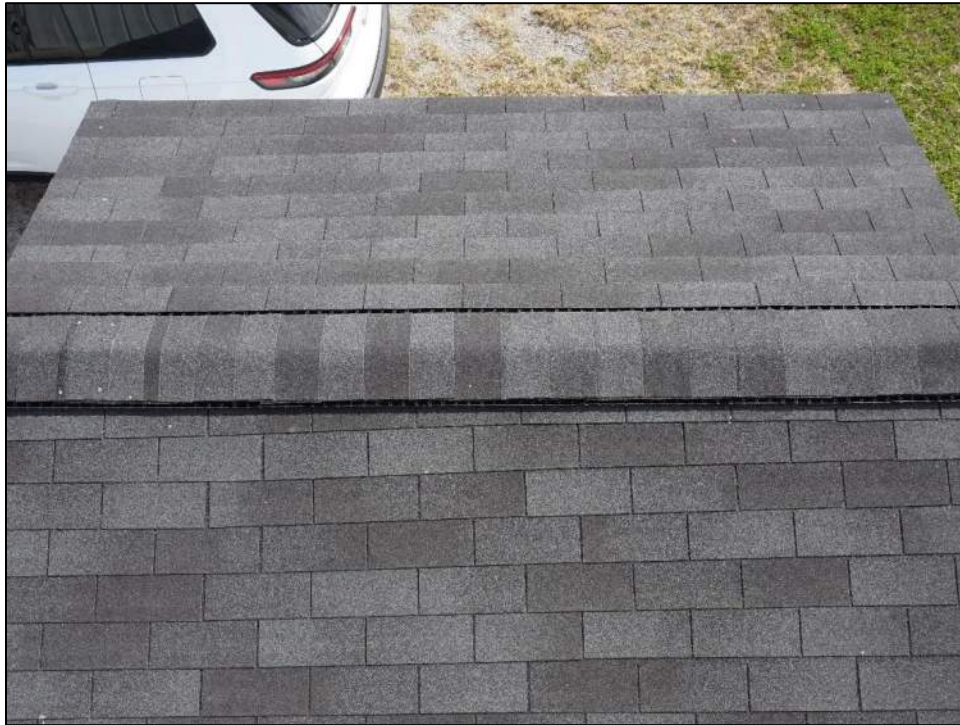
Photo 27: 3-Tabs shingles covering the tool shed to the east side of the building did not exhibit hail impact fractures or visible blemishes.
