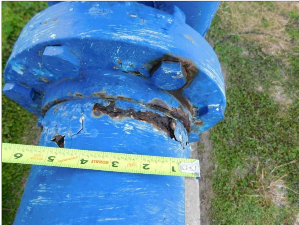
Photo 68: Closer view of typical corrosion at pipe flanges and connections.
