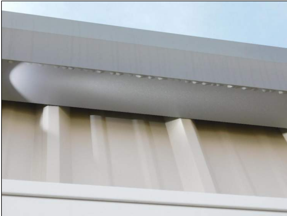
Photo 18: No indentations were observed at the bottom of the rear gutter.
