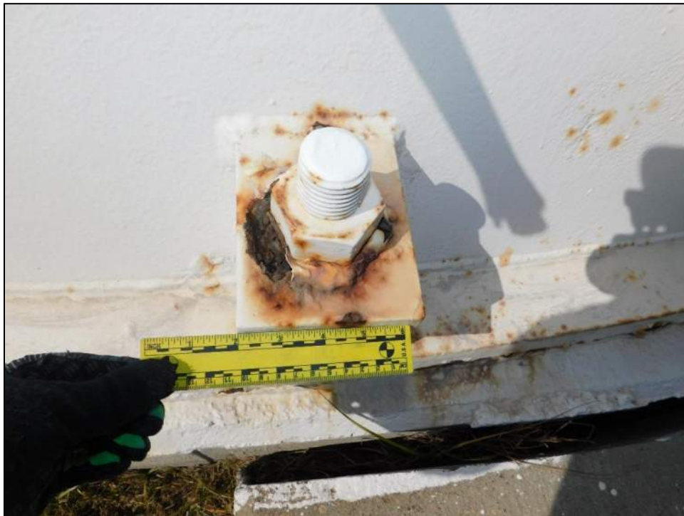
Photo 11: Typical view of corroded anchor plate.
