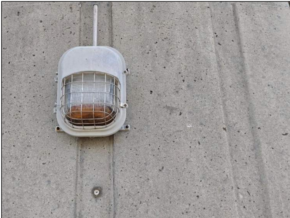
Photo 19: West-facing light fixture were not shattered.
