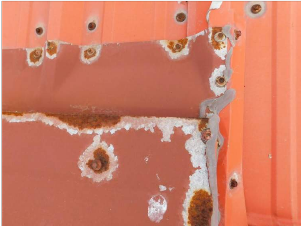
Photo 36: Widespread steel corrosion along other ridge vents.
