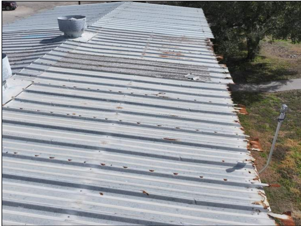
Photo 22: South slope overview. Note severe edge corrosion.
