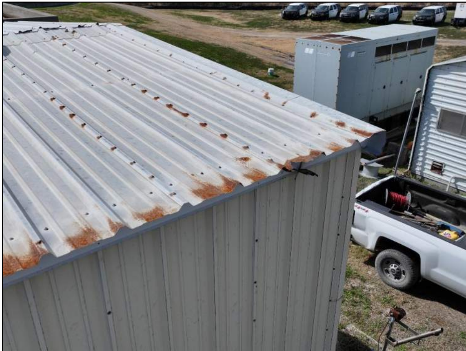
Photo 19: typical roof edge corrosion.
