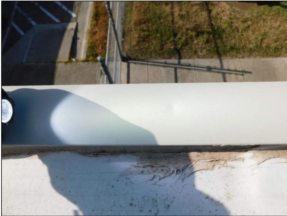
Photo 53: Metal coping along the top of the parapets exhibited slight hail denting absent of coating disruptions.
