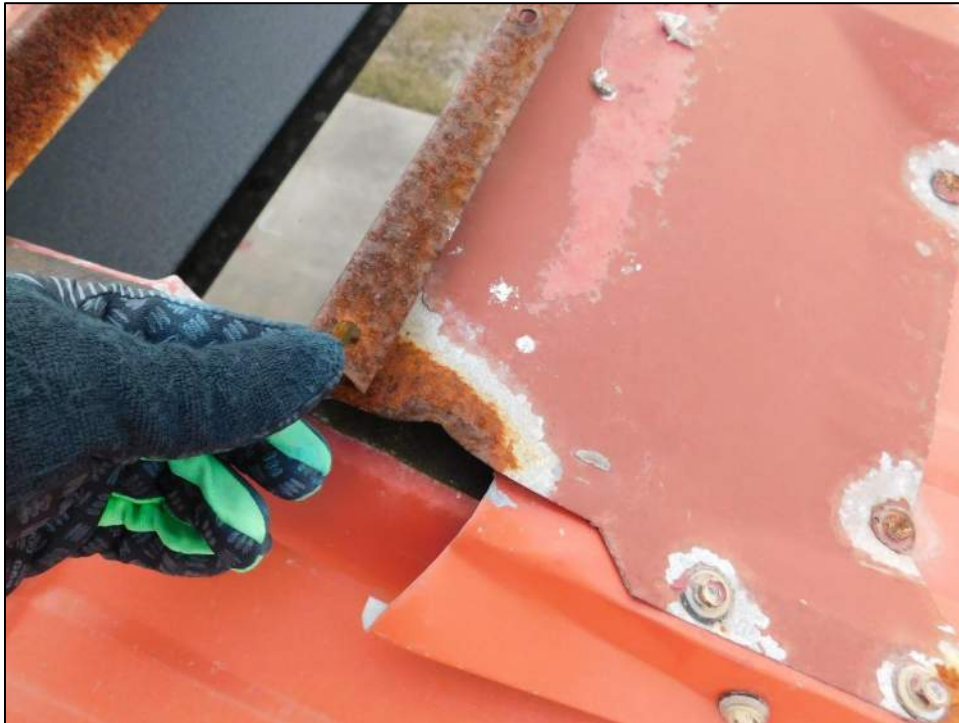
Photo 34: Corroded ridge vent curb.
