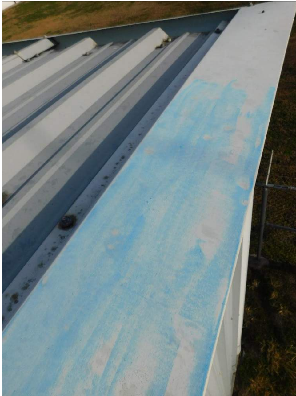
Photo 12: Hail denting on the west rake closure metal.
