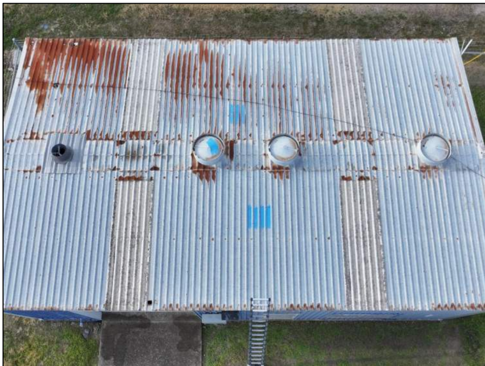
Photo 28: Roof overview. The missing ridge vent cover on the east side (left in the picture) was an existing condition since 2017.
