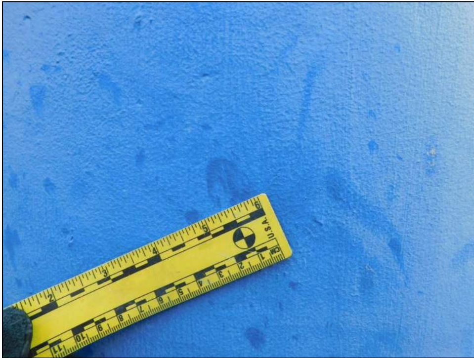
Photo 31: Hail spatters consistent with 0.75- to 1.0-inch hail on west-facing concrete column surface.
