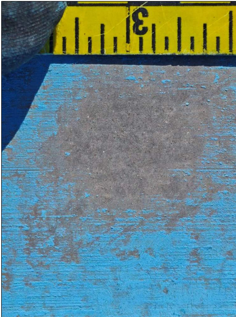
Photo 117: No coating disruptions were observed at the hail dents.
