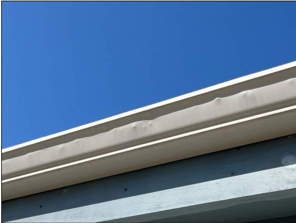
Photo 7: Close-up of the hail denting to the gutter walls.
