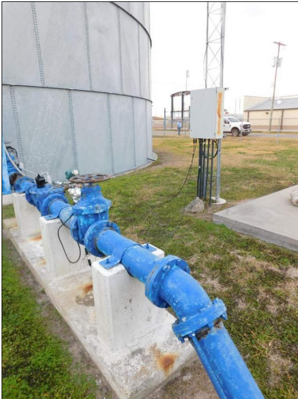
Photo 67: Tank pipe exhibited corrosion.
