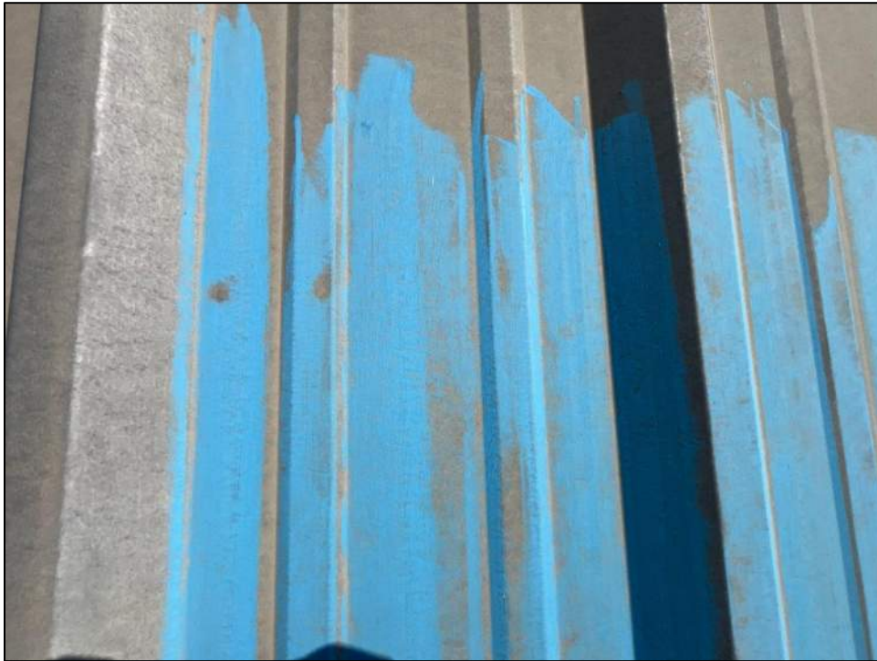
Photo 95: Hail denting in the roofing panels had a inner diameter of less than 3/8 inch.
