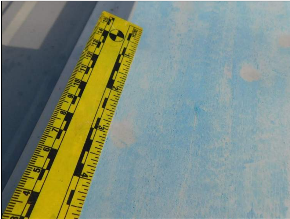
Photo 13: Dents on west rake closure metal has inner diameter less than 3/8 inch.
