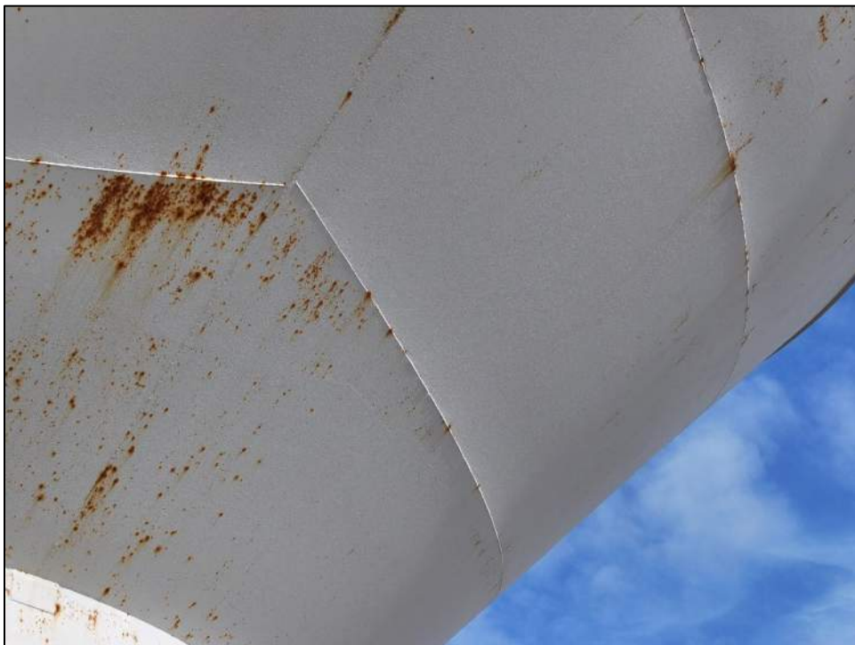
Photo 12: Rusting at surfaces of tank neck wall.
