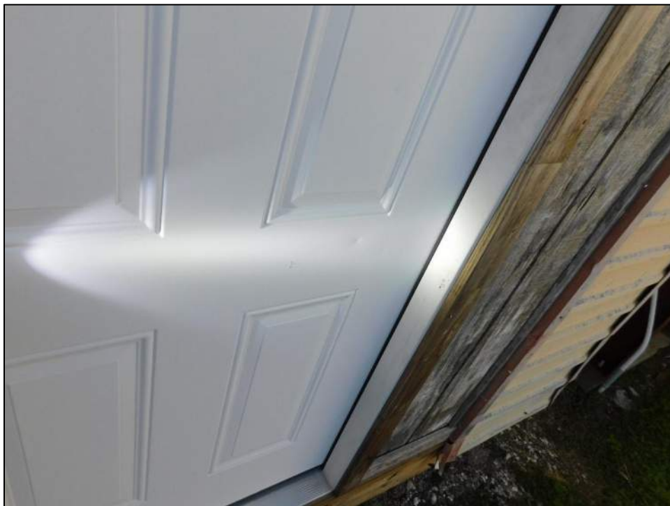
Photo 89: Isolated hail denting observed on the north-facing door of the storage building.
