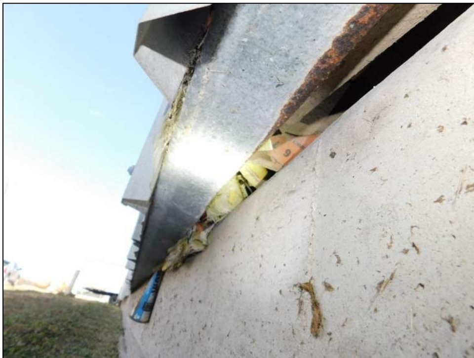
Photo 86: Upward view of the bulged-out west wall exhibited debris accumulation and edge corrosion.
