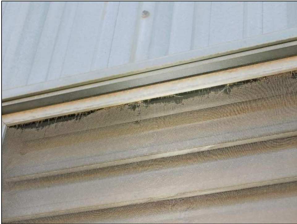
Photo 59: Dimpled screen in the north wall were mechanically torn.
