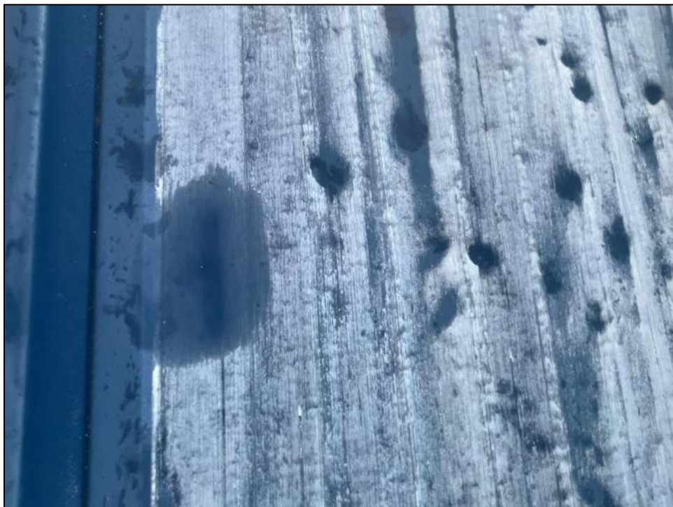
Photo 14: No coating disruptions were observed at the hail dents.
