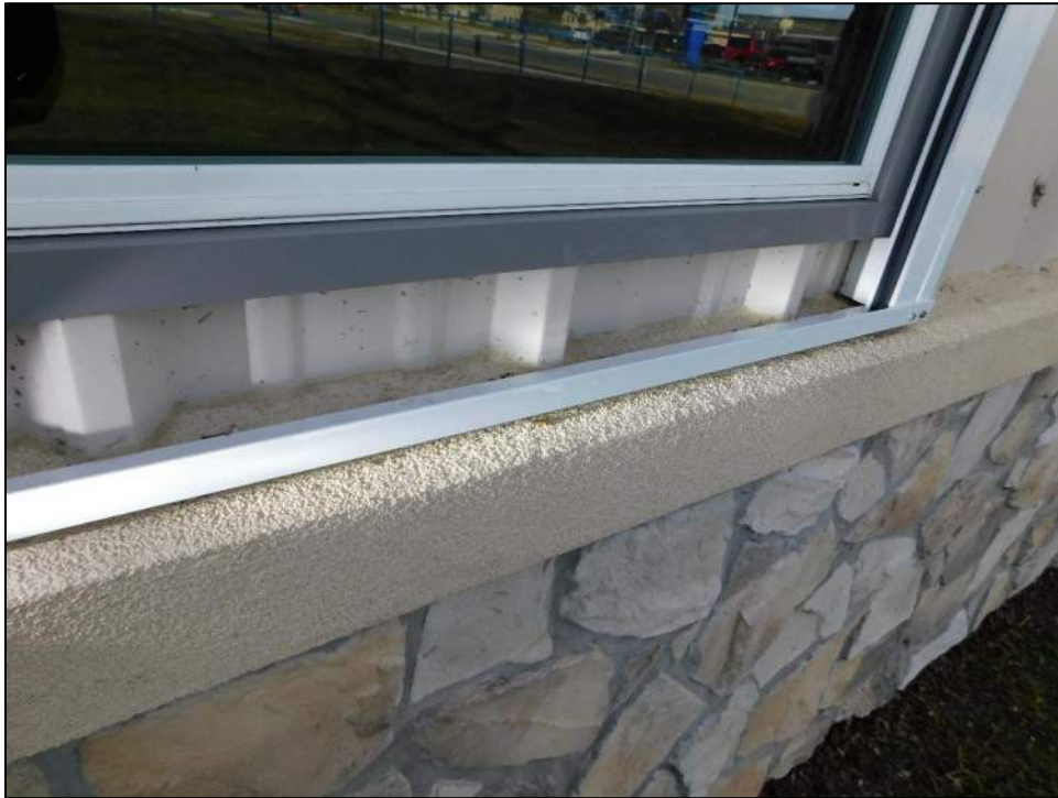
Photo 9: No hail impact fractures were observed along the EIFS accent along the west or north walls.
