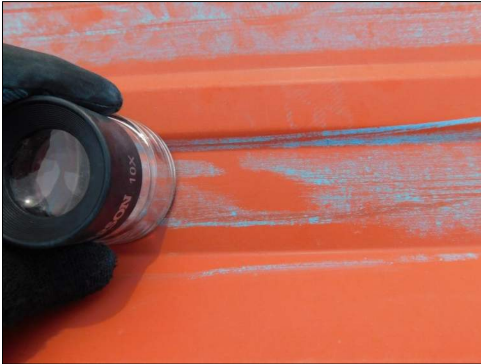
Photo 42: Denting inner diameter was less than 1/2 inch. No coating disruptions were observed.
