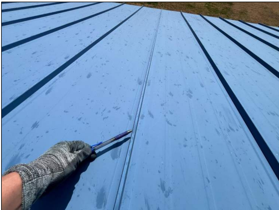
Photo 22: Standing seams remained intact.
