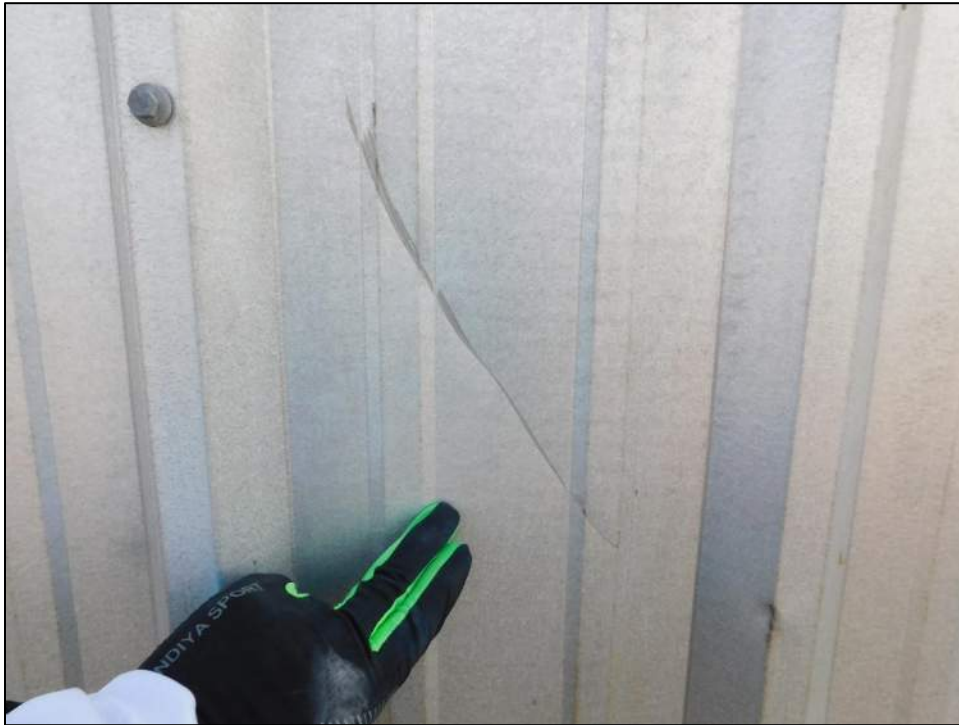
Photo 83: Mechanical damage on west wall.
