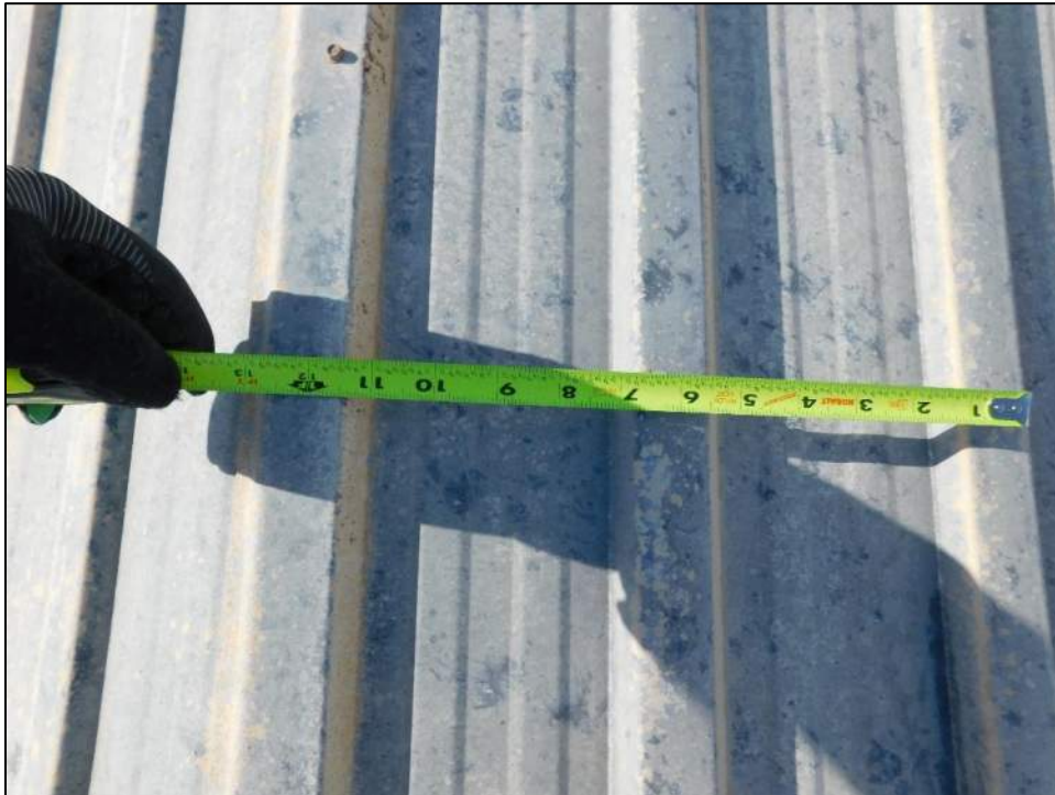
Photo 113: Spatter marks on the storage building roof reflect 1.0-inch hail.
