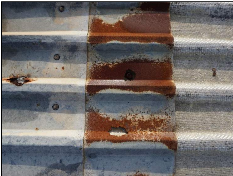
Photo 50: Corroded deck at fasteners unrelated to hail effects.
