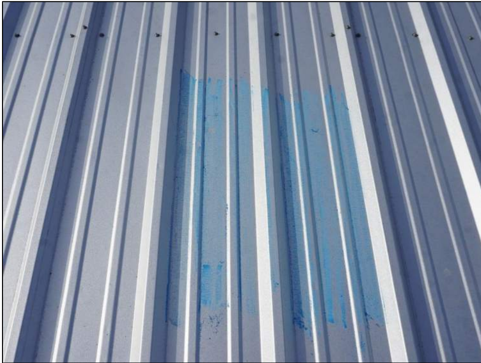
Photo 24: Hail denting on north slope had an inner diameter of less than 1/2 inch.
