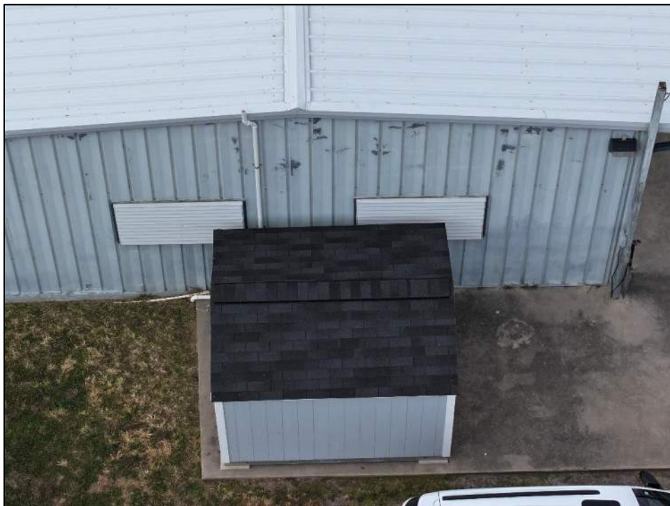
Photo 2: Tool shed on east side of the senior citizen building covered with 3-tabs asphalt shingles.
