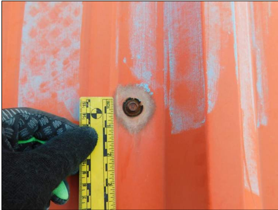
Photo 44: Typical fastener corrosion unrelated to hail impacts.
