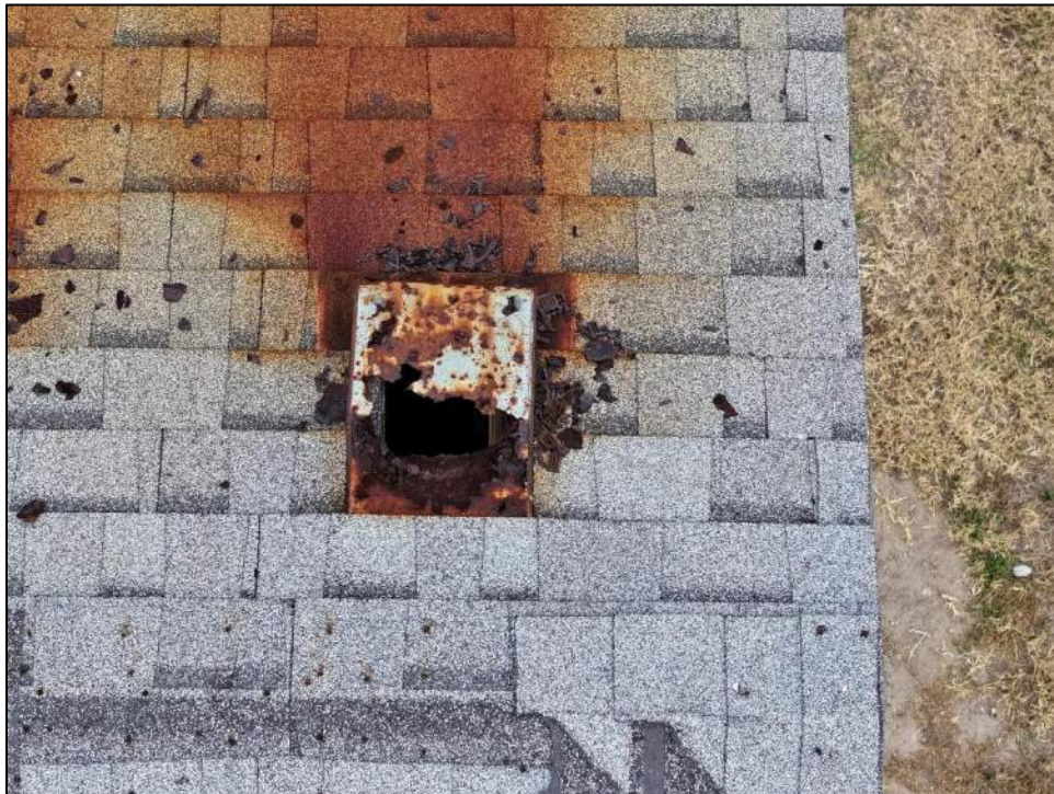
Photo 8: Deteriorated ridge vents.
