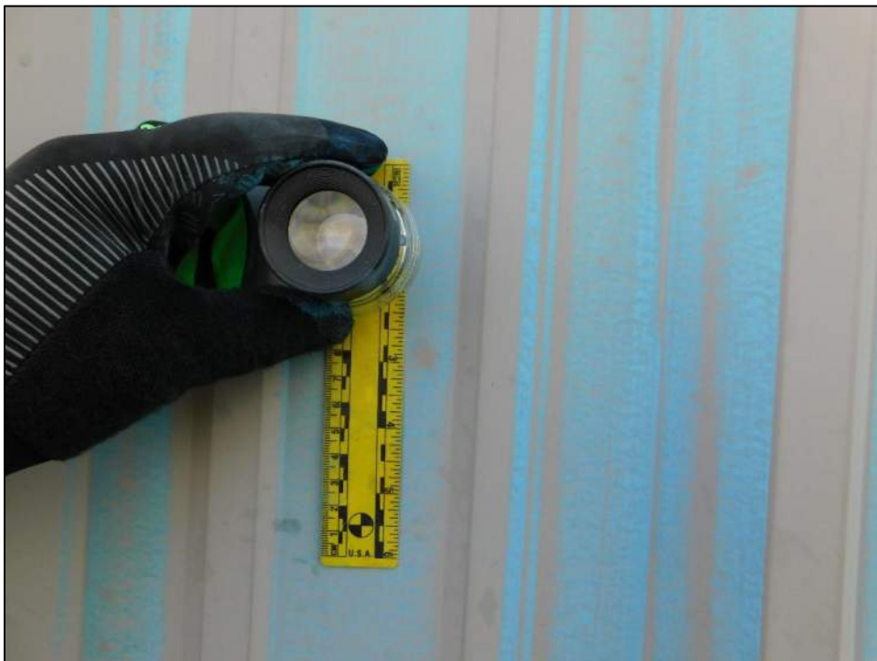
Photo 6: Hail denting on west wall were superficial with coating disruptions.
