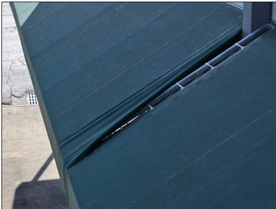
Photo 4: Pre-existing awning separation.
