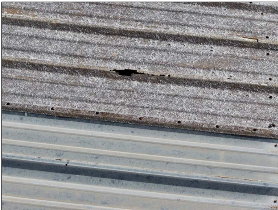
Photo 23: Skylight panels were highly deteriorated.
