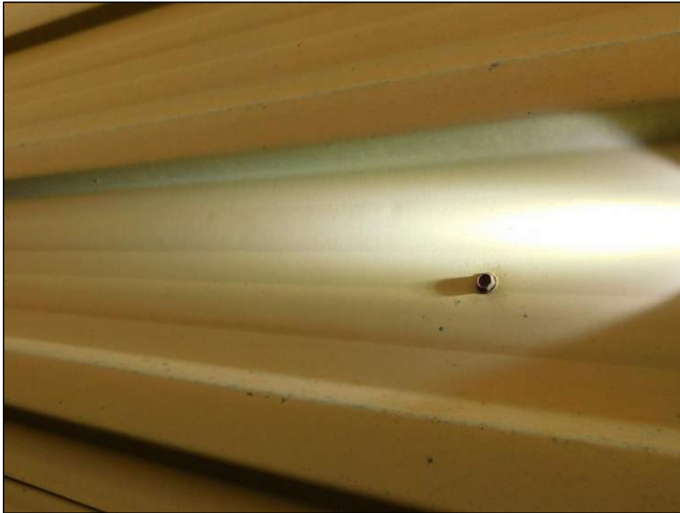
Photo 94: Slight denting observed on the west wall of the storage building.
