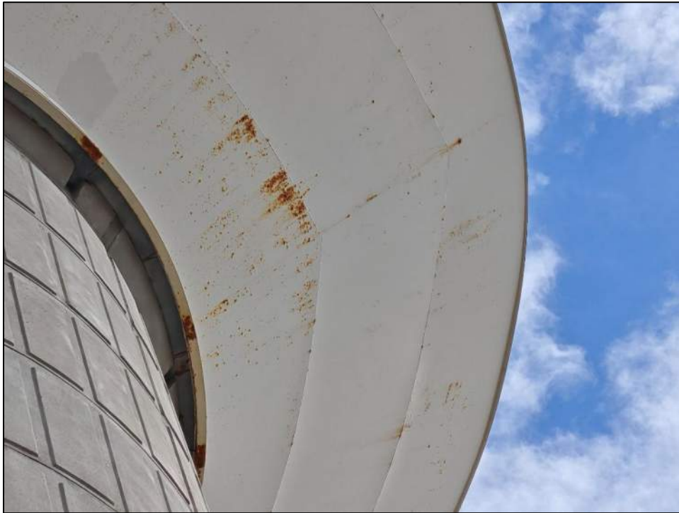
Photo 16: Underside of the tank bowl exhibited surface rusting.
