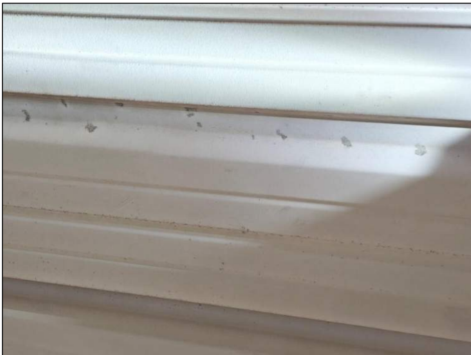
Photo 91: Denting to east slope were significantly less than west slope.
