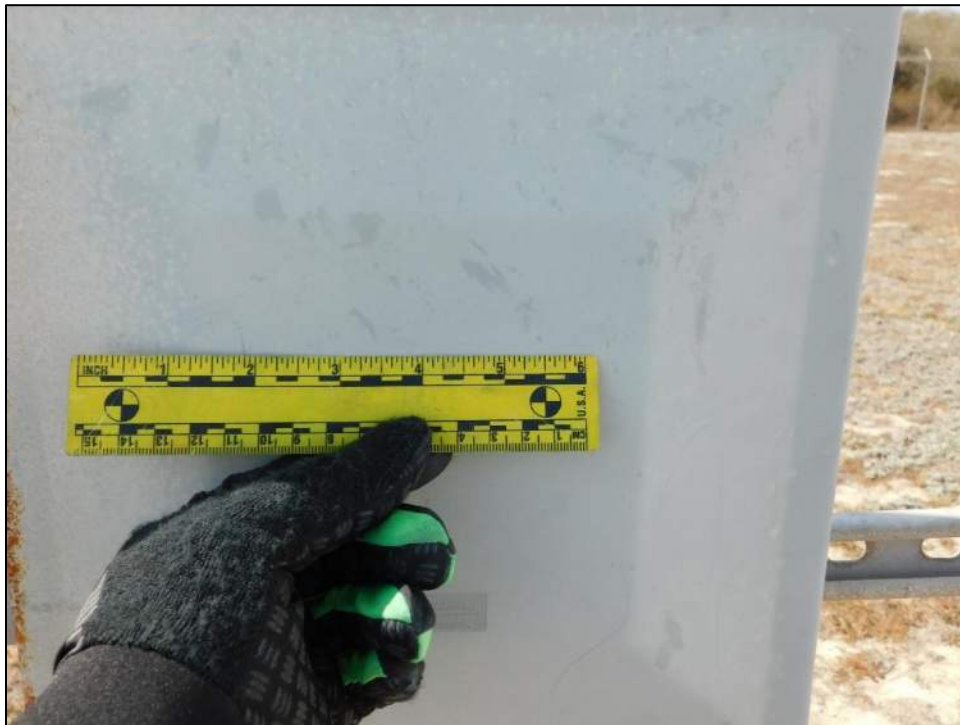
Photo 5: Hail spatter on nearby electrical panels indicative of 1-inch hail.
