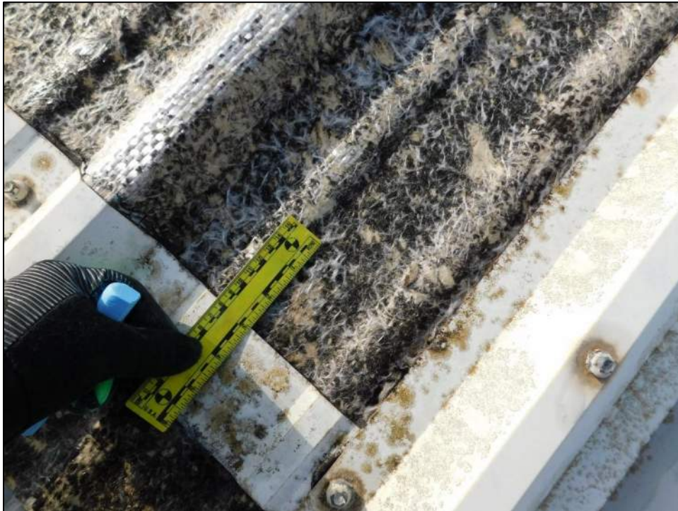
Photo 15: No discernible fractures observed at the hail spatters on the skylight panels.
