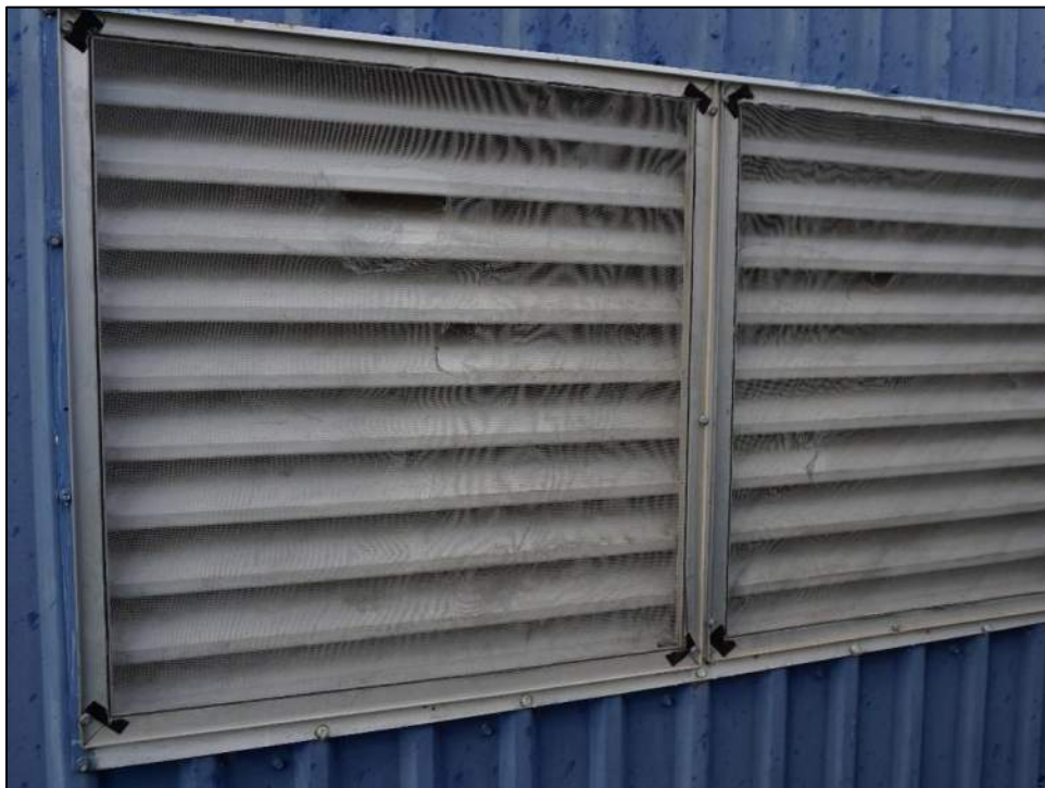
Photo 38: Torn screens on north elevation caused by mechanical damage. Hail impact caused additional dimpling damage.
