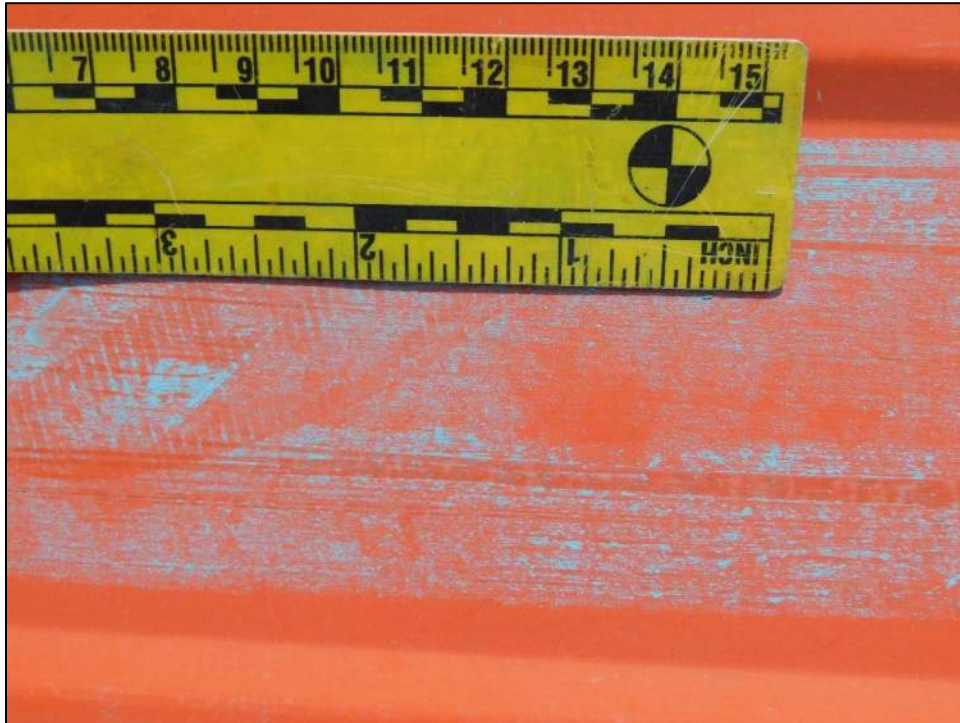
Photo 40: Denting inner diameter was less than 1/2 inch. No coating disruptions were observed.
