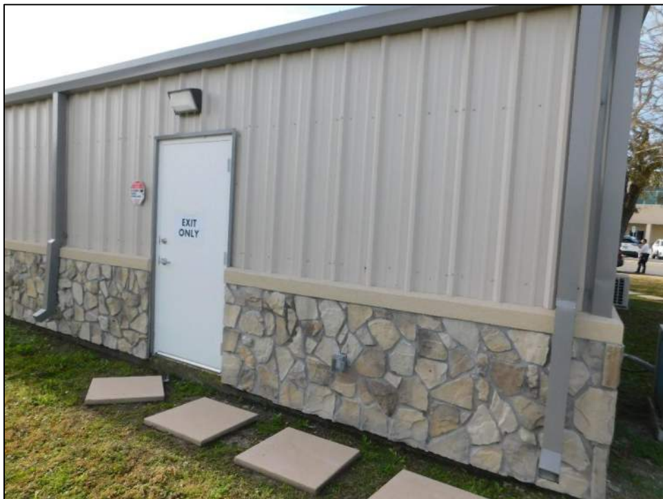
Photo 14: Gutter on the north wall exhibited slight hail impact denting.
