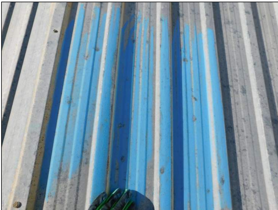
Photo 114: Hail denting on the storage building roof were less than 1/2 inch in inner diameter.
