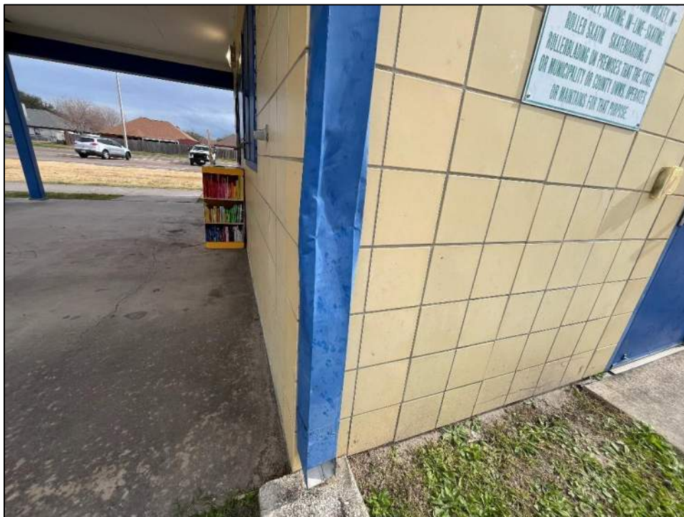
Photo 63: Mechanically deformed downspout on west wall that was inconsistent with hail impact.
