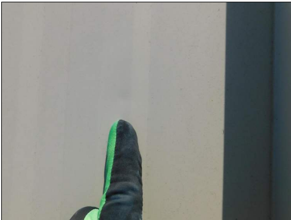
Photo 64: Close view of a hail dent on the fire department roof.
