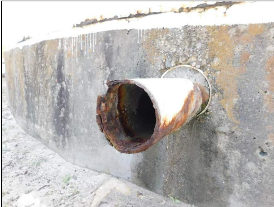
Photo 9: Close view of severely corroded drain pipe through the concrete foundation.
