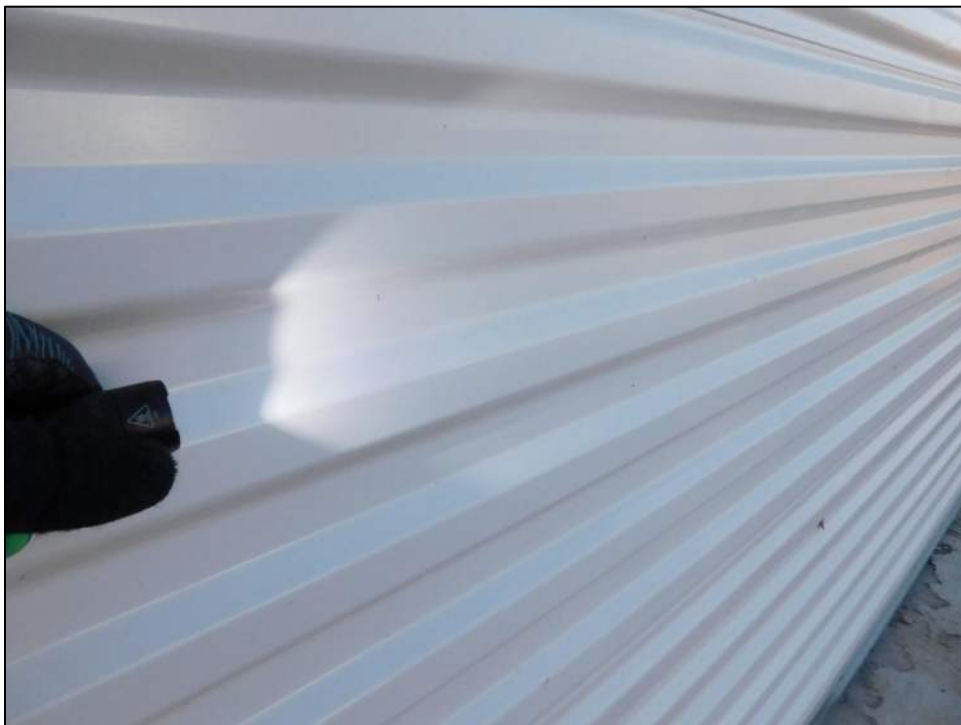
Photo 10: No hail denting on upper portion of roll-up doors.
