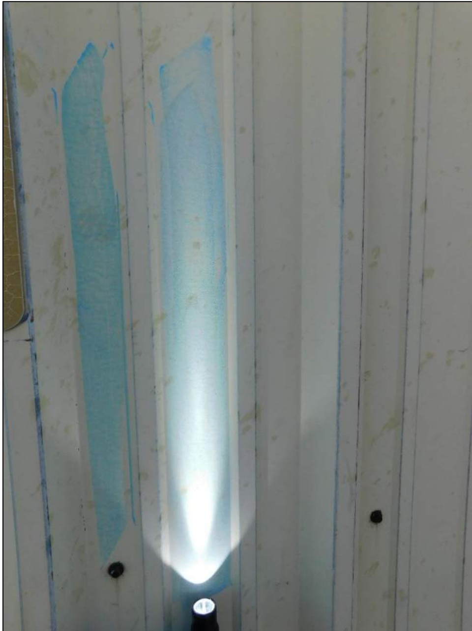
Photo 16: North wall exhibited no hail denting at the spatters.
