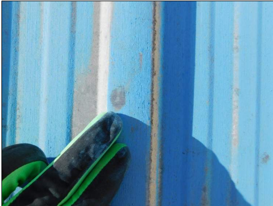
Photo 115: No coating disruptions were observed at the hail dents.
