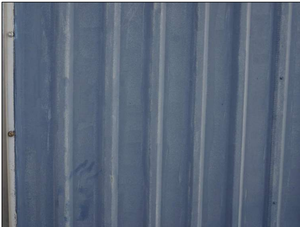
Photo 40: South wall was unaffected by the hail impact.
