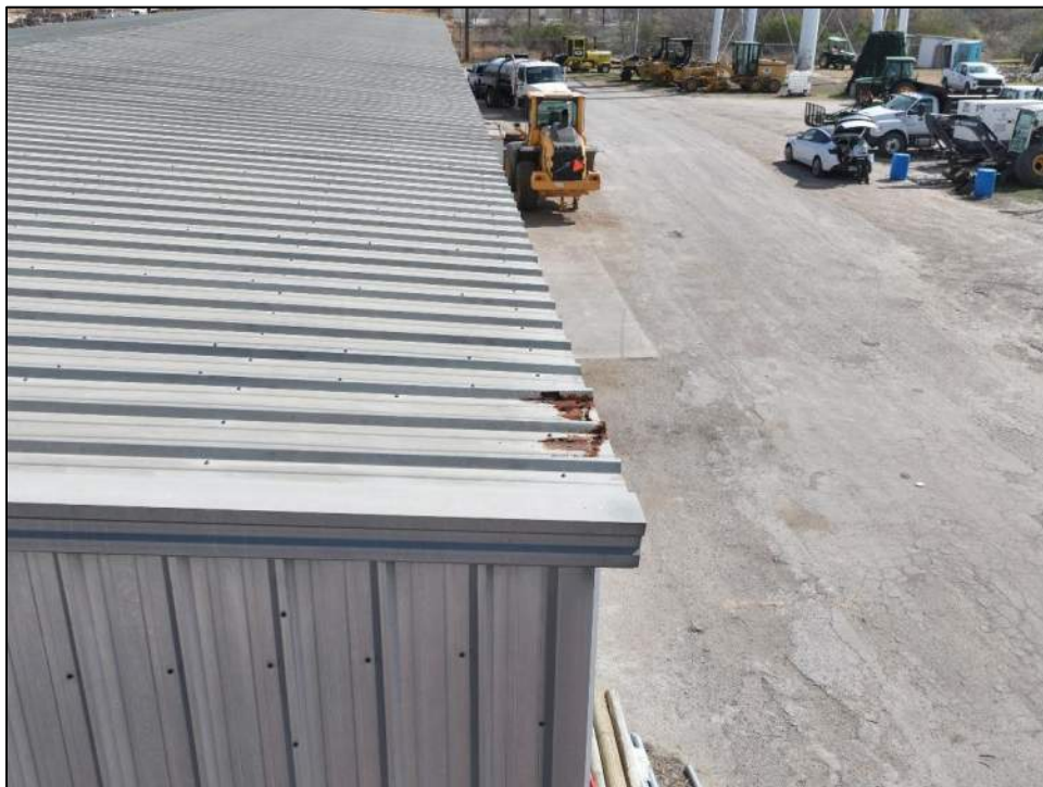
Photo 55: Intact west roof edge closure corroded southwest corner and straight-line roof eave line along the south edge.
