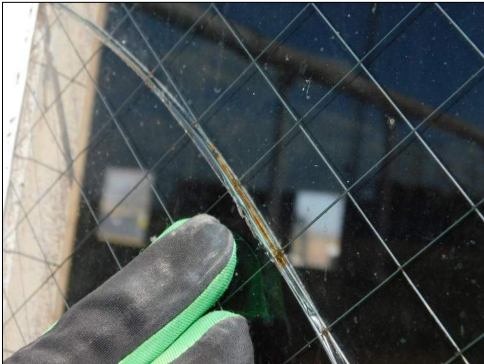
Photo 13: Close-up of the soiled and stained crack edges in the south door glazing cracks.
