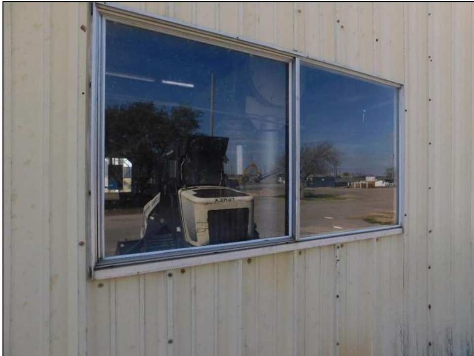
Photo 7: North wall windows remained intact.
