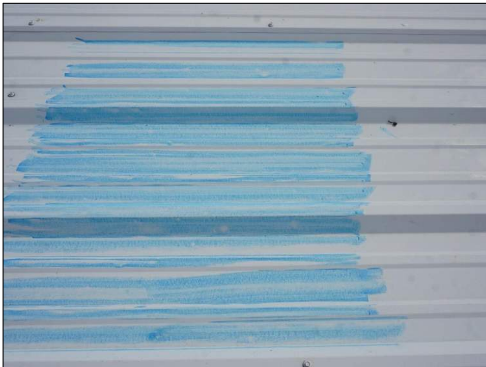
Photo 28: South slope panels exhibited indentations with largest inner diameters of less than 1/2 inch.
