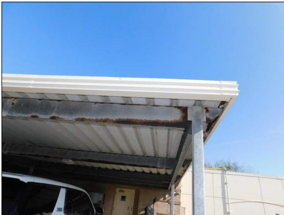
Photo 44: Corrosion was widespread on the carport structure and edge closures along the backside of the police department building.
