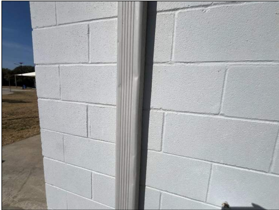
Photo 5: Mechanical denting to a downspout attached to the south wall inconsistent with hail impact.
