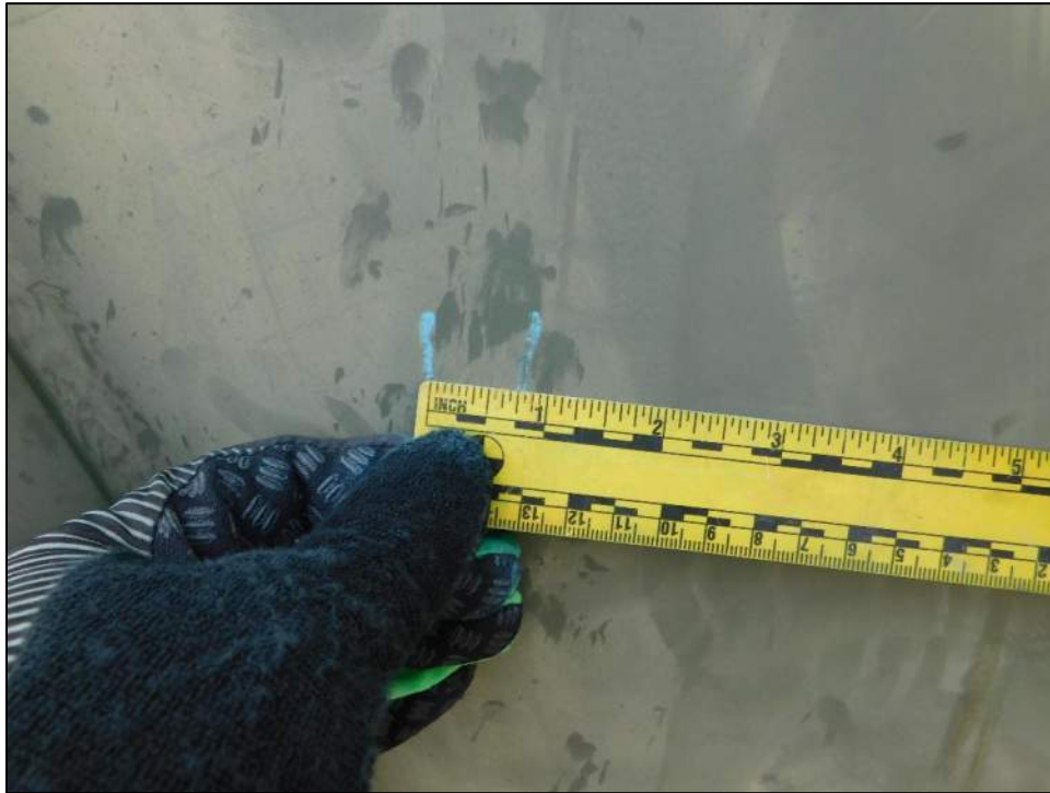
Photo 29: Hail spatters consistent with 0.75- to 1.0-inch hail on west-facing surfaces.
