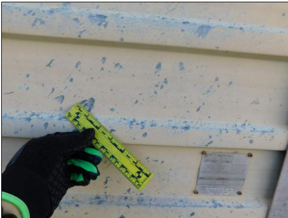
Photo 87: Hail spatters on front wall measured 1.0 inch in maximum size.
