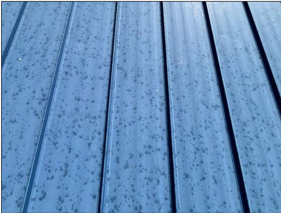
Photo 12: Hail spatters on north slope were consistent with 1.0- to 1.5-inch hail.
