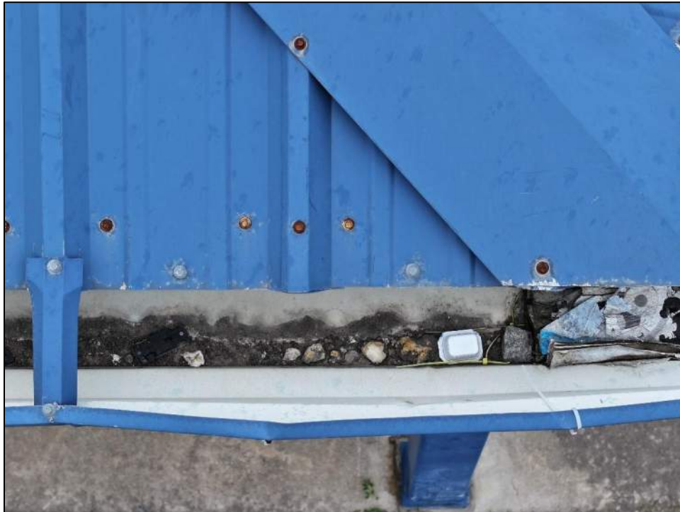
Photo 54: Debris accumulation in gutter above northeast downspout.
