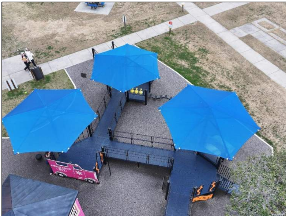
Photo 108: No punctures were observed in the smaller canopies.
