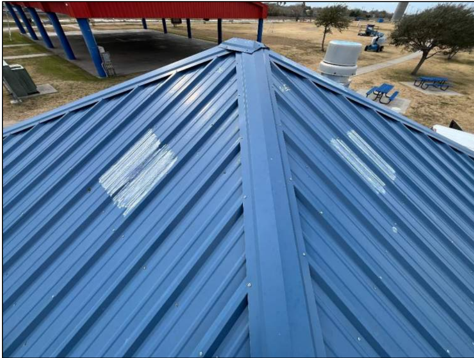
Photo 127: Ridge and hip caps remained fastened.
