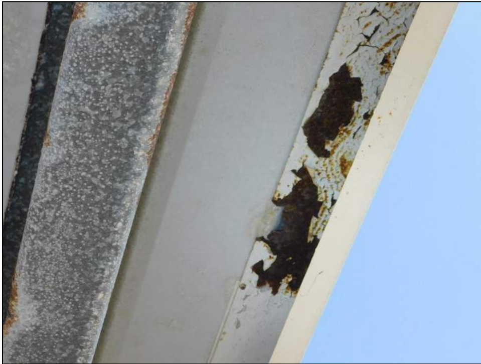
Photo 45: Corrosion was widespread on the carport structure and edge closures along the backside of the police department building.
