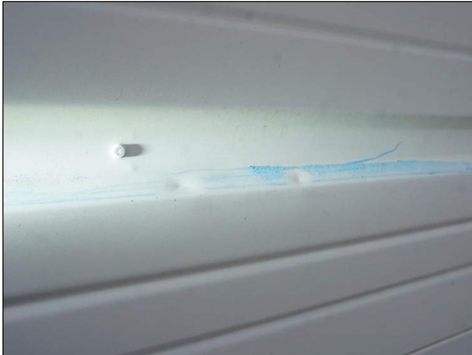
Photo 41: Denting along the top surfaces of the roll-up door along the north elevation consistent with hail impact.
