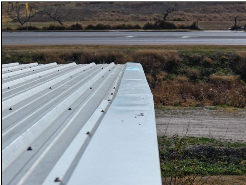
Photo 4: Hail denting visible on closure trim.
