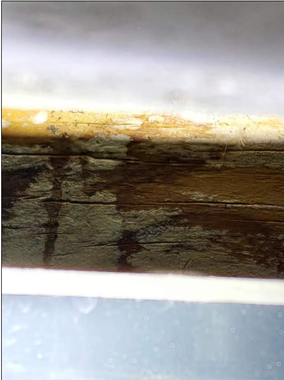
Photo 42: Additional view of the darkly stained plywood wall sheathing above the stained ceiling tile.
