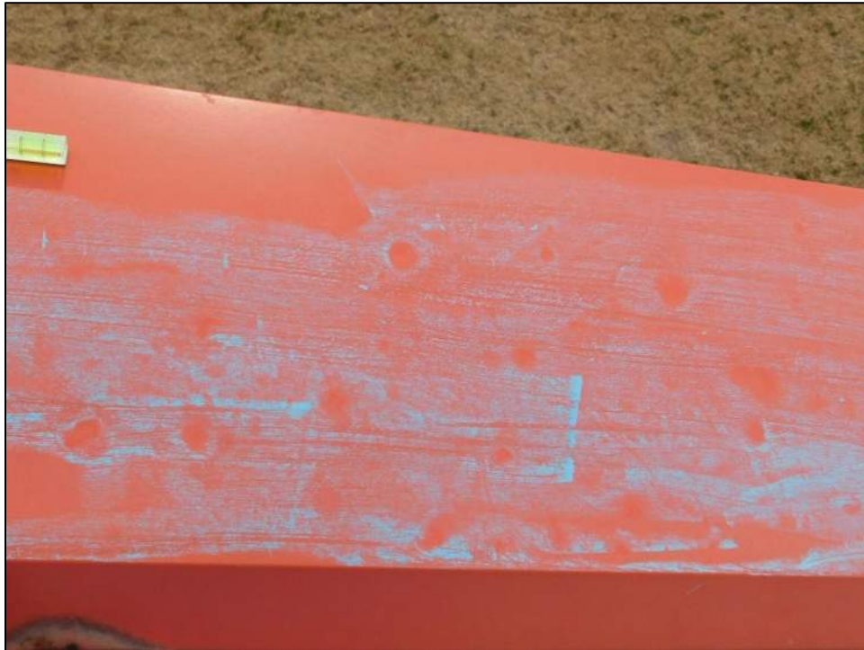
Photo 50: Indentations on gable end rake closures were dented absent of coating disruptions.
