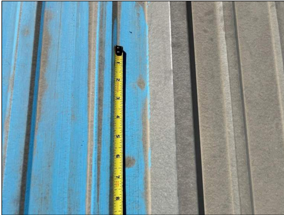
Photo 69: Denting in roof panels had inner diameter of less than 3/8 inch.
