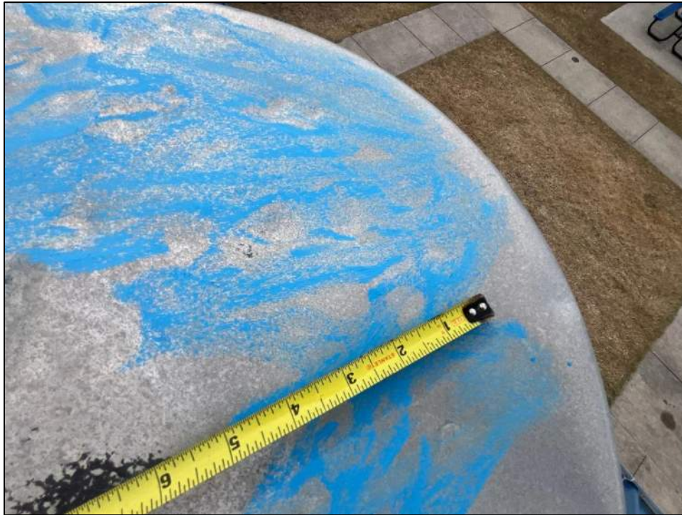
Photo 132: Hail dents on the top of the aluminum vent hood.
