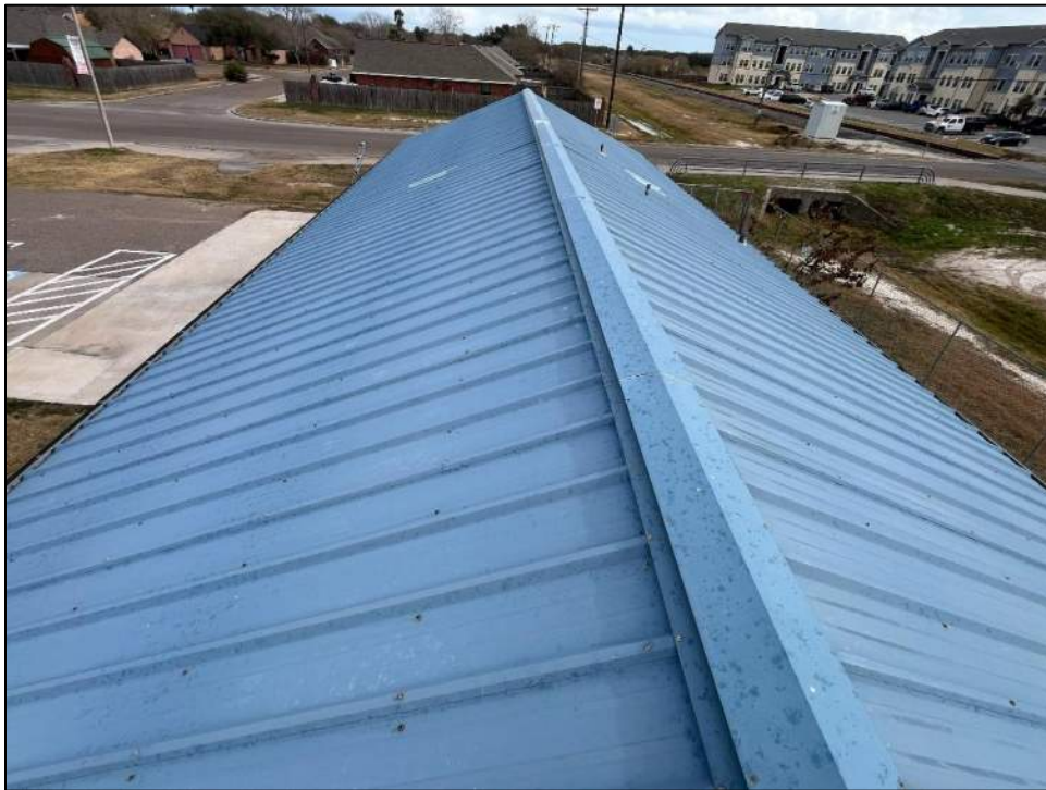
Photo 16: Ridge vent remained tightly fastened to roof panels.
