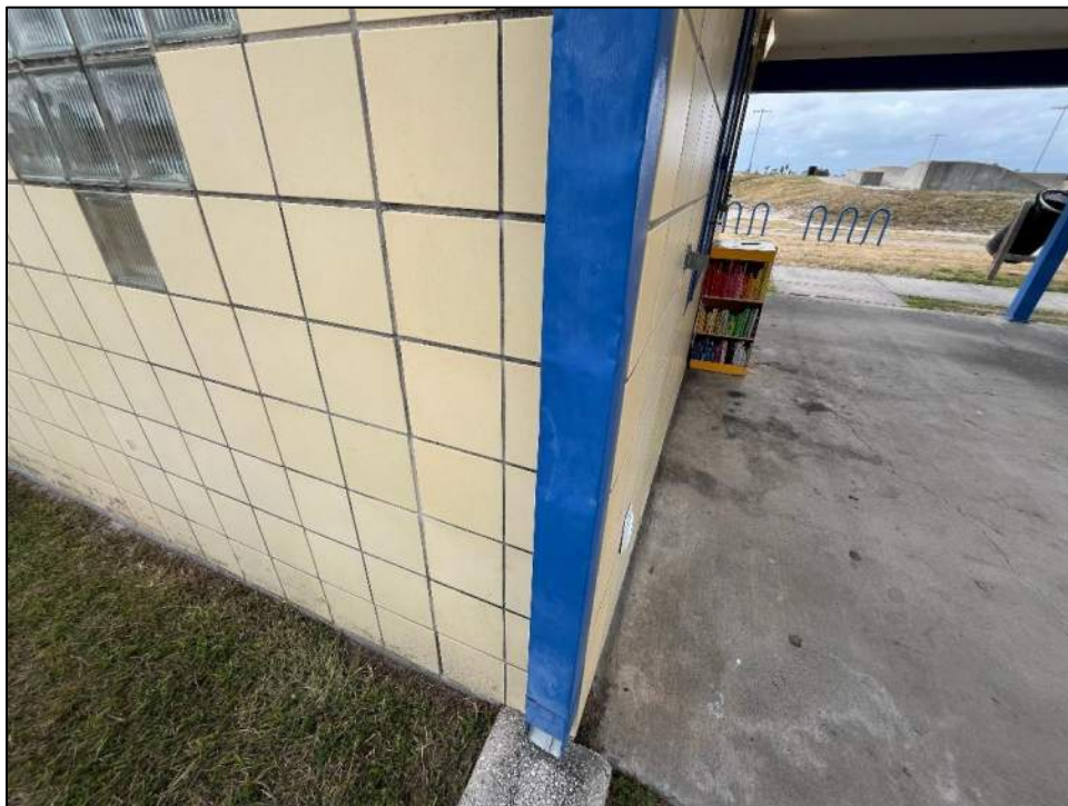
Photo 59: Mechanically deformed downspout on east wall where no hail impacts were observed.
