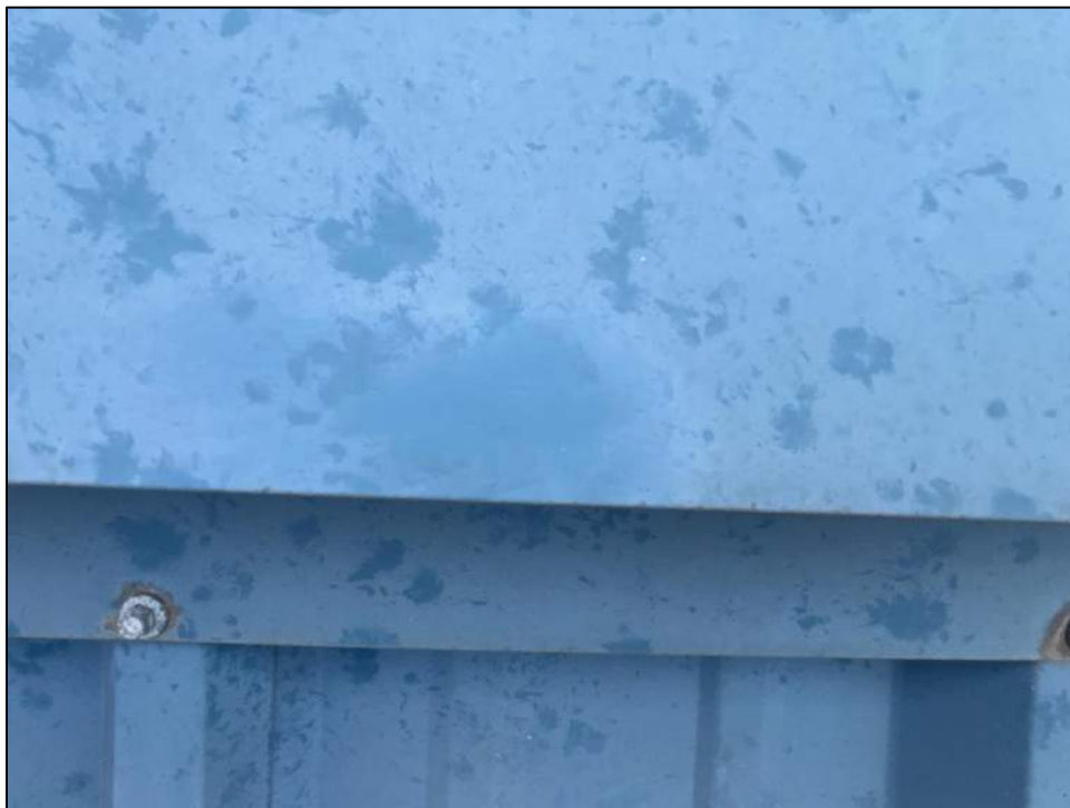
Photo 21: No coating disruptions were observed at the hail spatters along the ridge cap.
