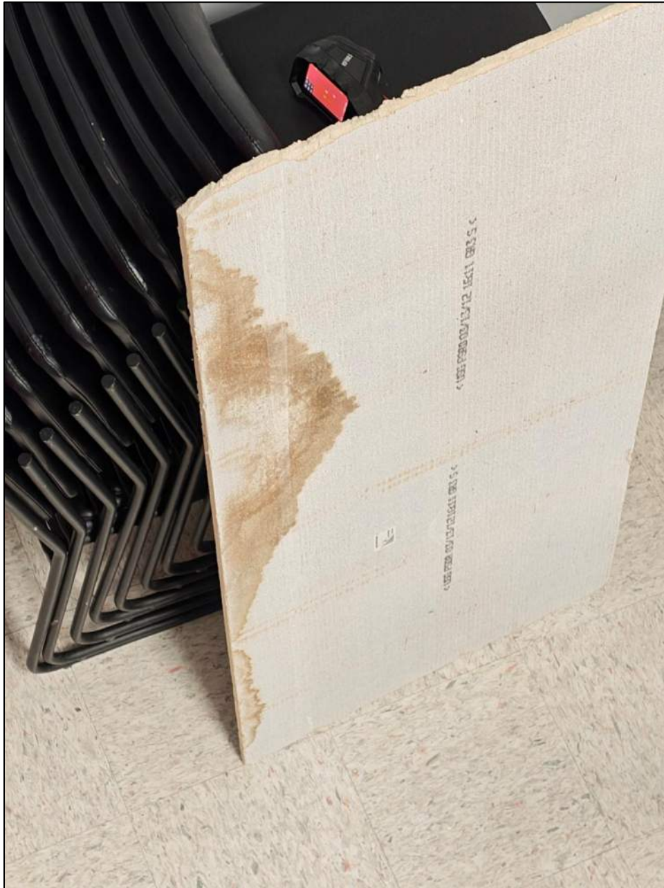
Photo 40: The stained ceiling tile was made in 2012 and exhibited multiple concentric rings of stains.
