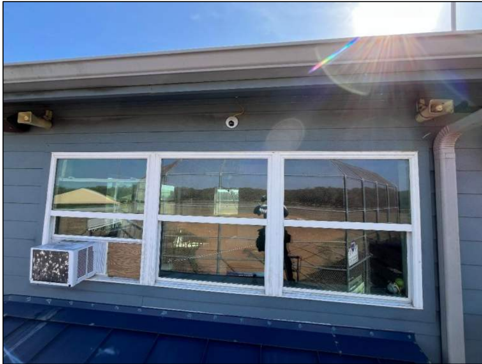
Photo 21: North wall windows remained intact Windows AC exhibited denting to condenser coils.
