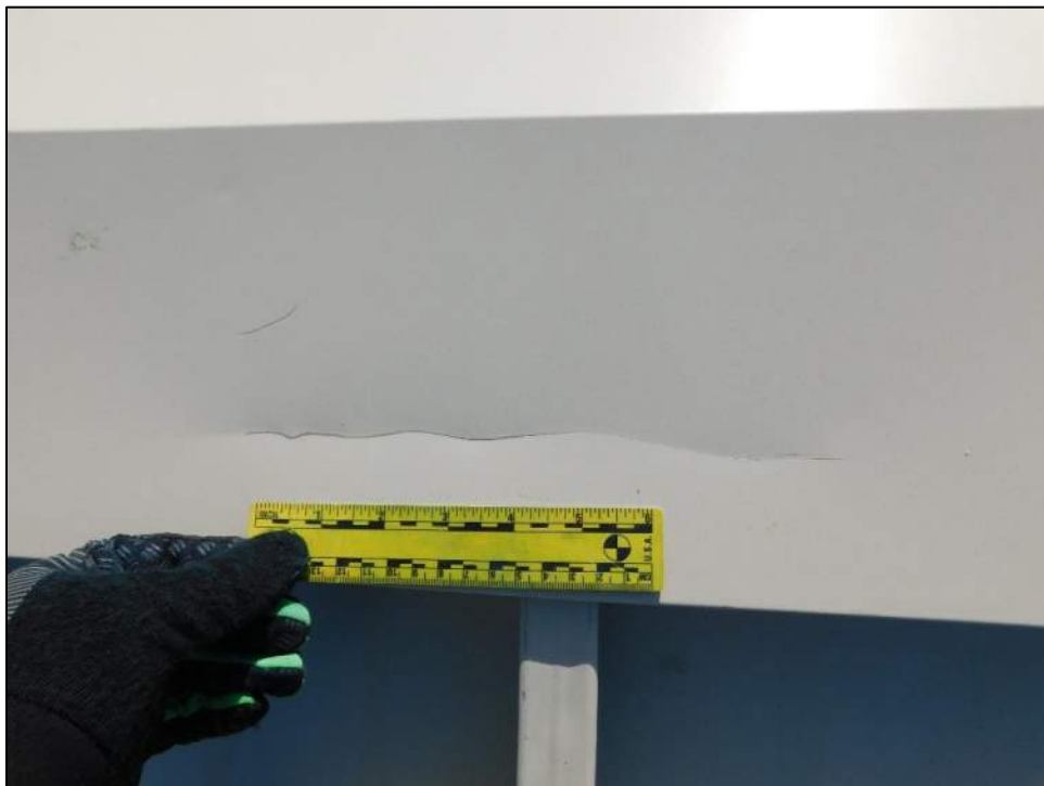
Photo 66: Typical mechanical scuff along the roof ridge that was irrelevant to hail impact.
