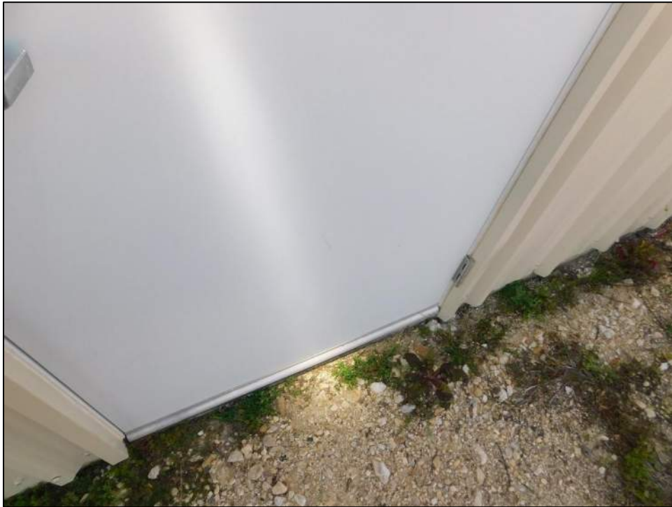
Photo 9: No hail denting on west-facing doors.
