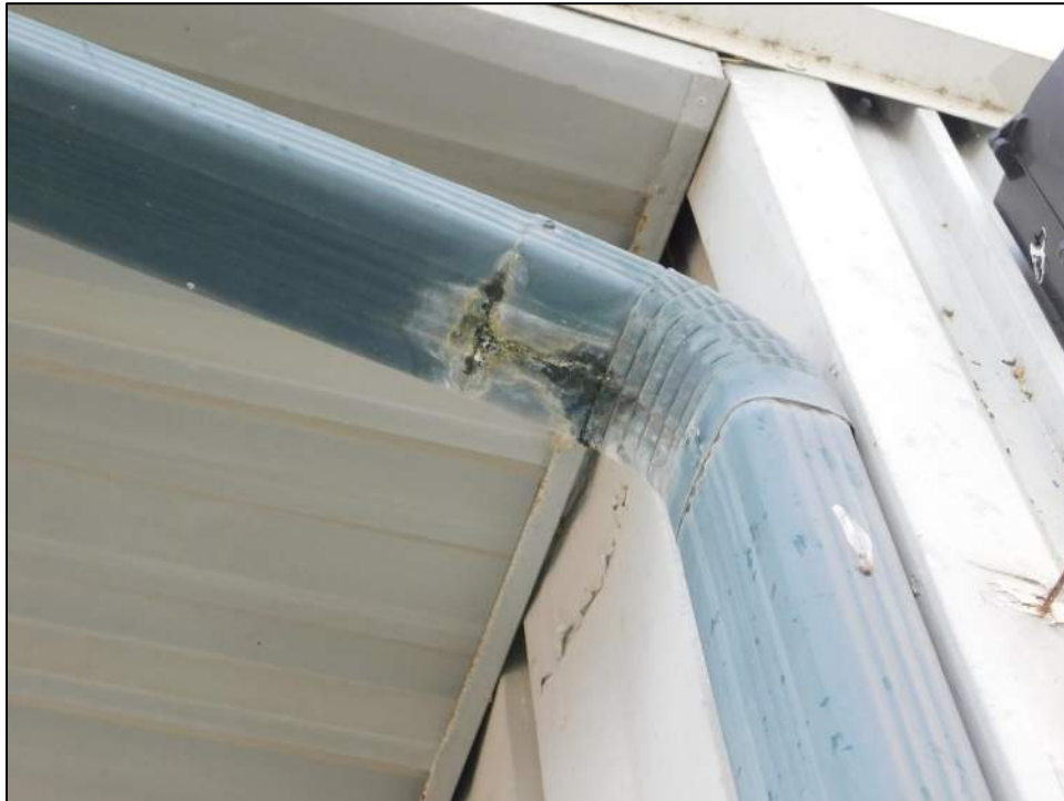
Photo 17: downspout corrosion irrelevant to hail impact.
