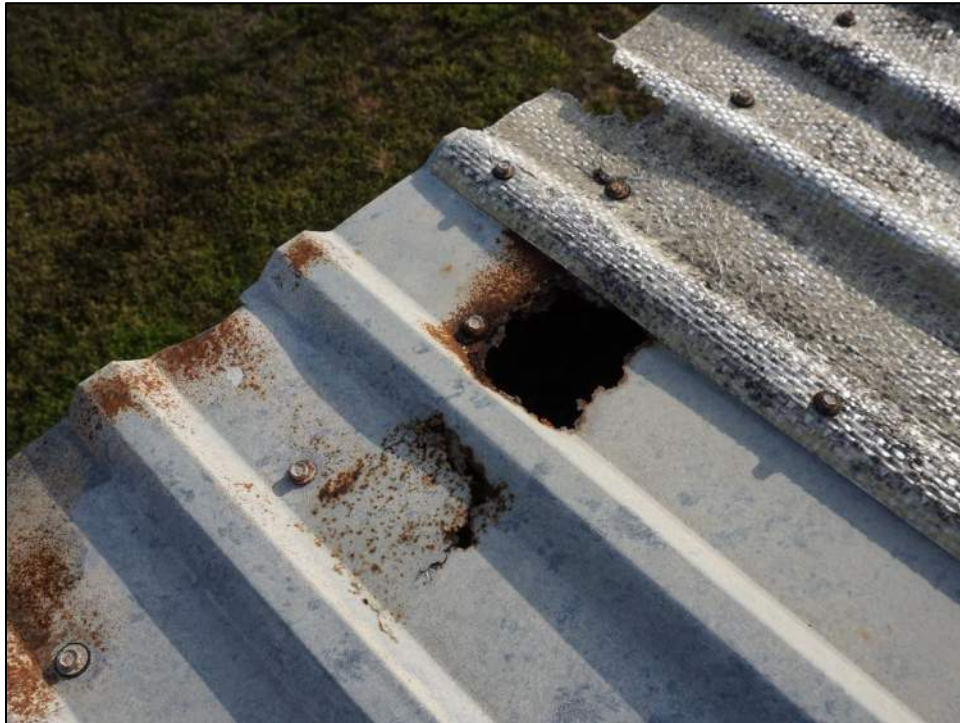
Photo 57: Rusting-through of deck at eave area near fasteners.
