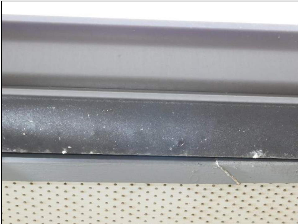
Photo 7: Closer view of the hail dents at the bottom of the front aluminum gutter.
