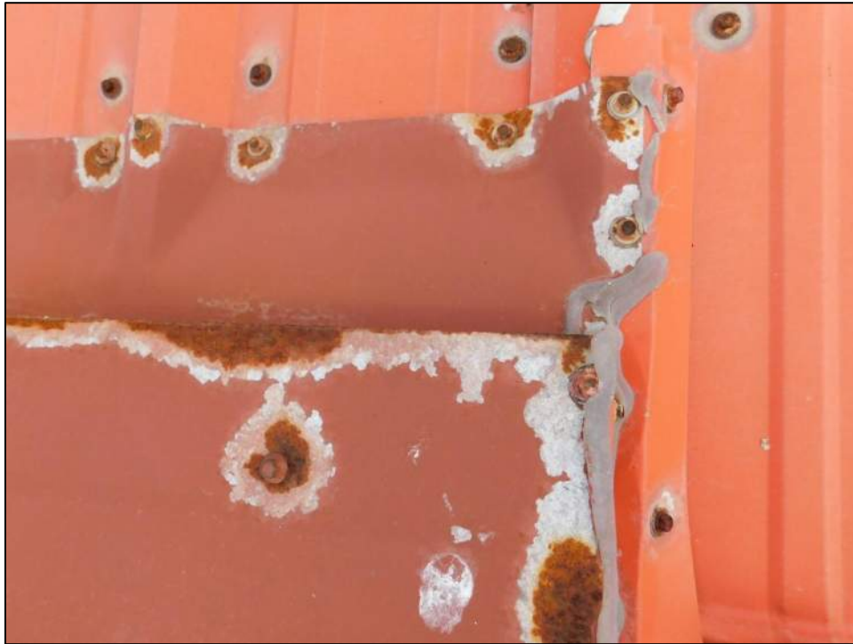
Photo 36: Widespread steel corrosion along other ridge vents.
