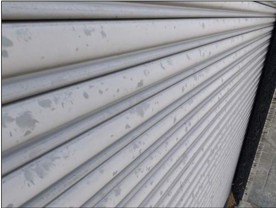
Photo 18: Hail spatters on the roll-up door were unaccompanied by indentations.
