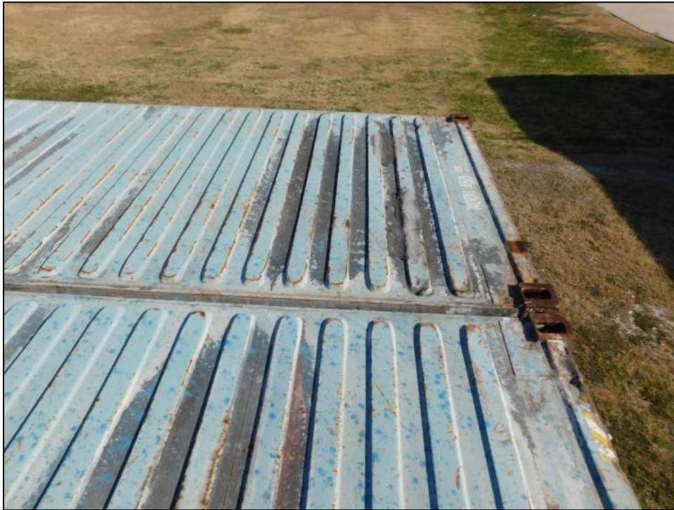
Photo 109: Container storage located along the north side of the vehicle storage building exhibited hail spatters widespread rusting.
