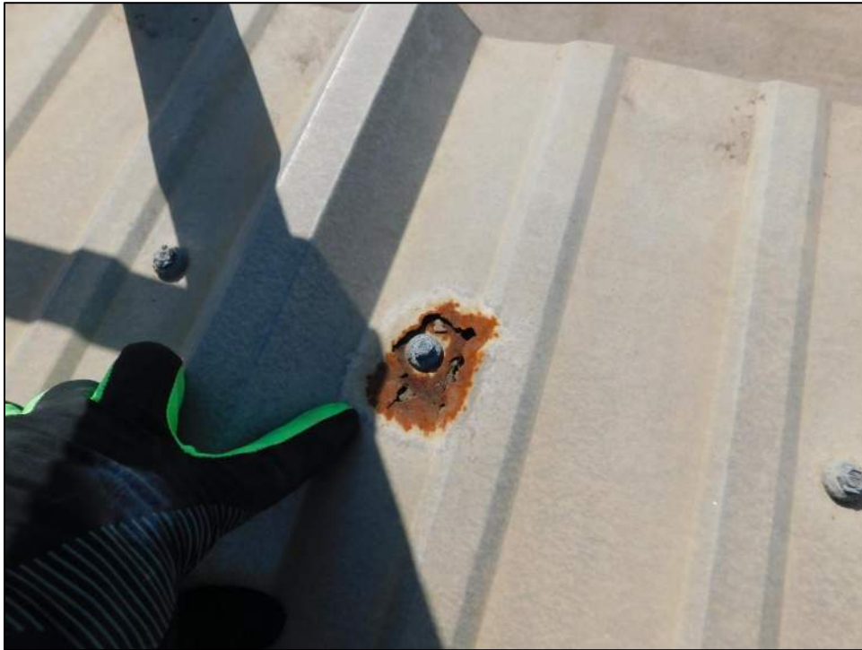
Photo 67: Corroded roof deck at fastener locations.
