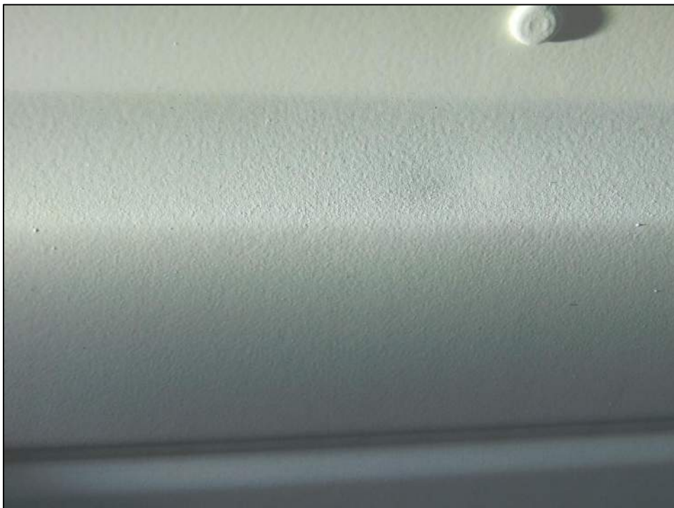
Photo 38: Close-up of the slight denting on the roll-up door consistent with hail impact. No coating disruptions were observed.
