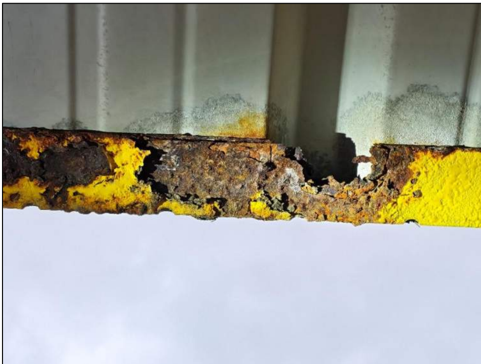
Photo 94: Typical closure metal corrosion along roof eaves.
