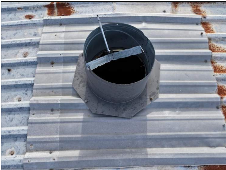
Photo 44: The missing ridge vent cover on the east side of the ridge was an existing condition since 2017.
