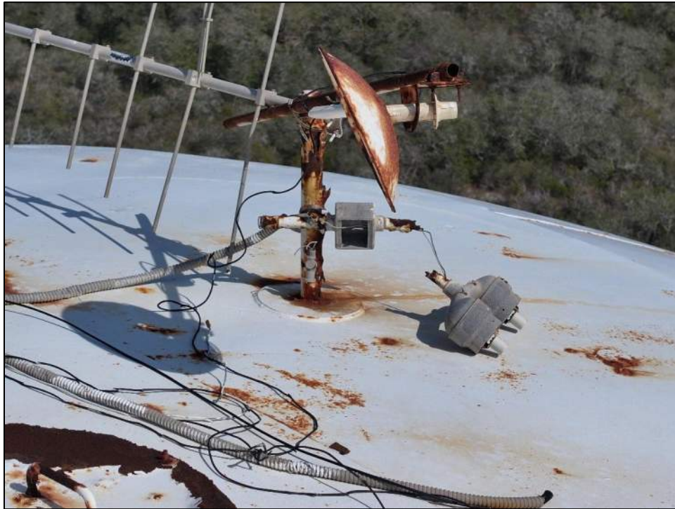
Photo 19: Corrosion of roof-mount tubing resulted in detached fixtures unrelated to hail impact.
