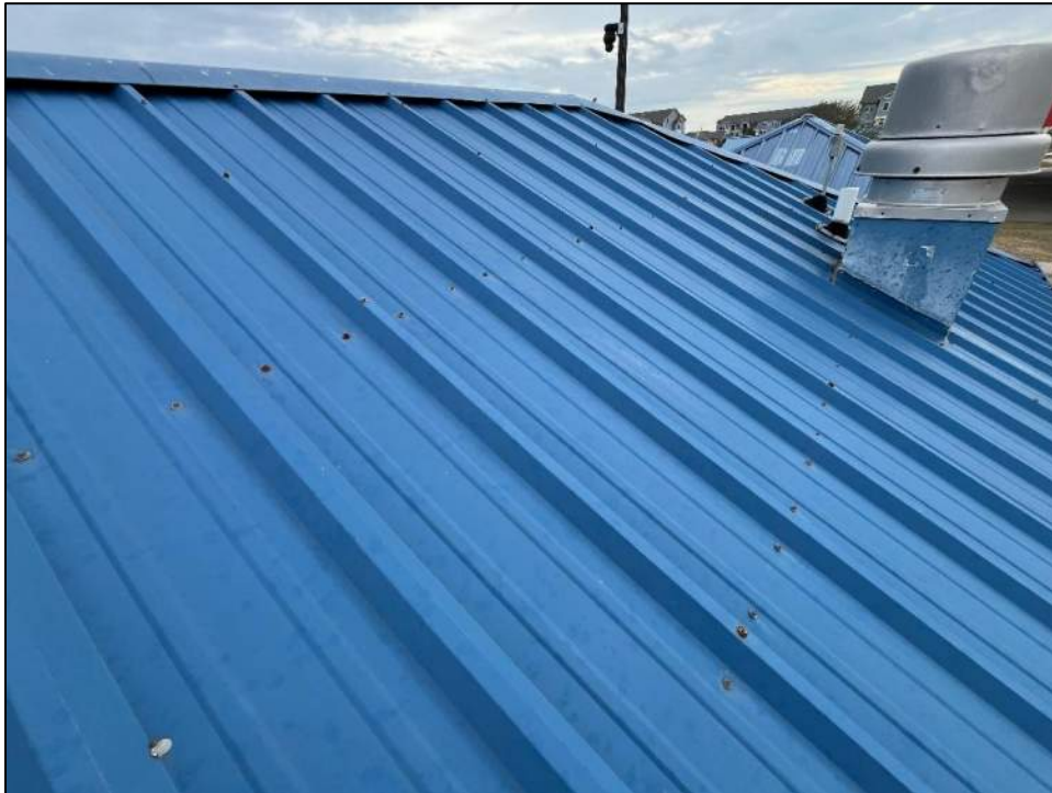
Photo 68: West slope. Note widespread fastener corrosion.
