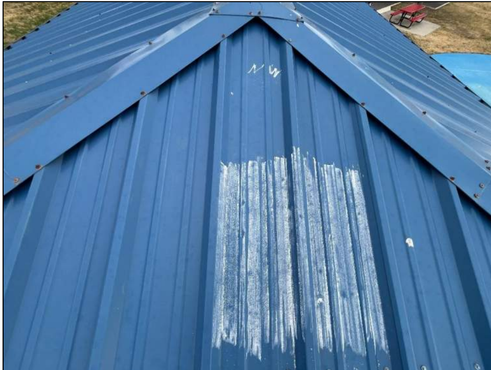
Photo 13: Hail spatters and denting observed on west slope indicative of 1-inch hail.
