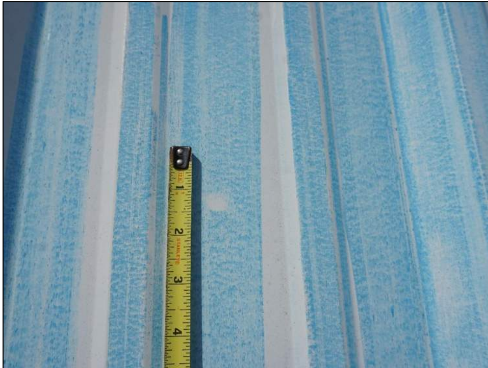
Photo 25: North slope hail dents had inner diameter less than 1/2 inch.
