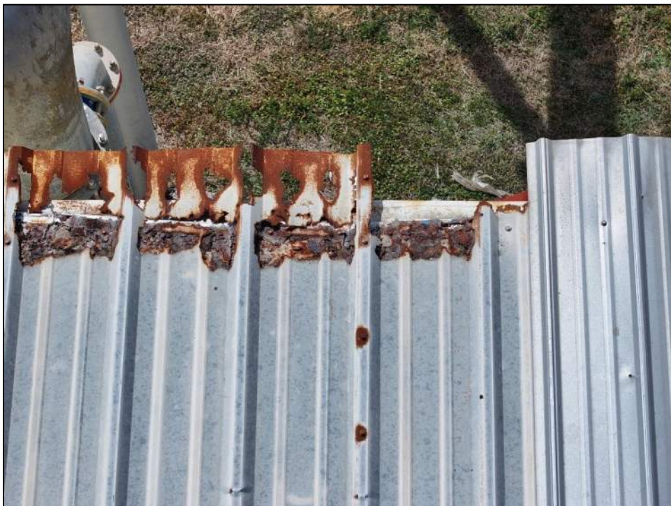
Photo 21: Severe south roof eave corrosion over south wall.
