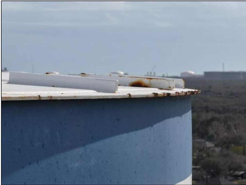
Photo 11: Tank roof plate was approximately 1/4-inch thick. Note edge corrosion.
