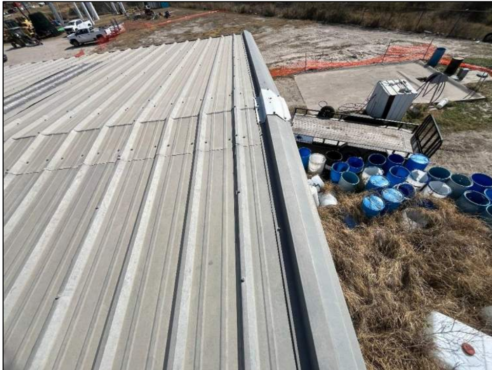
Photo 98: Closure metal along the south edge of the vehicle storage building remained attached and linear.
