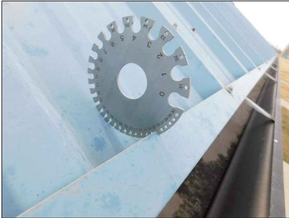
Photo 11: Splash guard metal was 25 gauge
