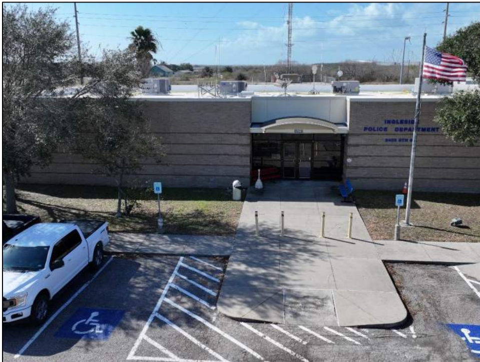
Photo 32: Front elevation of the police station building. The polycarbonate canopy above the front entry sustained hail impact fractures.
