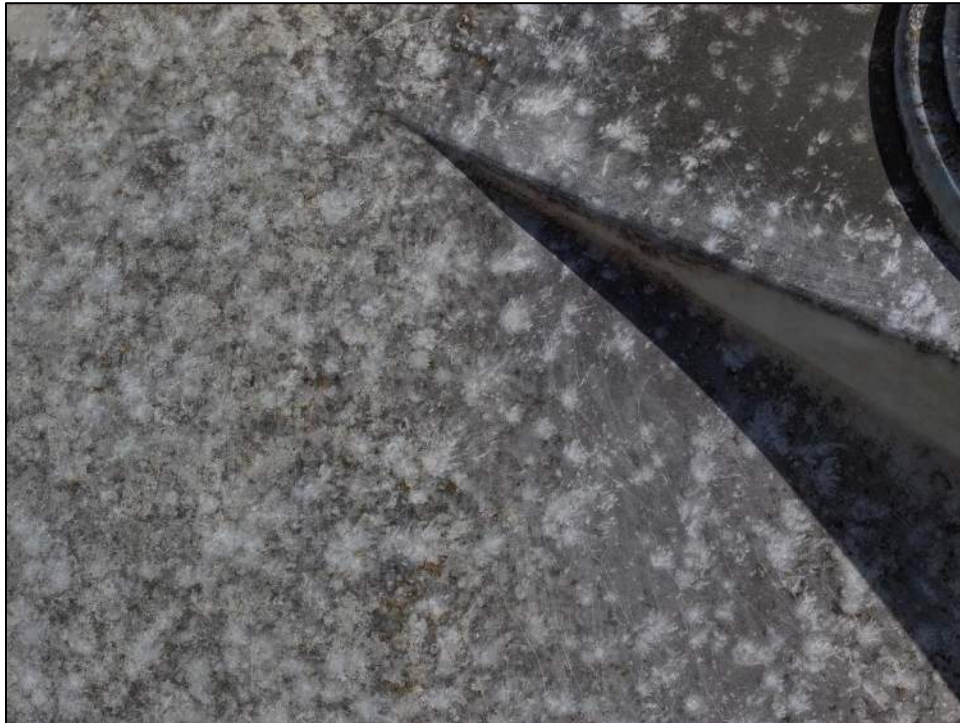
Photo 7: Hail spatter on nearby electrical panels indicative of 1-inch hail.
