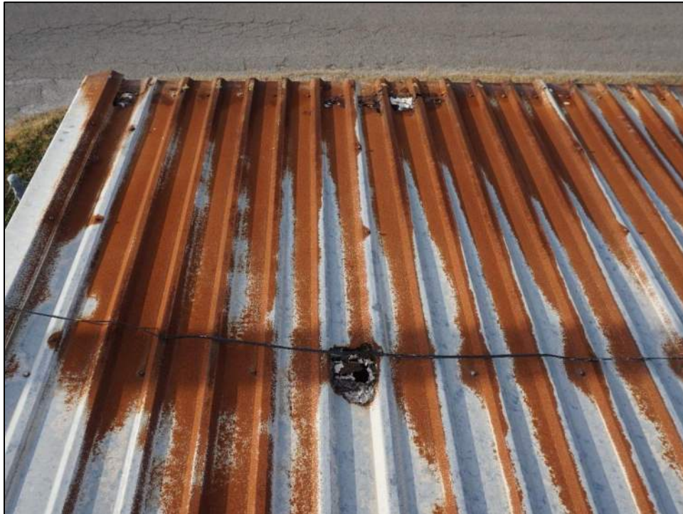
Photo 51: Rusty-through deck at south-east quadrant a long-term condition unrelated to recent hail.
