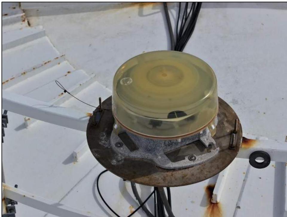
Photo 14: The polycarbonate casing of the aviation obstruction light were not fractured.
