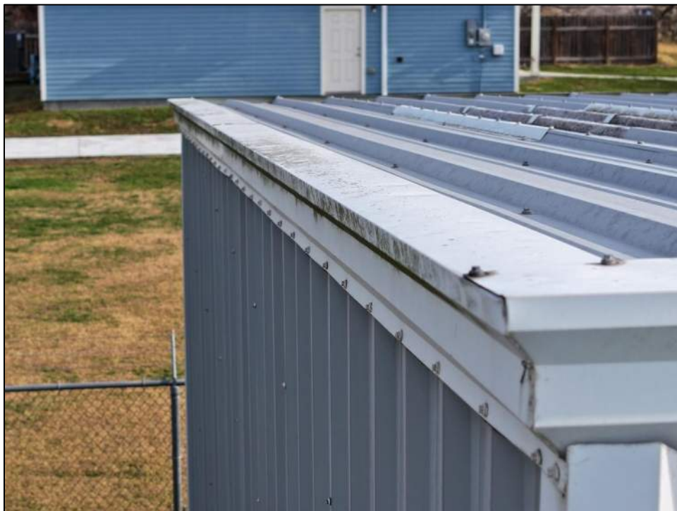
Photo 10: West rake closure remained securely fastened. Note surface denting at the top consistent with hail impact.
