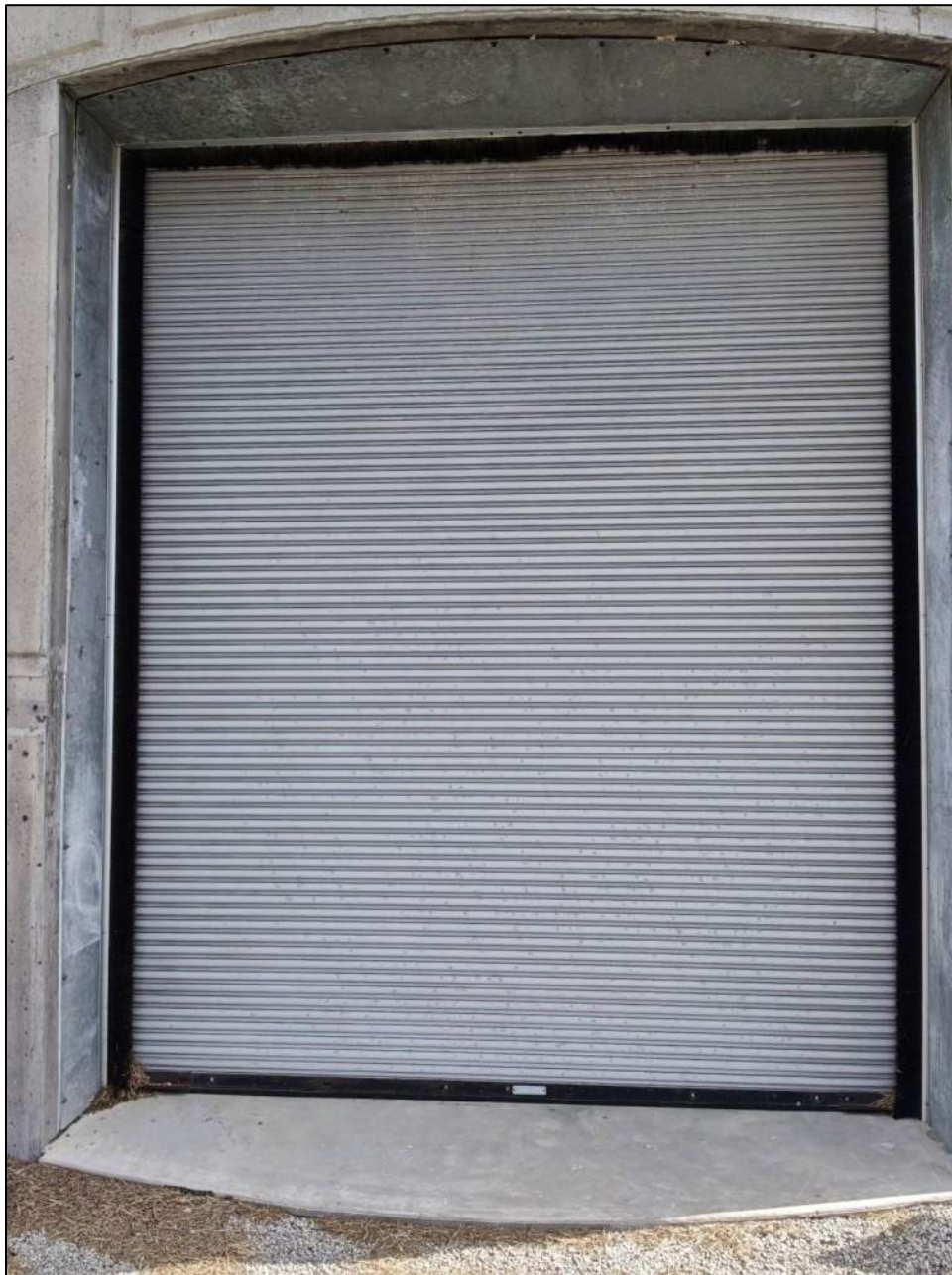
Photo 17: West-facing roll-up door were not dented.
