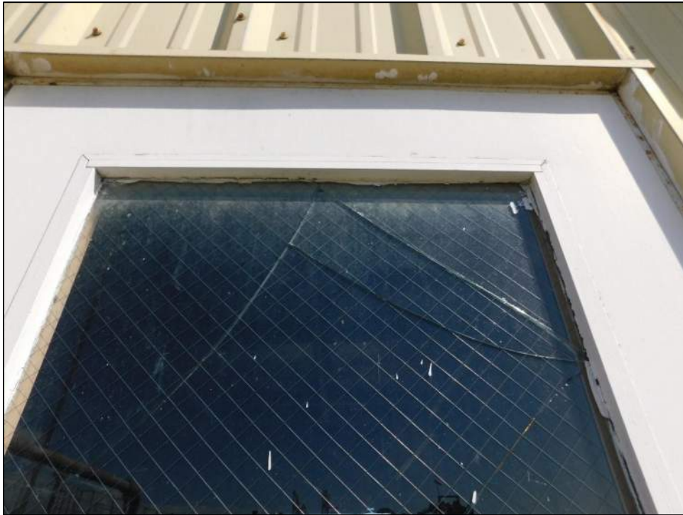
Photo 12: Cracked door glazing in the south (rear) wall unaffected by hail impact.
