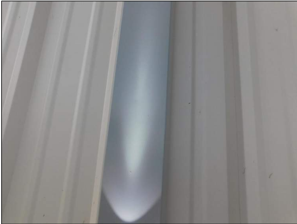
Photo 16: Slight isolated denting on the rear gutter downspout.
