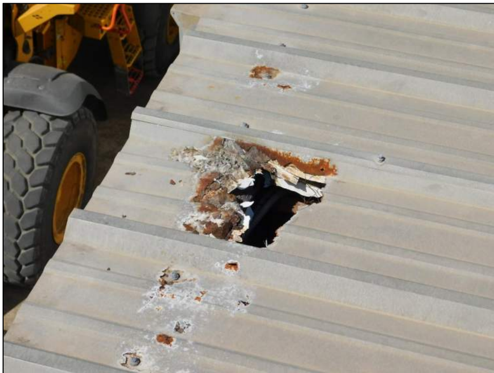
Photo 66: Corroded roof eave along front side of roof inconsistent with hail impact.
