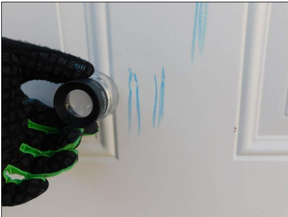
Photo 91: Closer view indicated no coating disruption to the dented door surface.
