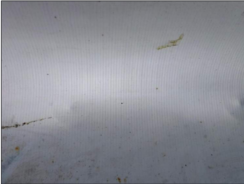
Photo 33: Unsupported PVC membranes at the base of parapets facing the direction of the hail were not punctured dimpled or scuffed.
