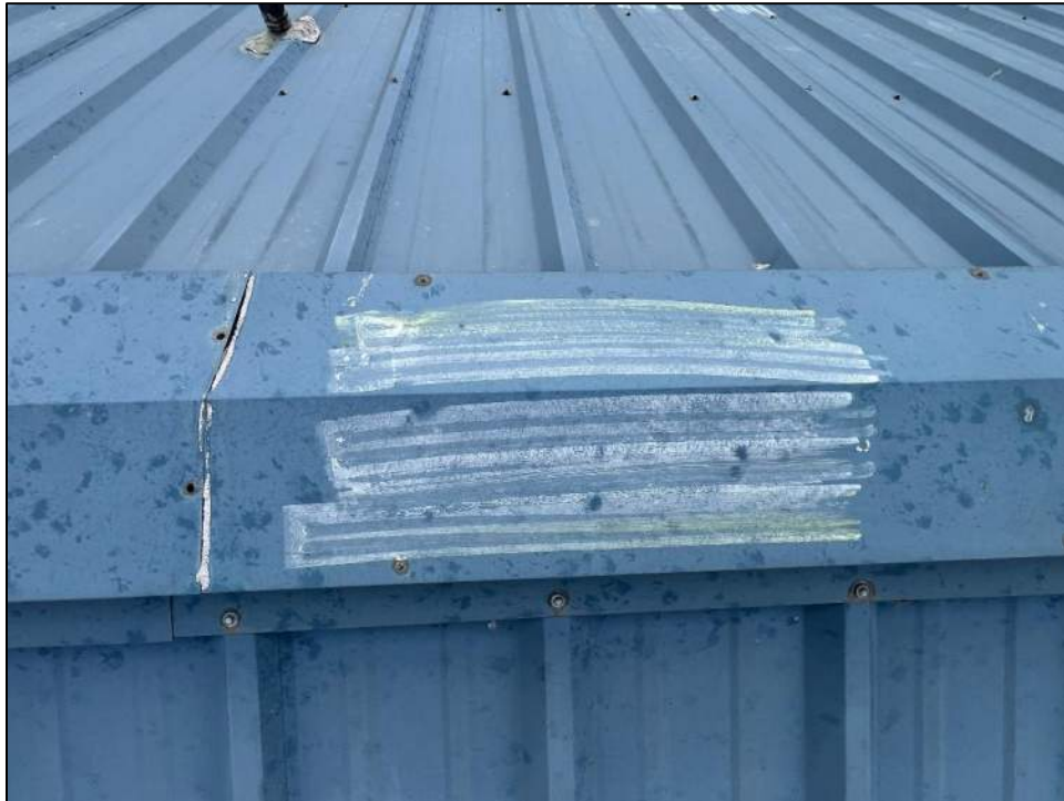
Photo 20: Hail-denting along ridge cap had maximum inner diameter of 1/2 inch.
