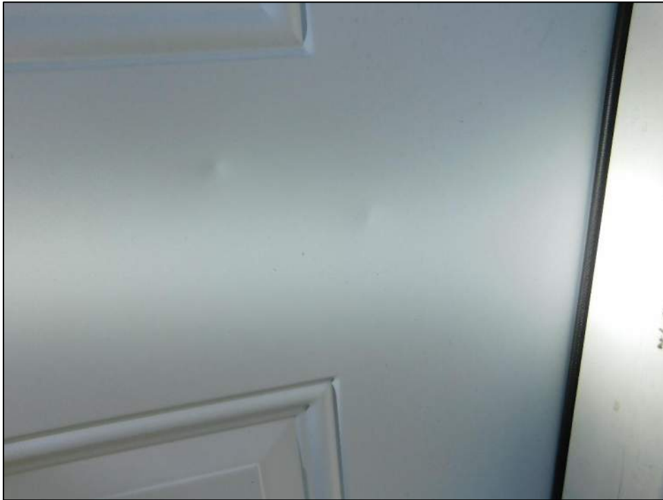
Photo 90: Closer view of the isolated denting on the front door consistent with hail impact.
