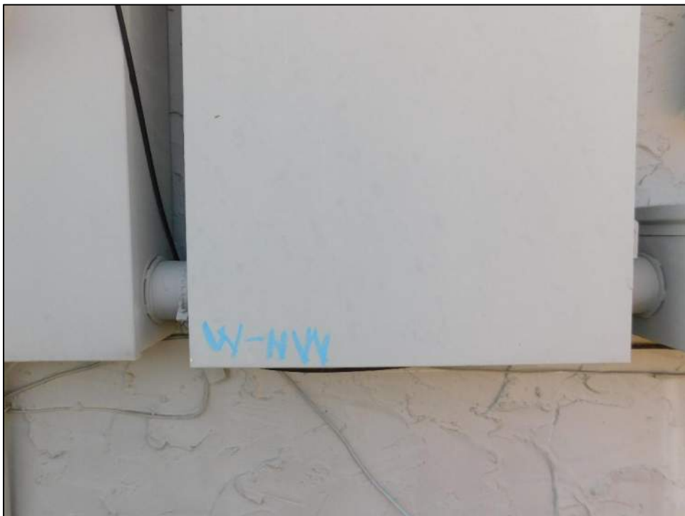
Photo 14: Slight hail spatters on west wall.
