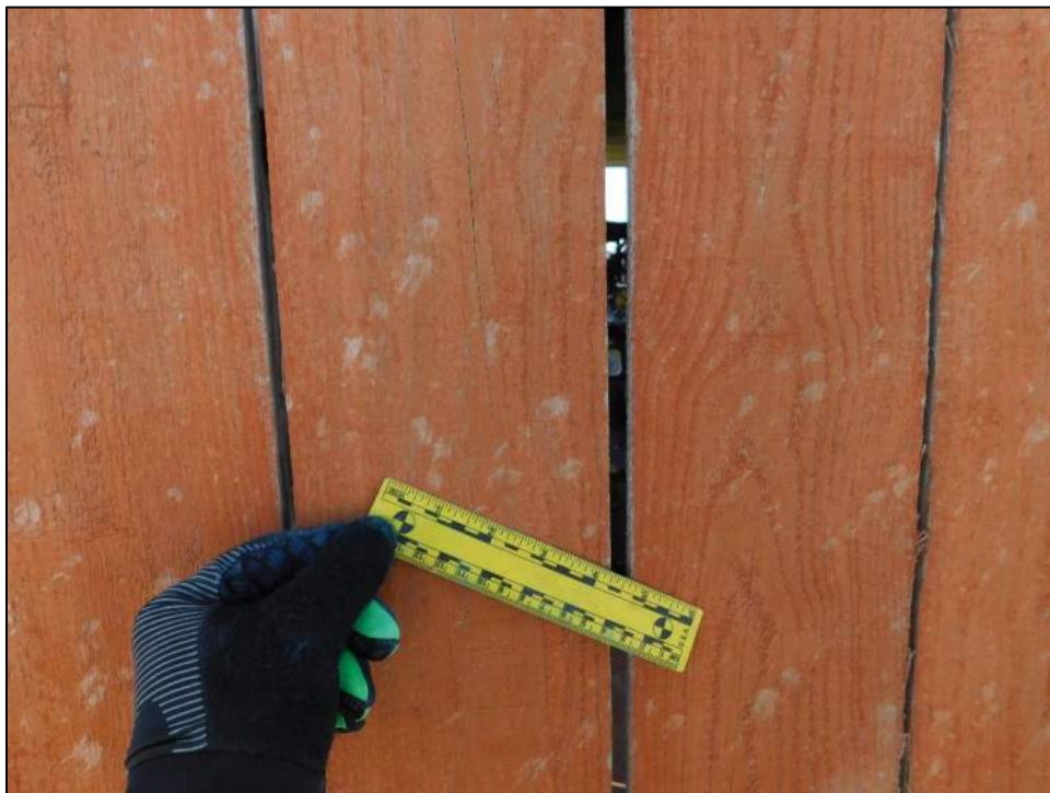
Photo 16: Hail spatters on wood-fence enclosing a dumpster reflected 1-inch hail at the site.
