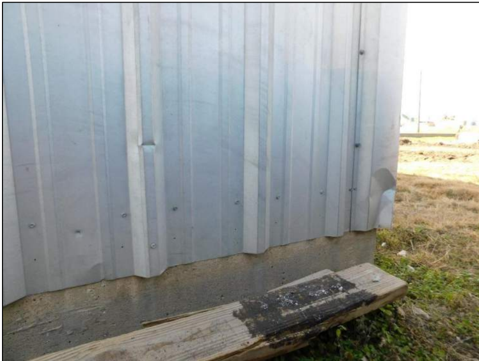
Photo 82: Mechanical damage at the bottom portion of the north wall unrelated to hail impact.
