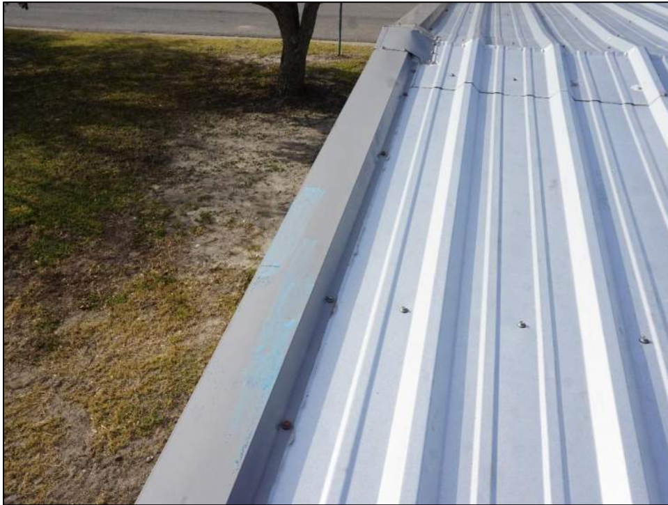
Photo 28: Edge enclosure metal along gable end rakes were dented but absent of coating disruptions.
