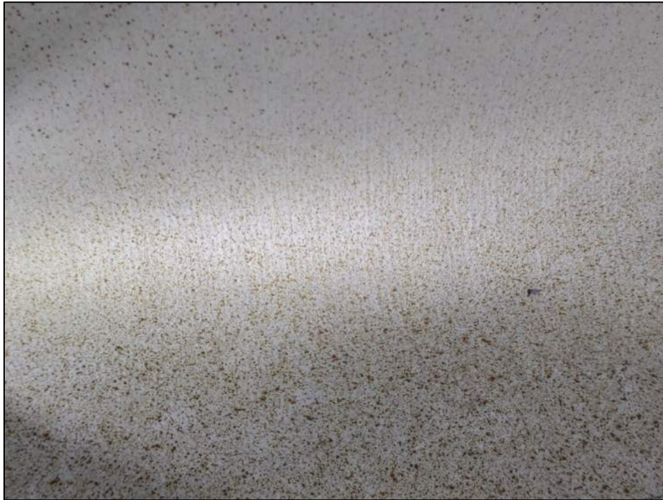
Photo 35: Unsupported PVC membranes at the base of parapets facing the direction of the hail were not punctured dimpled or scuffed.
