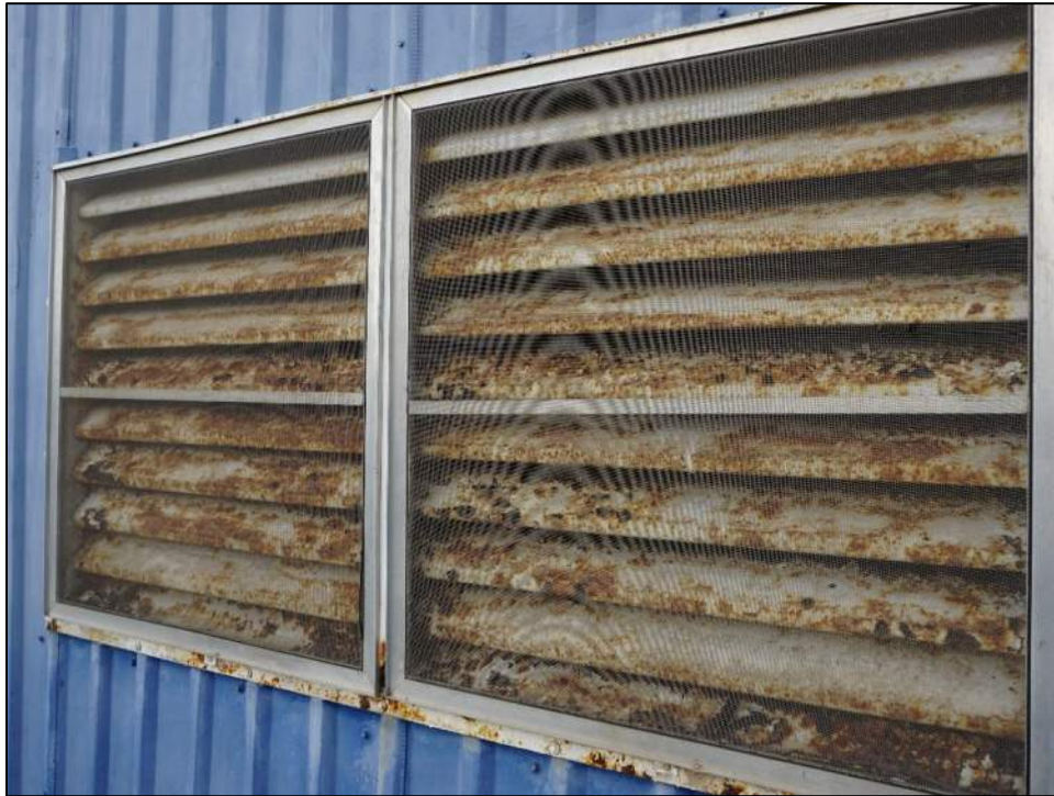
Photo 39: Severely corroded louvers on east elevation.
