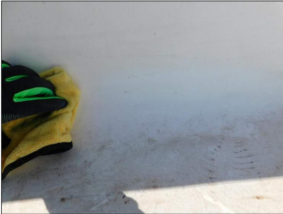
Photo 25: Unsupported PVC membranes at the base of parapets facing the direction of the hail were not punctured dimpled or scuffed.
