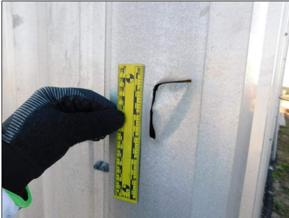
Photo 61: Mechanically punctured north wall.
