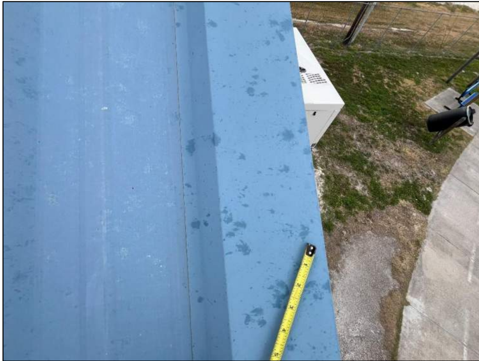
Photo 17: Largest hail spatter on west gable rake top surface reflected 1.25 inch hail.
