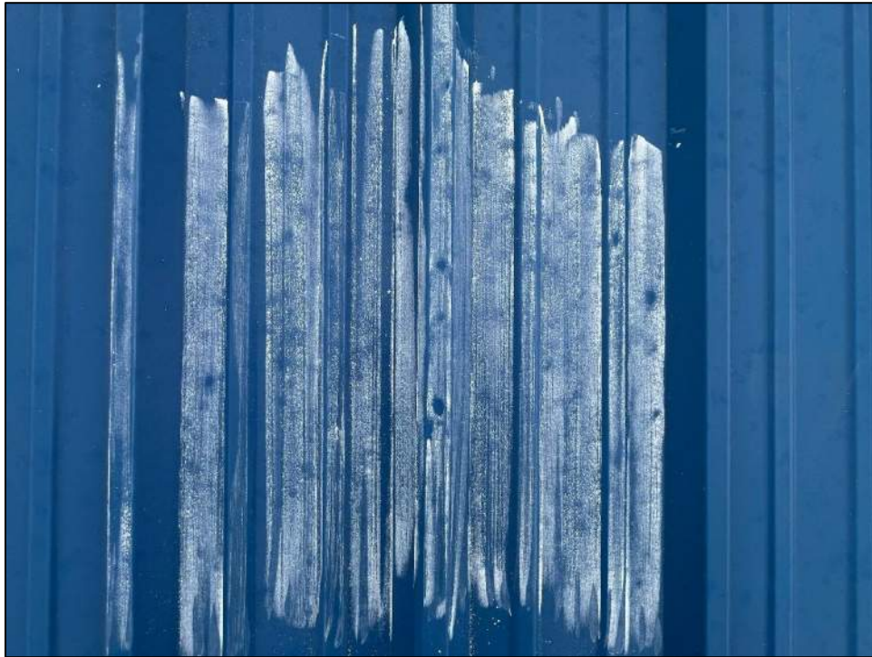
Photo 11: Close-up of the hail denting on north slope. No coating disruptions were observed.
