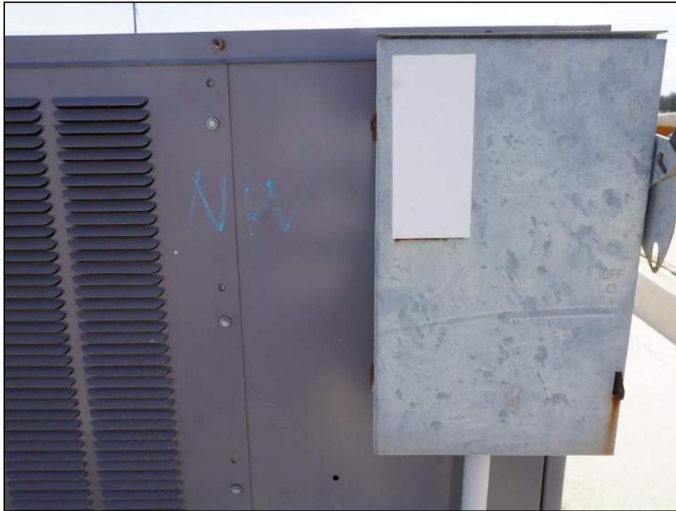
Photo 7: Hail spatters on rooftop units reflect 1-inch hail.
