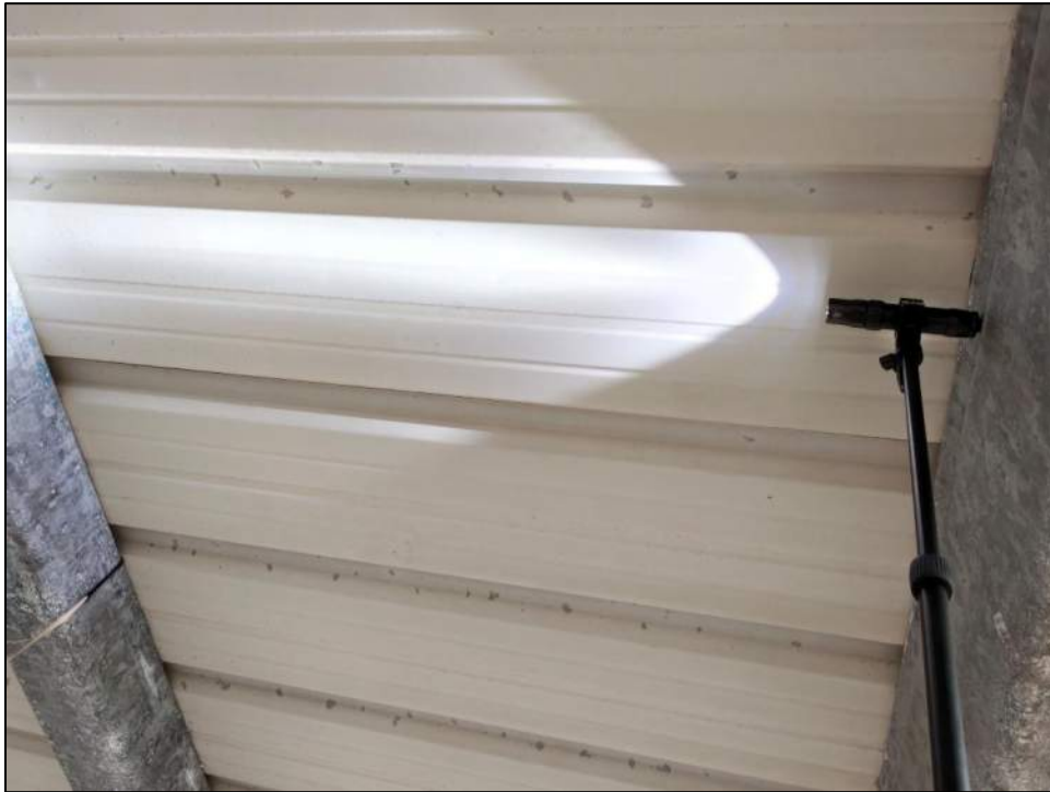
Photo 90: Denting to east slope were significantly less than west slope.
