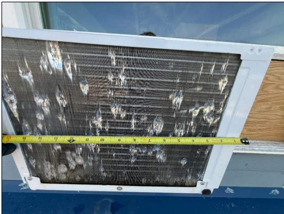
Photo 22: Largest hail dentings on the window AC coils directly facing the impact of hail were consistent with 1.5-inch-diameter hail.
