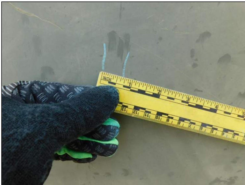
Photo 28: Hail spatters consistent with 0.75- to 1.0-inch hail on north-facing surfaces.
