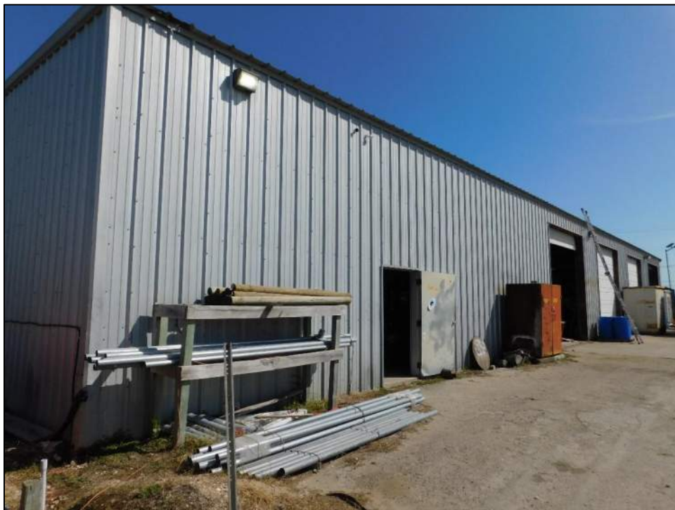
Photo 53: Front wall panels were not dented.
