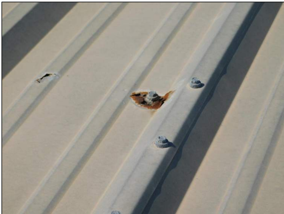
Photo 90: Corroded roof deck at fasteners.
