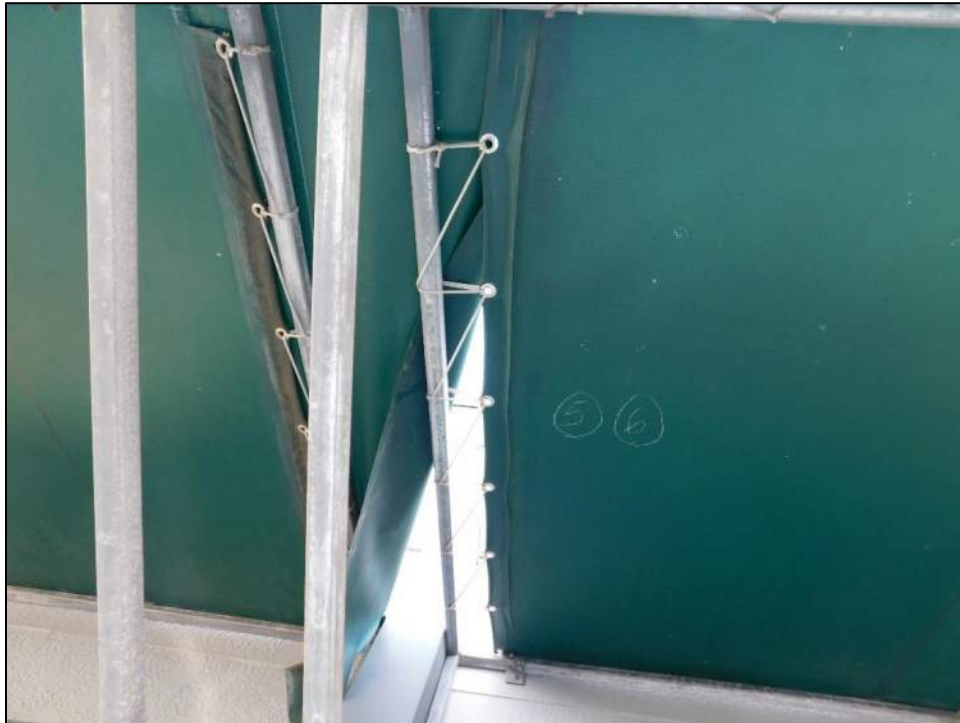
Photo 11: Impact fractures consistent with hail impact observed on the PVC coated awning along the north and east walls.
