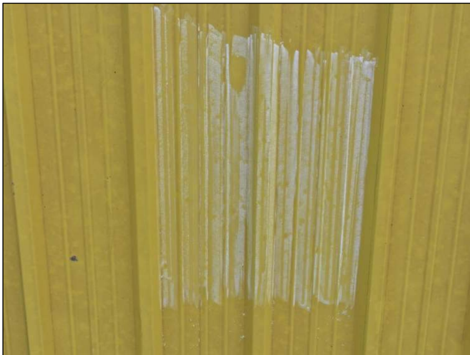
Photo 81: Denting consistent with hail impact was observed. No coating disruptions were observed at the dents.
