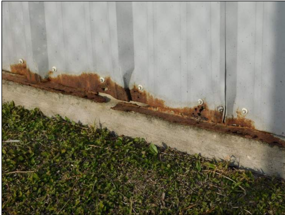
Photo 9: Corrosion along the bottom of the east wall.
