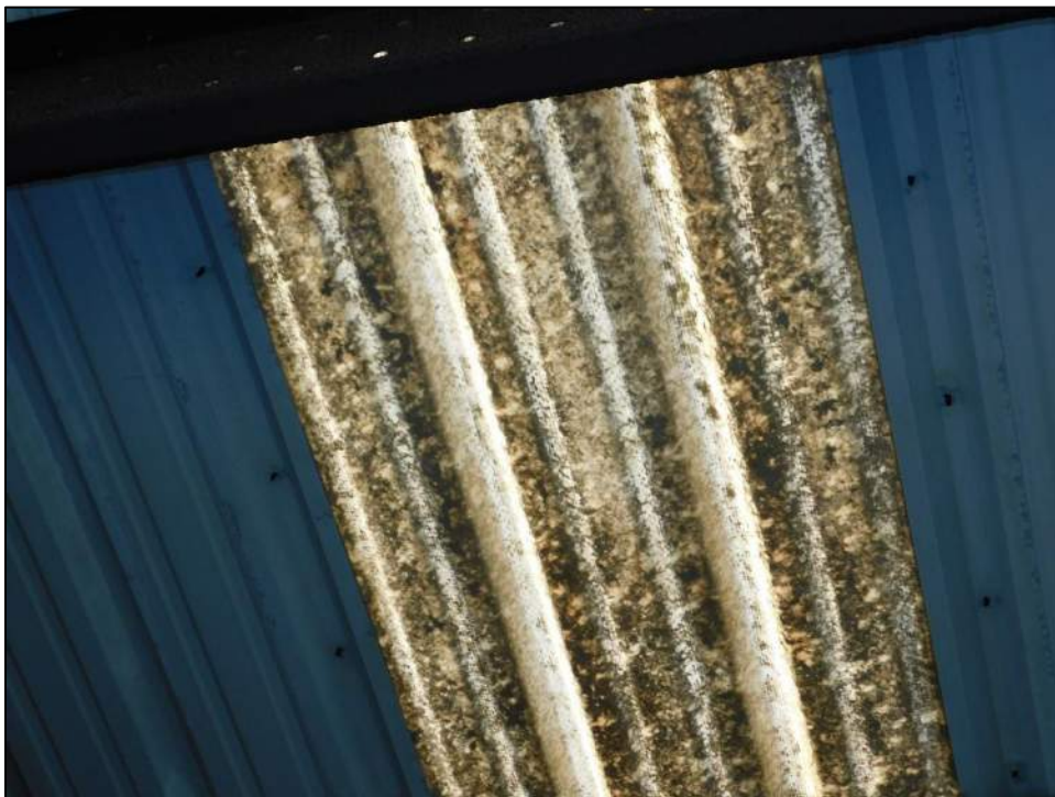
Photo 26: No discernible hail impact fracture was observed in the skylight panels.
