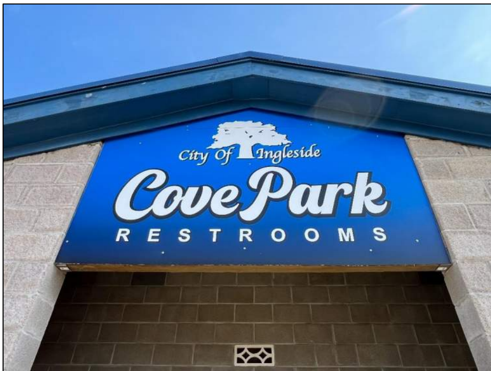
Photo 2: Signs above restroom entry exhibited no hail impact scuff marks.
