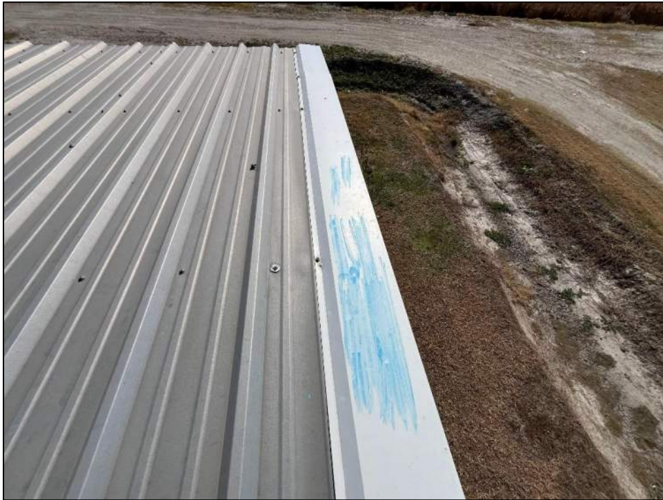
Photo 21: Hail denting identified on closure trim along south rake.
