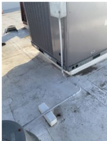
Photo Documentation 33 Electrical lines in PVC
